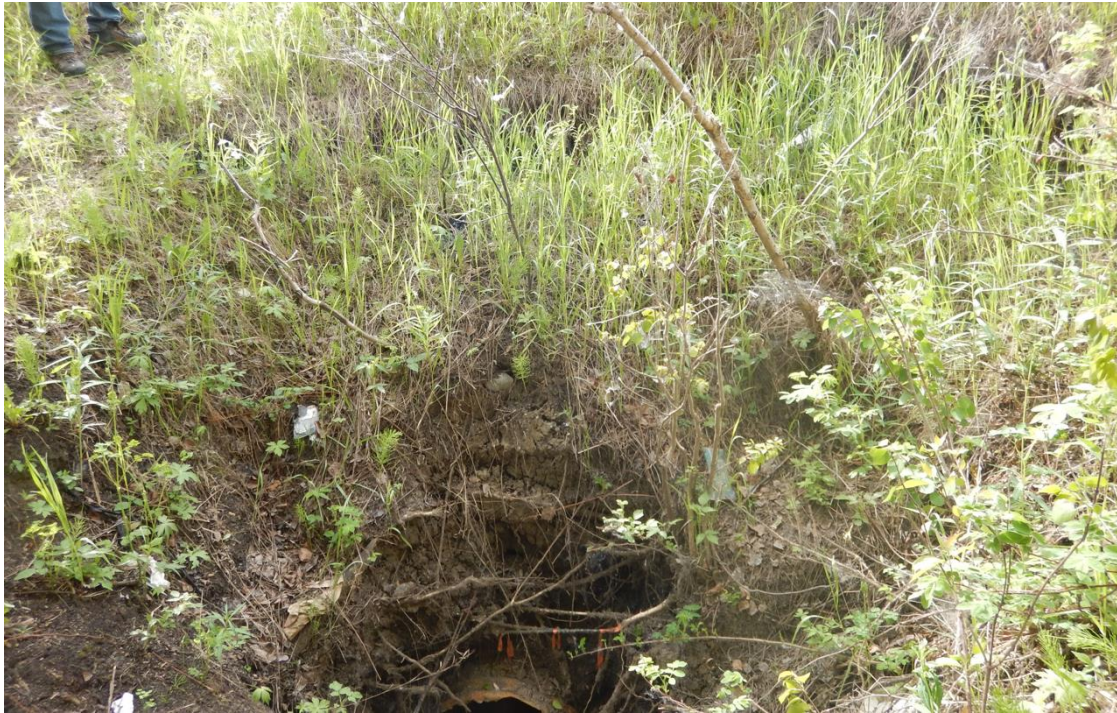
Photo No. 3 – Scarp crack above the culvert inlet (400 mm wide, 600 mm drop)
