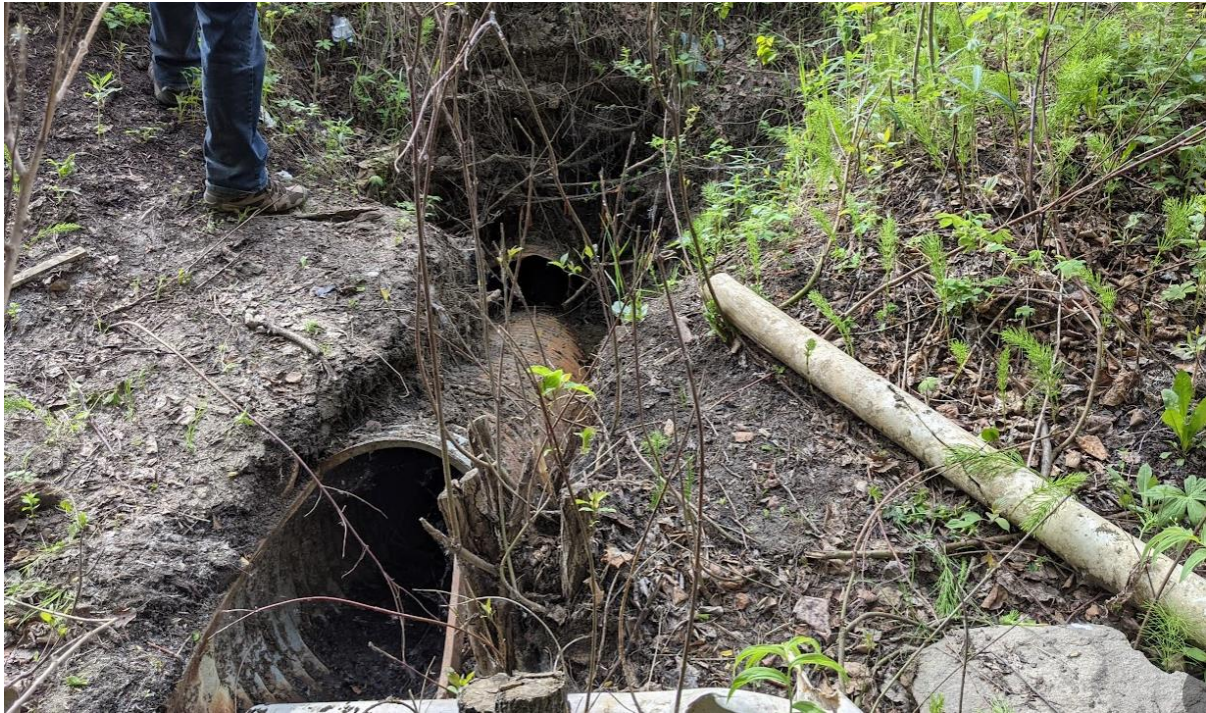
Photo No. 1 – 600 mm CSP culvert separated at 3 m from inlet. Note sinkhole developed above culvert separation
