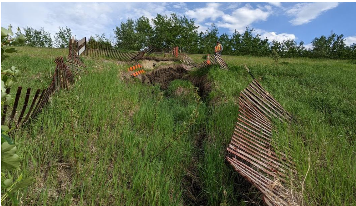
Photo No. 4 – Looking east at the head scarp crack of the slump. Slump area approximately is 1.4 m wider on each flank.
