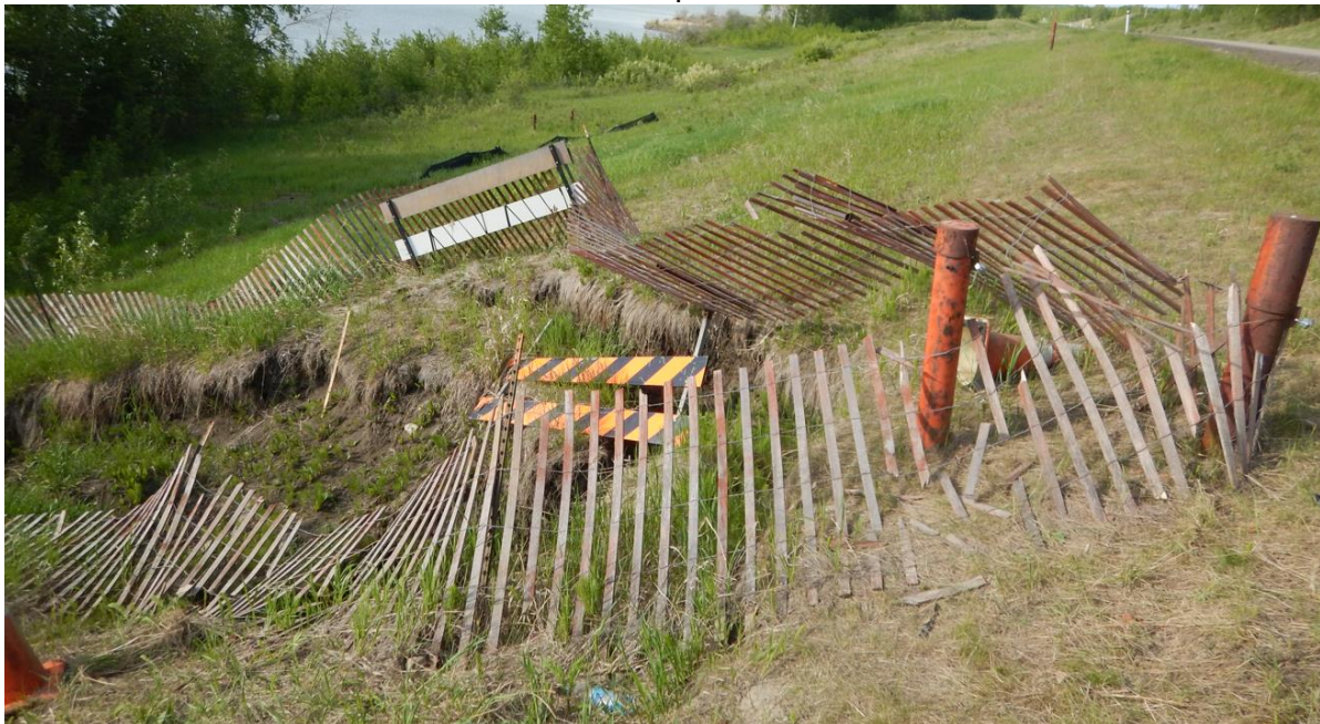
Photo No. 2 – Looking northeast at the observed slump downslope of the pile wall location. Snow fence collapsed due to ongoing movement of the slump.
