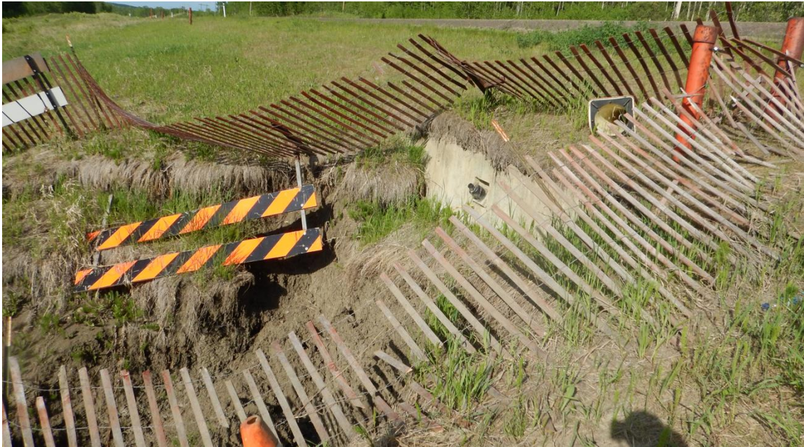
Photo No. 5 – Looking at the northeast flank of the slump; the slump exposed a 5 m long section of the concrete water
