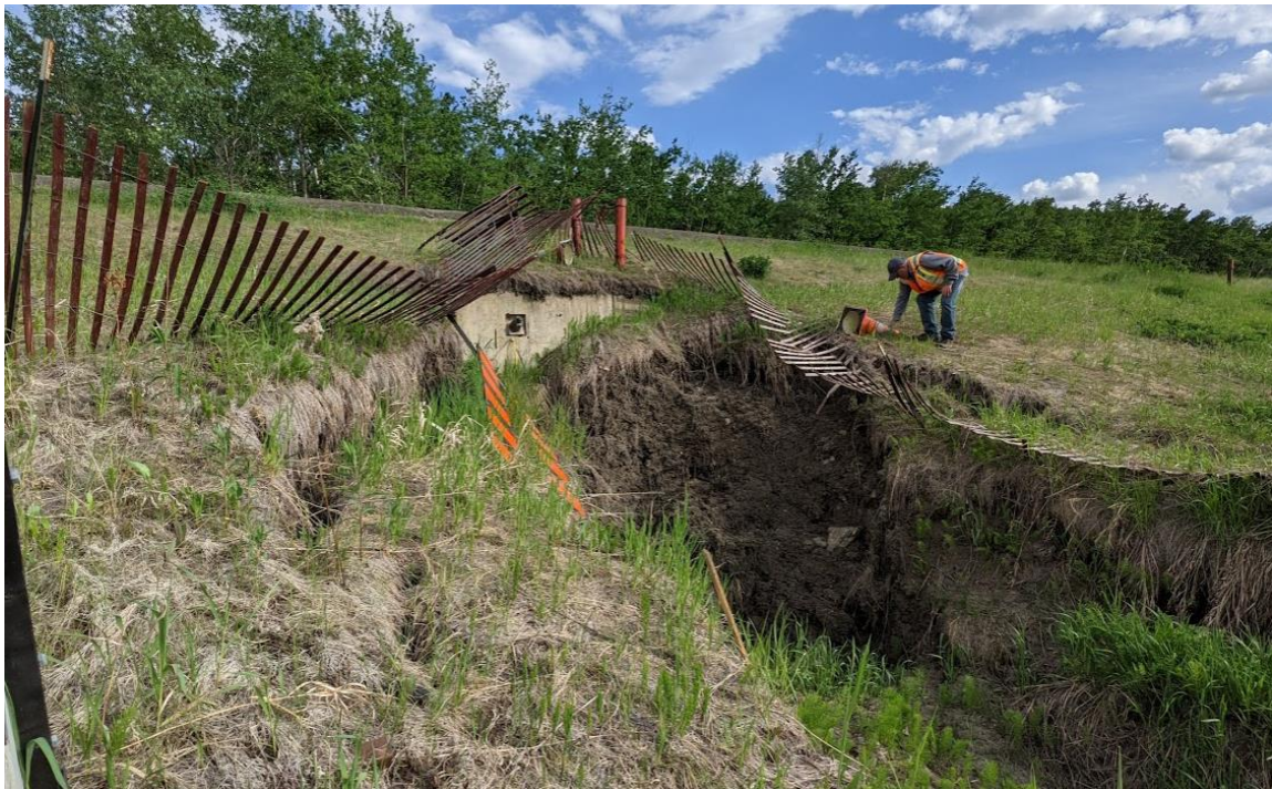
Phot No. 6 – Looking at southeast flank of the slump
