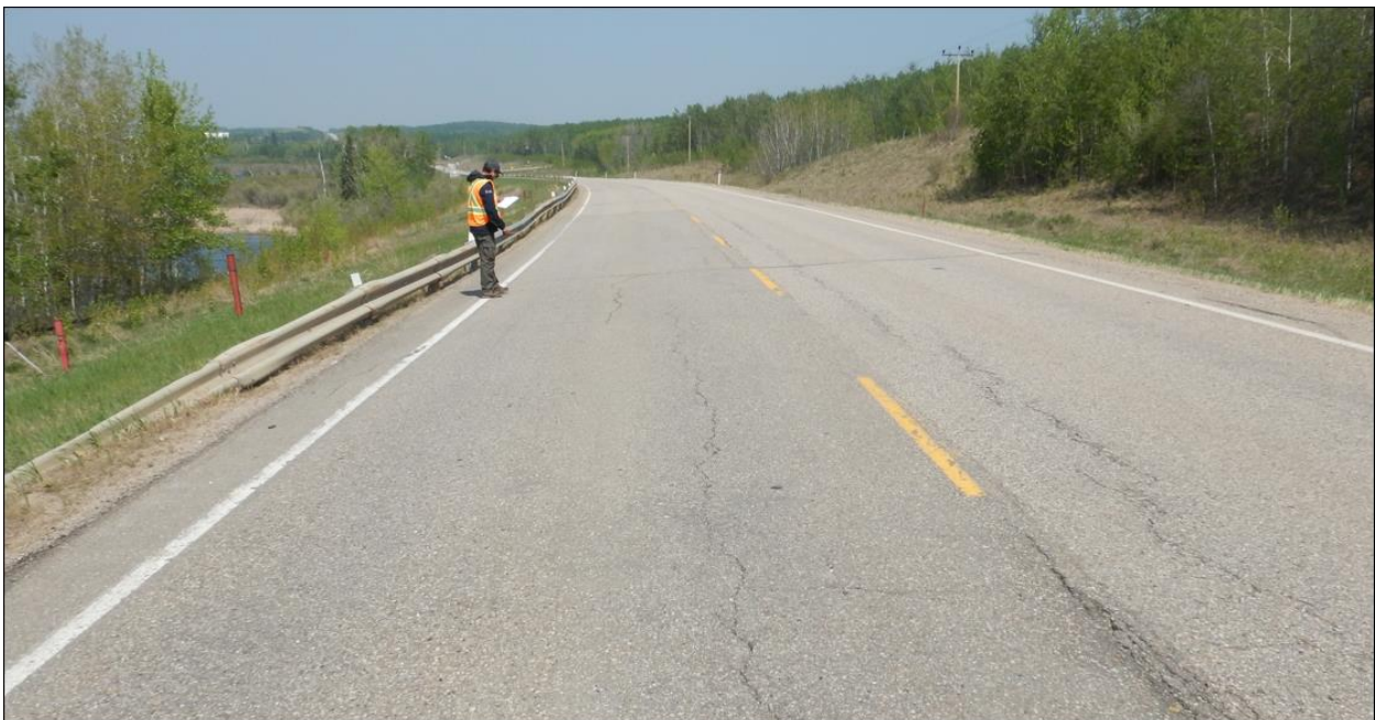
Photo No.2 - Looking north at up to 20 mm wide reflective cracks, no drop on the SBL at the NC24D pile wall location
