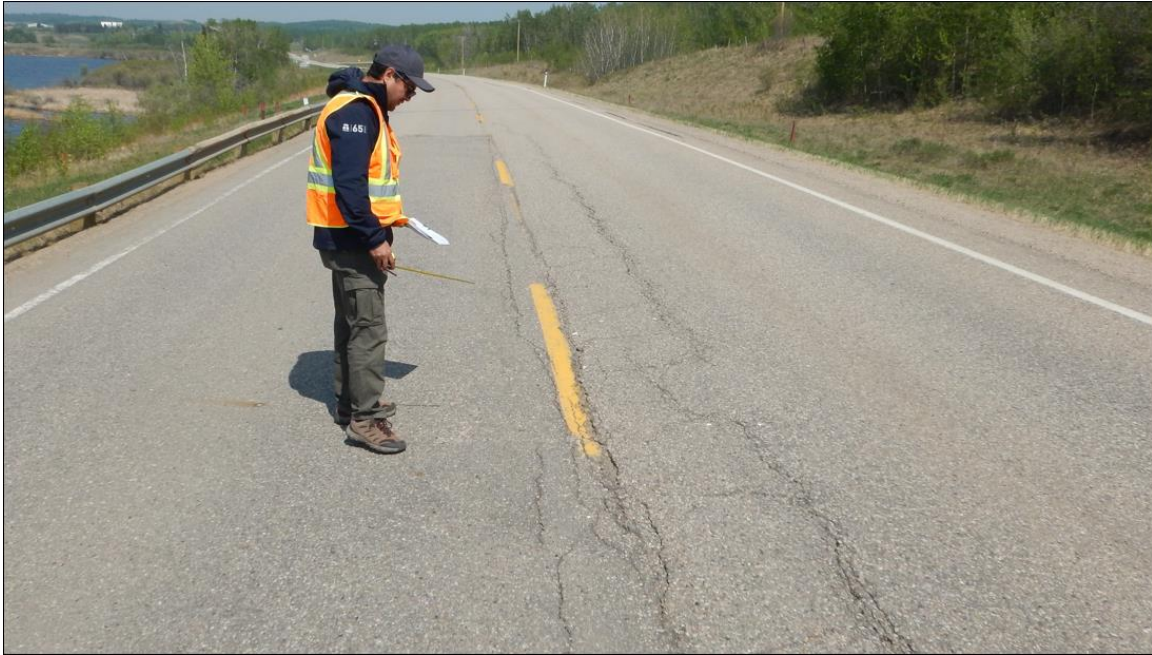
Photo No.3 - Looking north at up to 30 to 40 mm wide reflective cracks on the highway surface at the NC24D pile wall location
