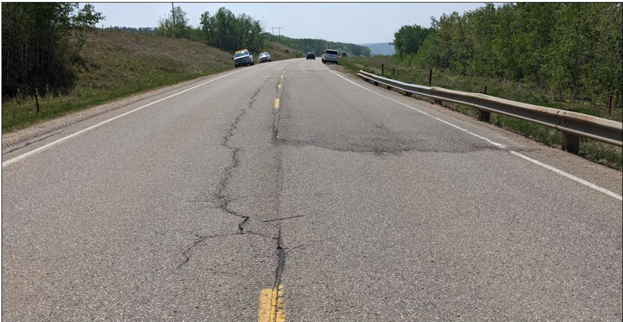
Photo No.4 - Looking south at longitudinal open cracks (10 to 40 mm wide) on the highway at the NC24D pile wall location
