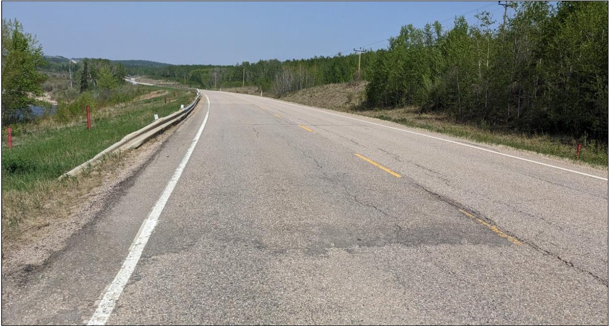
Photo No.1 - Looking north at the 2017 ACP patch placed on the highway surface at the NC24D pile wall location; no visible dip on highway surface.
