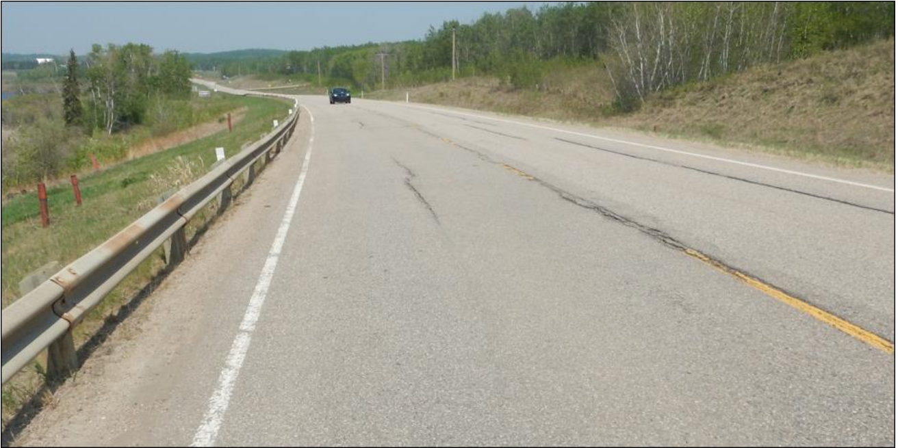
Photo No. 5 – Looking north at a reflective crack (60 mm wide with 5 mm drop) on the highway surface above NC24B pile wall location
