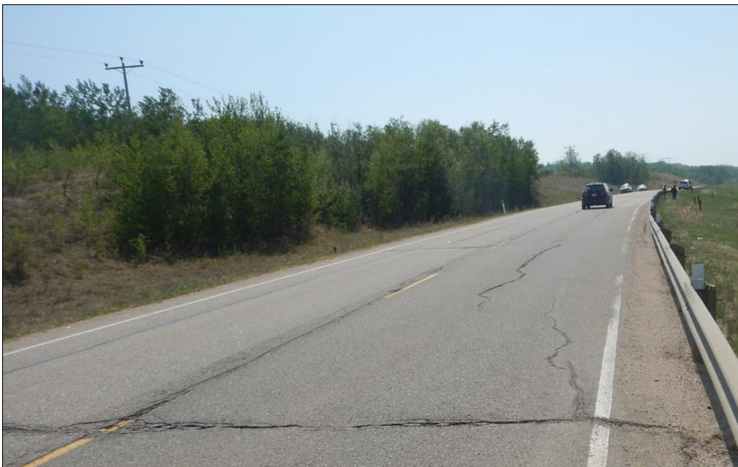
Photo No. 6 – Looking south from the northern flank of the NC24B landslide location at open reflective cracks (30 to 100 mm wide with 5 mm drop)
