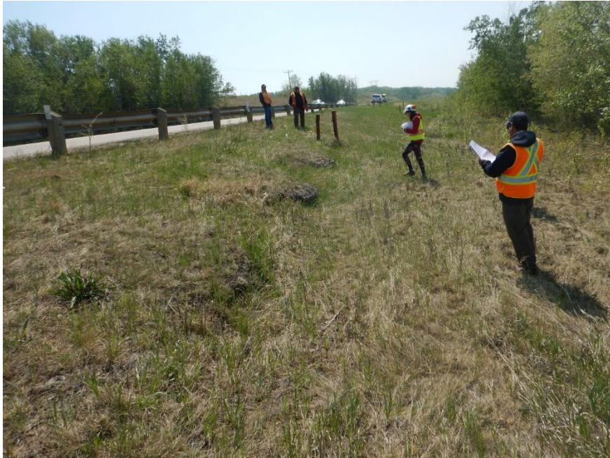
Photo No. 7 – Looking south at a minor slump developed immediately downslope of the NC24B pile wall; the slump exposed the tops of four concrete piles.
