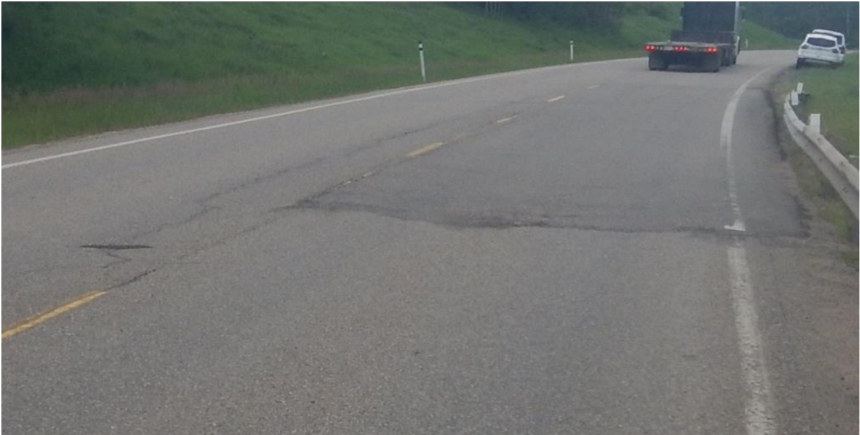
Photo No.4 - Looking south at longitudinal open cracks (10 to 40 mm wide) on the highway at the NC24D pile wall location
