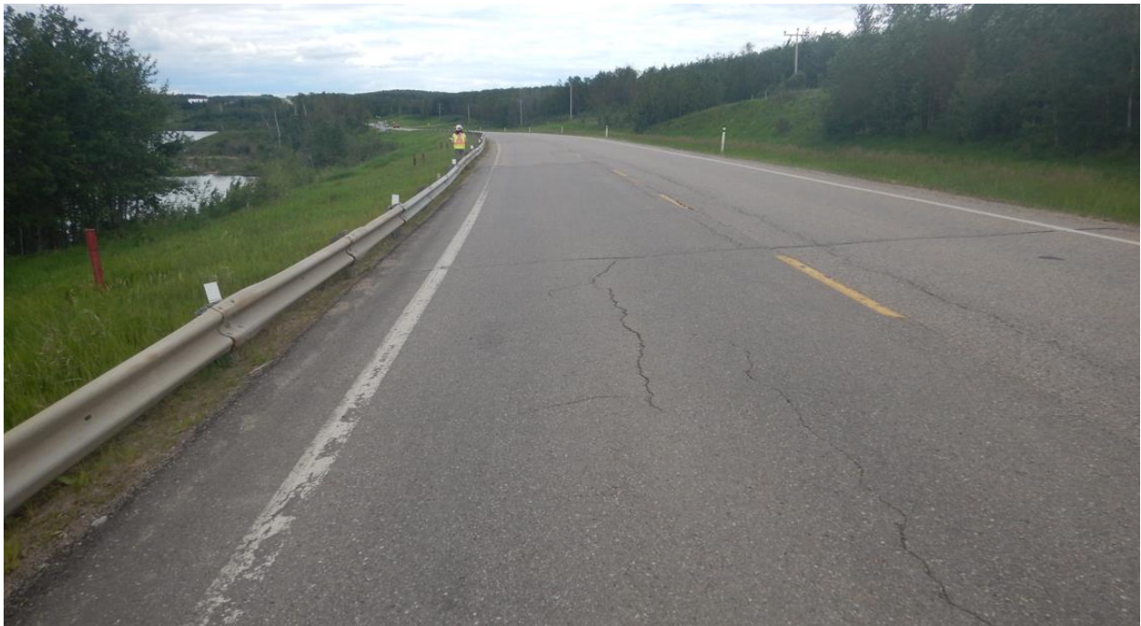
Photo No.2 - Looking north at up to 20 mm wide reflective cracks, no drop on the SBL at the NC24D pile wall location
