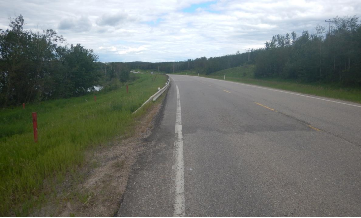
Photo No.1 - Looking north at the 2017 ACP patch placed on the highway surface at the NC24D pile wall location; no visible dip on highway surface
