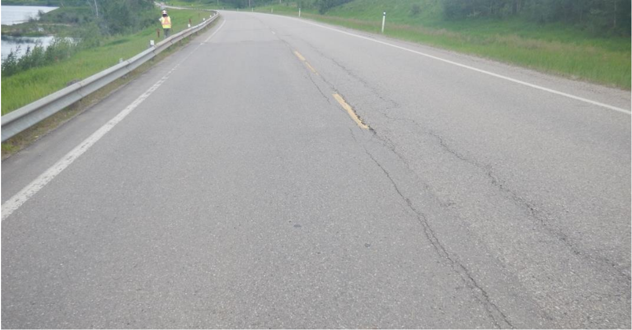
Photo No.3 - Looking north at up to 30 to 40 mm wide reflective cracks on the highway surface at the NC24D pile wall location
