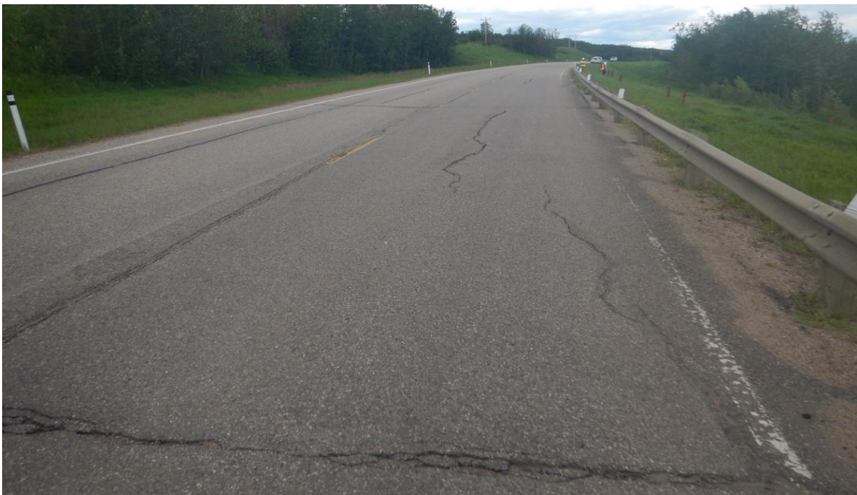
Photo No. 6 – Looking south from the northern flank of the NC24B landslide location at open reflective cracks (20 to 50 mm wide with no drop)
