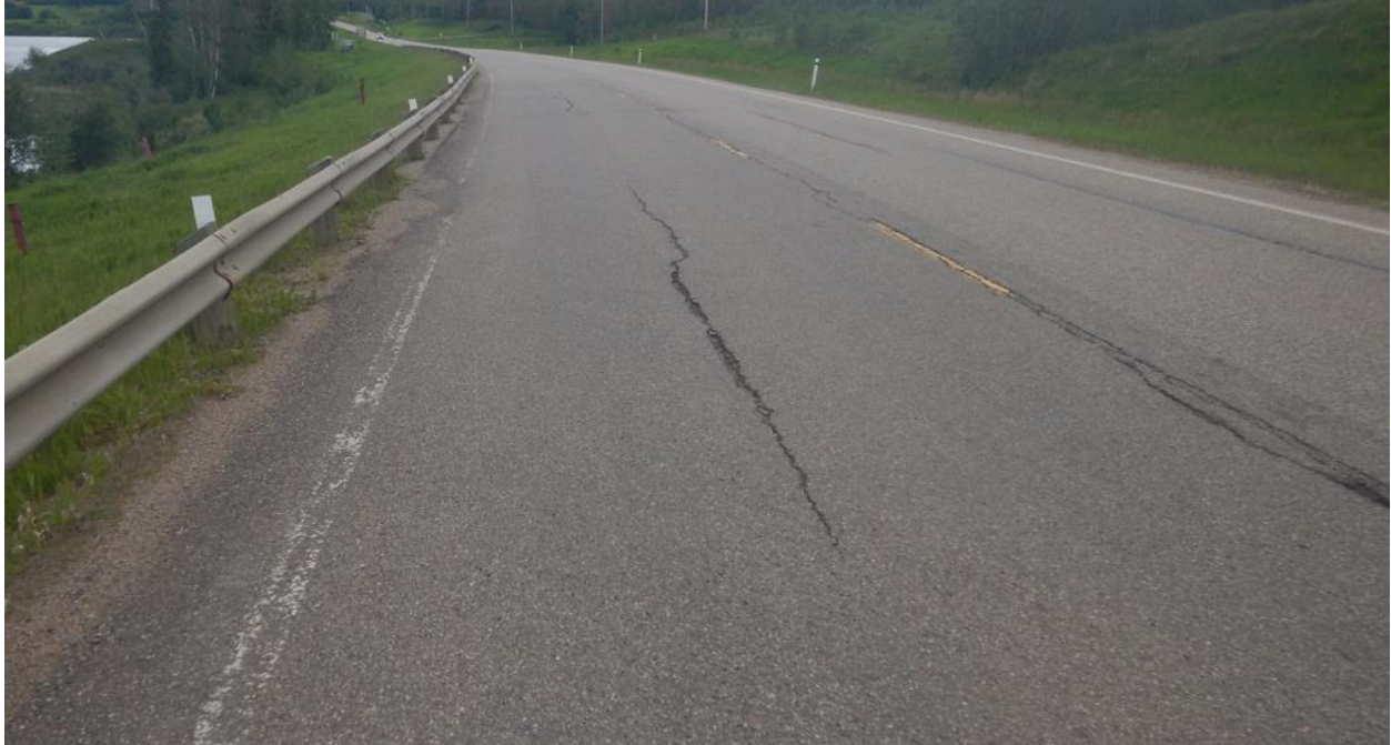
Photo No. 5 – Looking north at 11 m long x 50 mm wide reflective crack on the highway at the NC24B pile wall location
