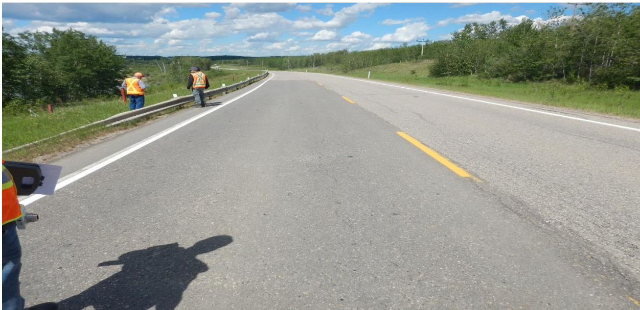
Photo No.2 - Looking north at up to 10 mm wide reflective crack on the SBL at NC24D location
