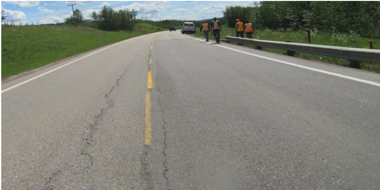
Photo No.3 - Looking south at reflective longitudinal open cracks (10 to 20 mm wide) at NC24D location
