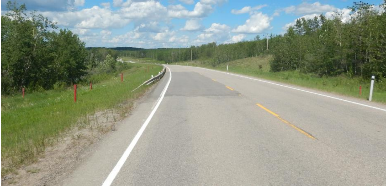
Photo No.1 - Looking north at the 2017 ACP patch placed at NC24D location; no visible dip on highway surface
