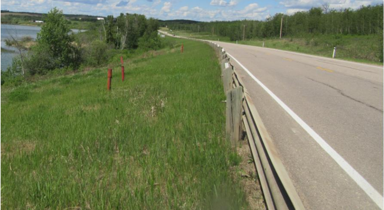
Photo No.4 - Looking north at the highway side slope downslope at NC24D location; no signs of cracking or bulging noted on the side slope
