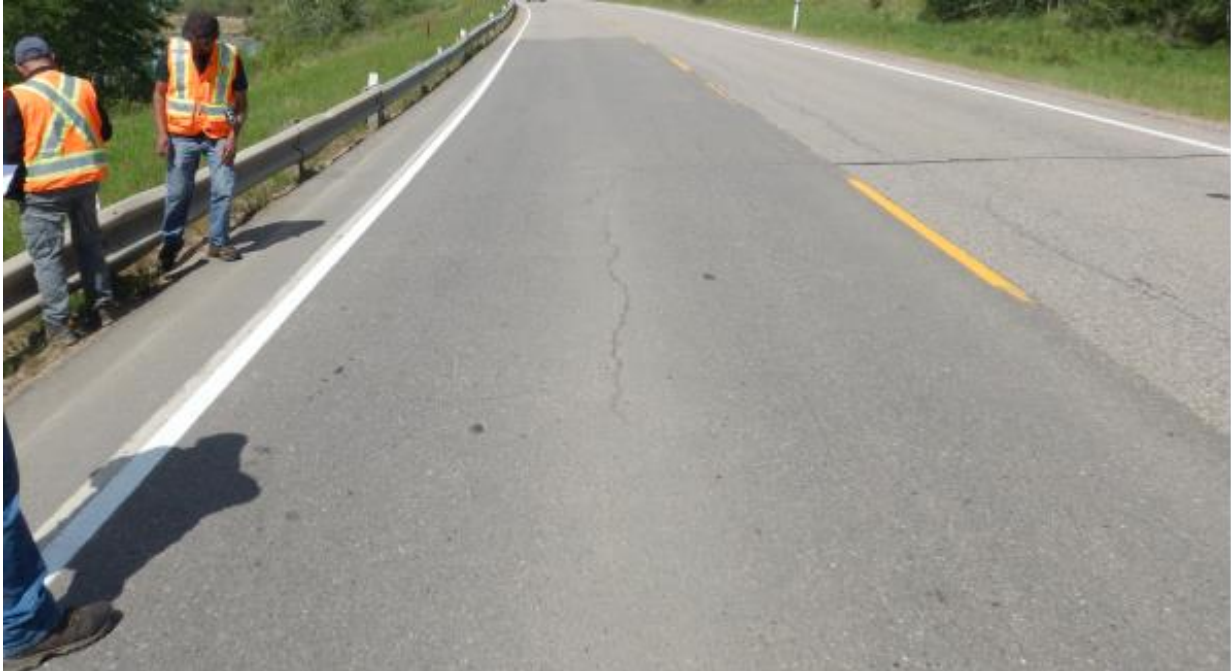
Photo No.2A - Looking north at up to 10 mm wide reflective crack on the SBL at NC24D location
