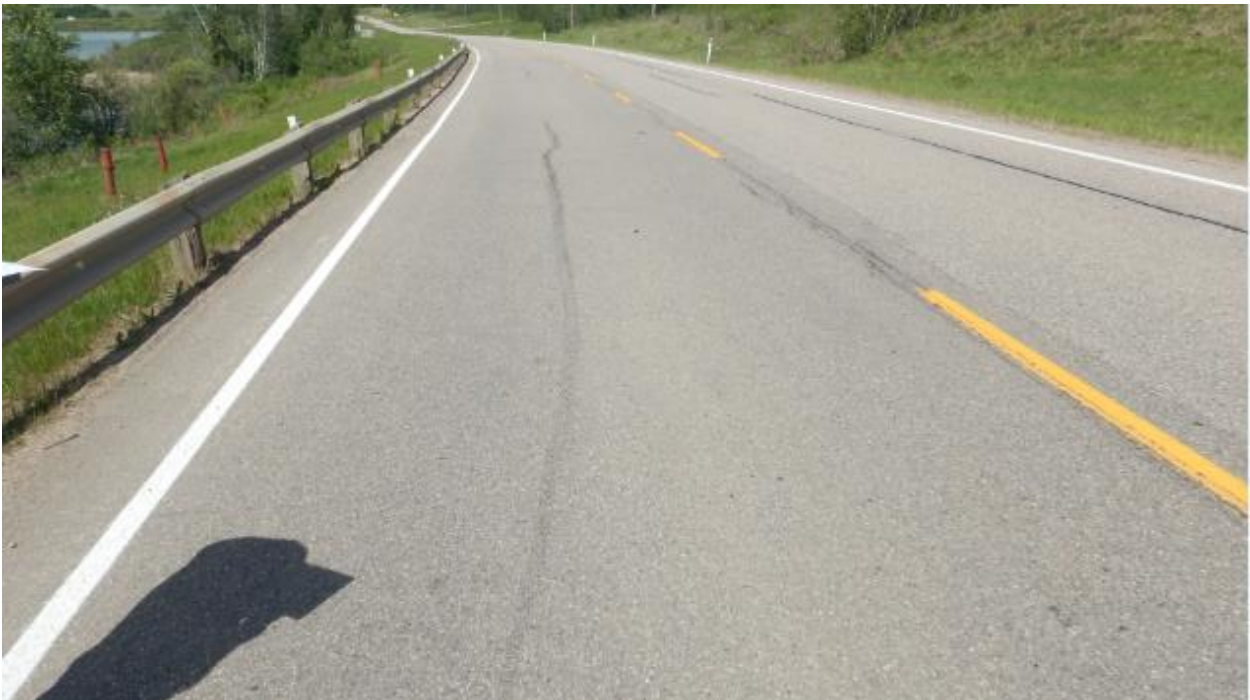
Photo No. 5 – Reflective cracks along the highway above NC24 B Pile Wall
