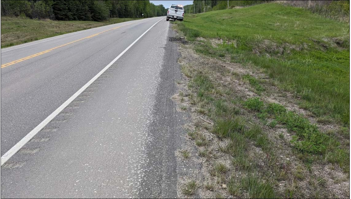
Photo No. 1 – Looking west at highway surface at the landslide location. Highway was overlaid in 2022
