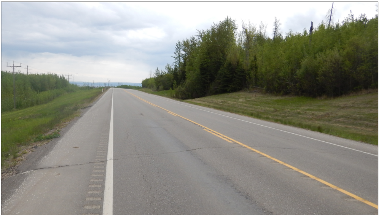
Photo No. 2 – Looking east at transverse and longitudinal reflective cracks on the highway surface at the landslide location
