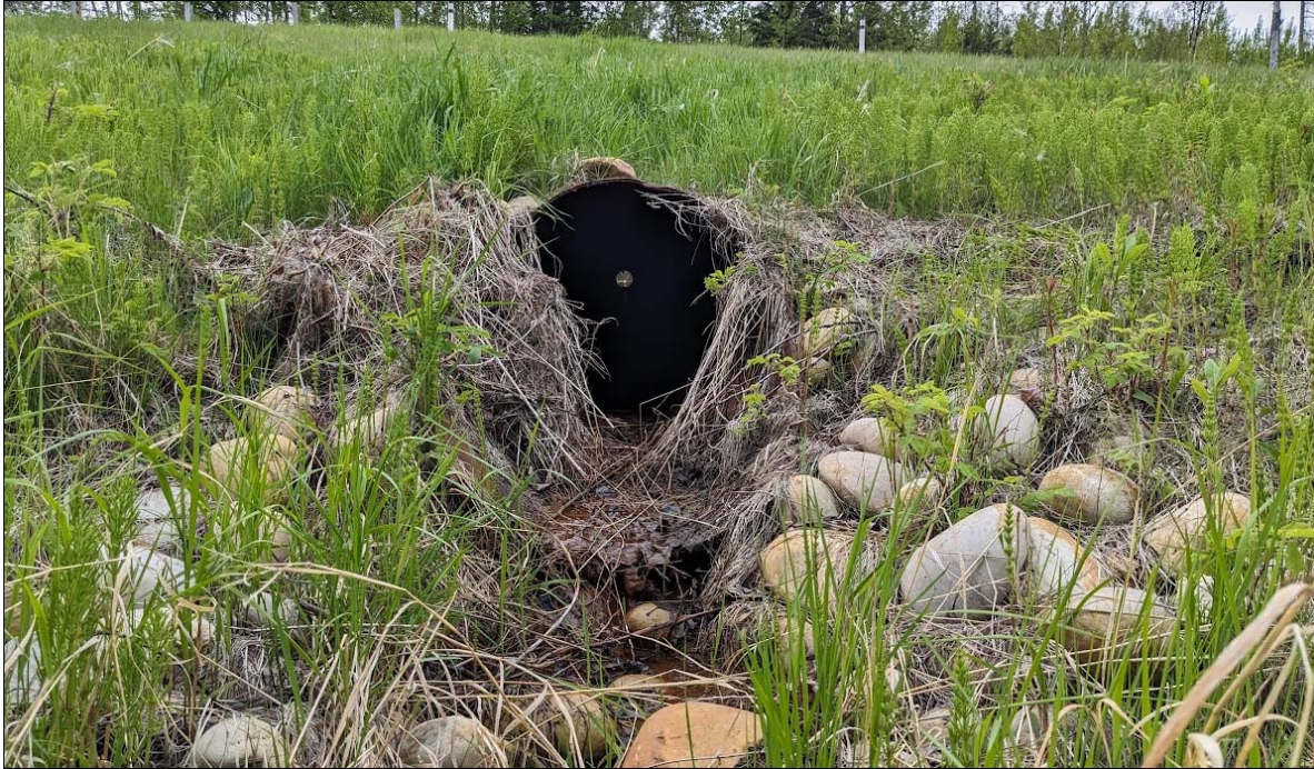
Photo No. 9 – Looking south at the outlet of the 600 mm diameter SWSP culvert
