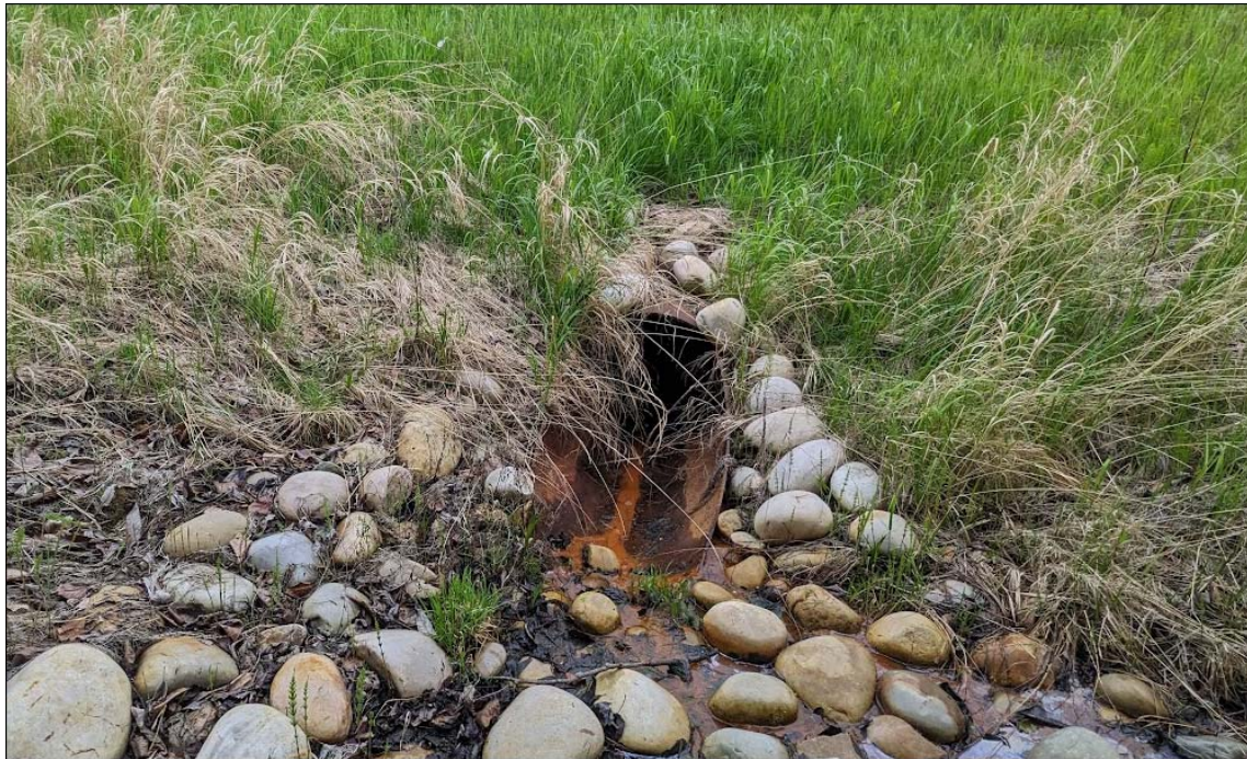
Photo No. 8 – Looking northeast at the inlet of the 600 mm diameter SWSP culvert
