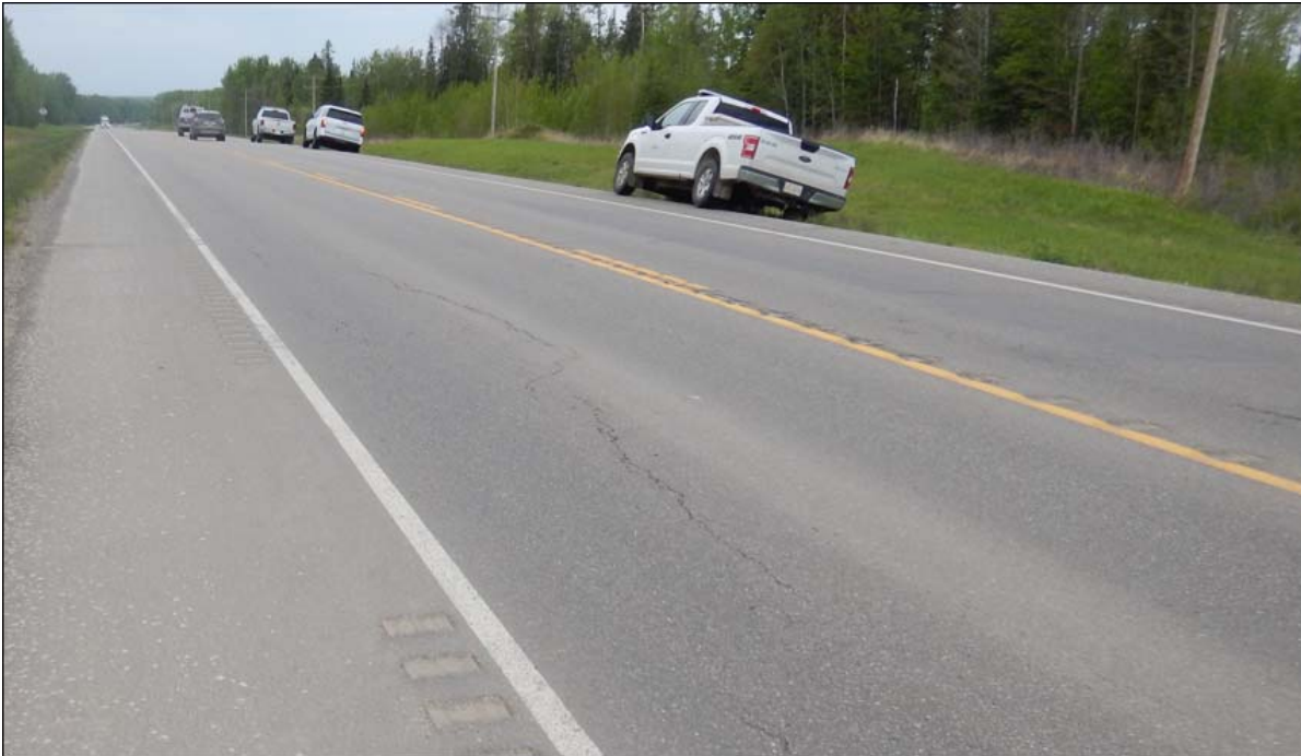
Photo No. 3 – Looking west at a 5 to 10 mm wide longitudinal crack on the highway surface
