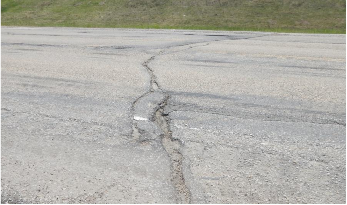
Photo No.3 – Looking north at a 60 to 130 mm wide transverse crack on the highway surface to the east of the landslide location; Pothole is 1 m long, 260 mm wide, 30 mm deep
