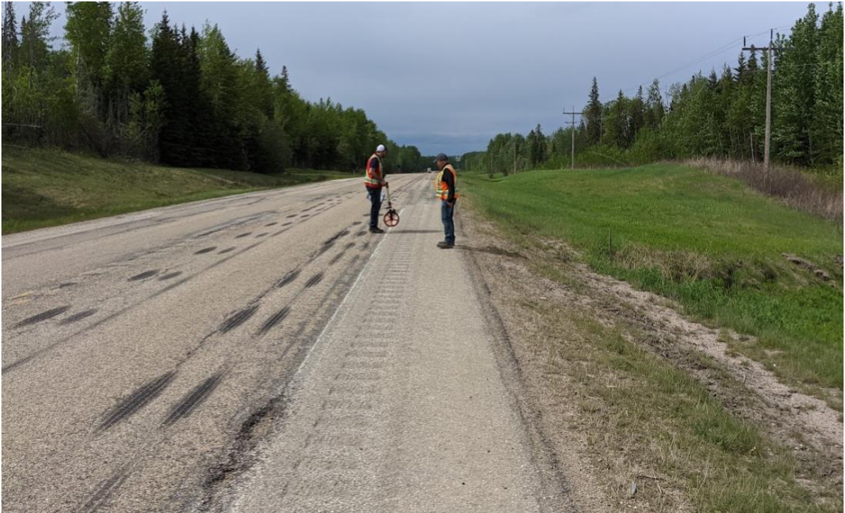
Photo No.1 – Looking west at longitudinal cracks on the highway surface at the landslide location
