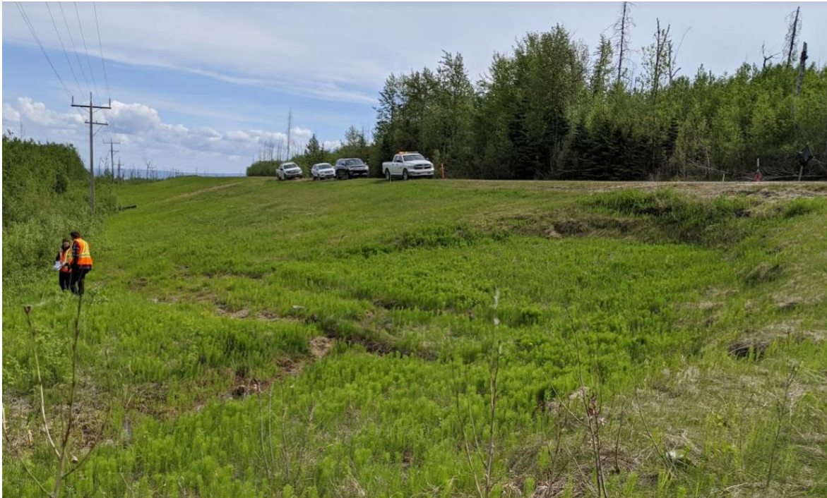
Photo No.5 – Looking southeast at the head scarp crack of landslide mass; a distinct toe roll was noted at the bottom of the slope; more vegetation grew within the landslide mass
