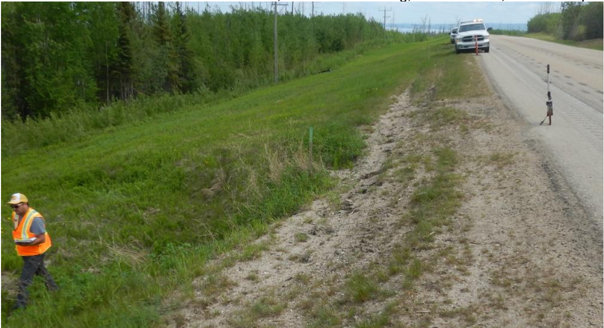
Photo No.4 – Looking east at the landslide developed on the highway side slope; head scarp crack measured at 4.4 m from the white line (same as measured in 2020)
