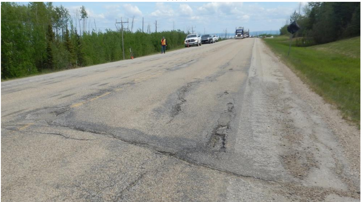
Photo No.2 – Looking east at transverse and longitudinal cracks on the highway surface at the landslide location; wide open cracks are more pronounced within the highway EBL
