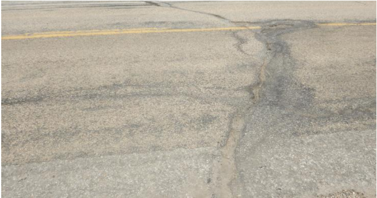
Photo No.3 – Looking north at a 50 to 130 mm wide transverse crack on the highway surface to the east of the landslide location
