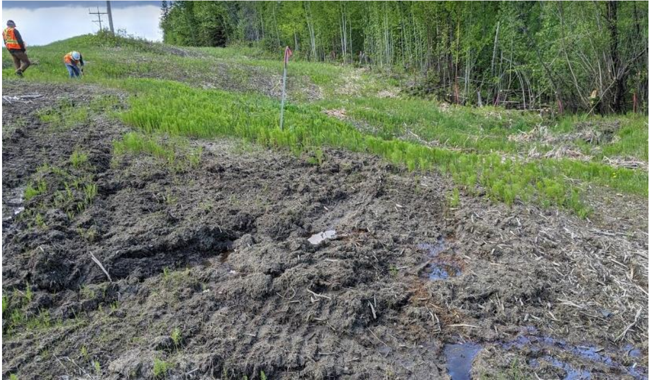
Photo No.7 – Looking north at the landslide toe roll; note the presence of seepage and Telus pedestal near the bottom of the slope
