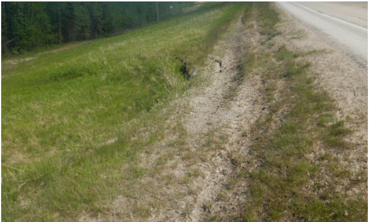
Photo No.4 – Looking east at the landslide developed on the highway side slope; note the retrogression of the landslide head scarp crack towards the highway
