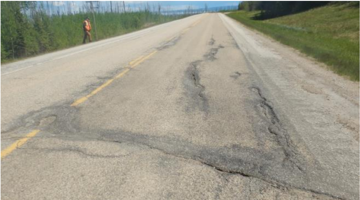
Photo No.2 – Looking east at transverse and longitudinal cracks on the highway surface at the landslide location; wide open cracks are more pronounced within the highway EBL
