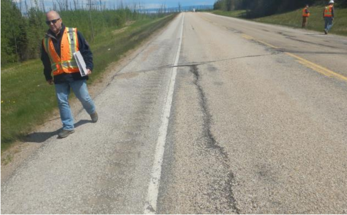
Photo No.1 – Looking east at a longitudinal crack on the highway WBL to the east of the landslide location
