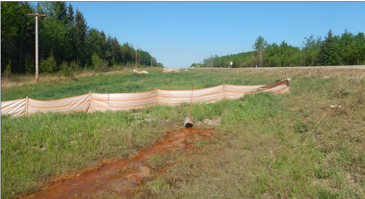
Photo # 8 Looking west at the outlet of the 200 mm diameter CSP subdrain pipe; reddish-brown stained water was flowing from the pipe and silt accumulated within the bottom of the pipe (approximately 50 mm in thickness; 25 percent of pipe diameter)
