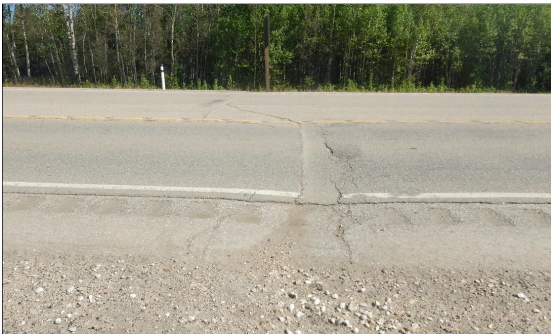
Photo # 6 Looking north at Crack C; 10 to 50 mm wide and 15 mm drop
