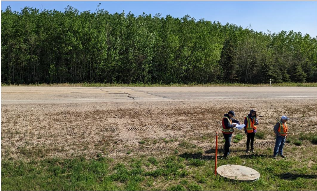
Photo # 3 Looking north at highway side slope and the 1.2 m CSP Manhole. The manhole lid was bent and could not be opened; accumulated sediment around the manhole
