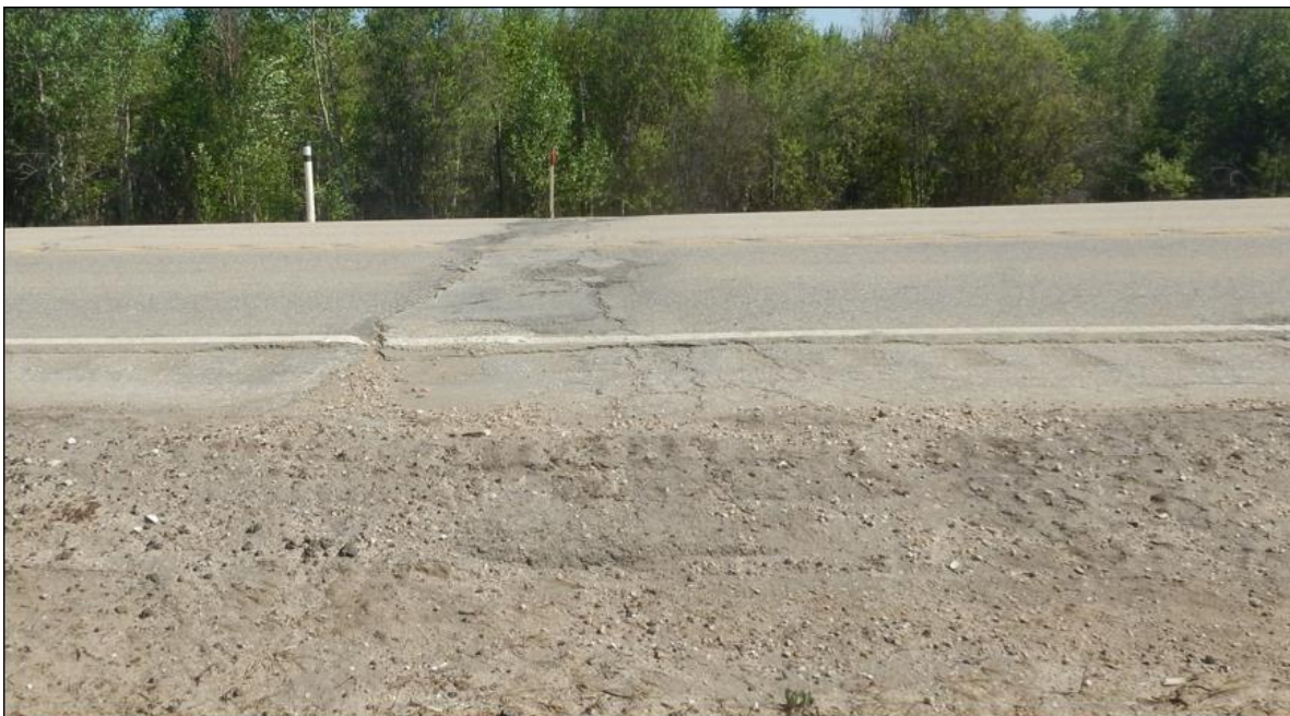
Photo # 4 Looking north at the bump crack (Crack A); 20 to 30 mm wide and 20 mm drop
