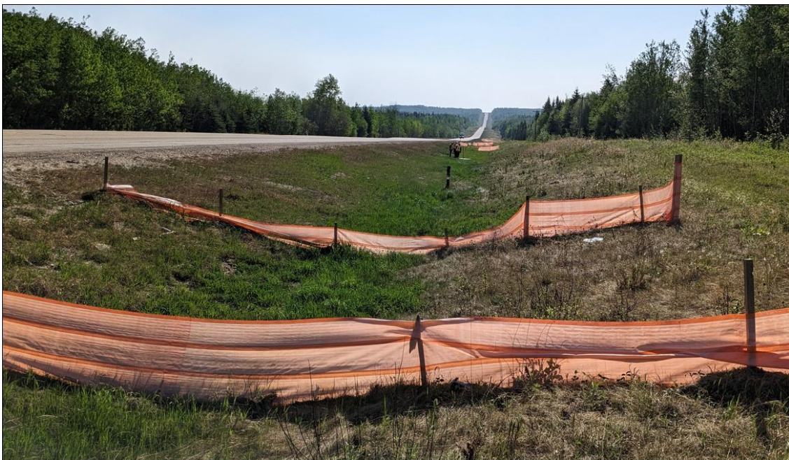
Photo # 2 Looking east at south ditch from the western limit of the site; falling silt fencing
