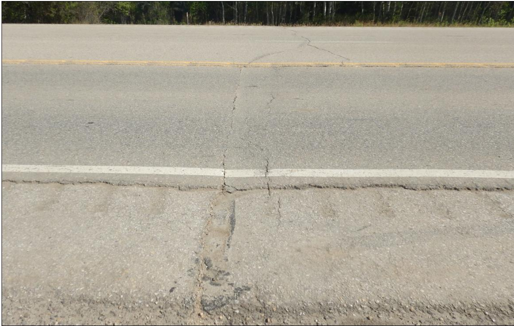
Photo # 5 Looking north at Crack B; 10 to 20 mm wide and 10 mm drop
