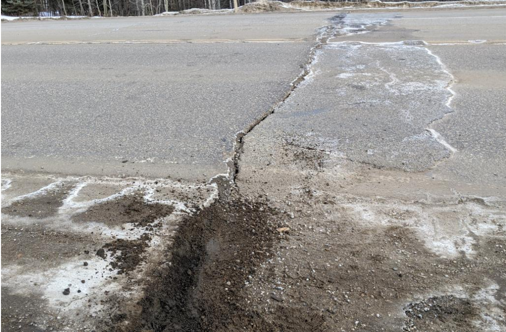
Photo # 1 Looking north at the bump crack (Crack A); there is about 60 to 100 mm drop at the crack location and plough shaved asphalt taper in the middle lane
