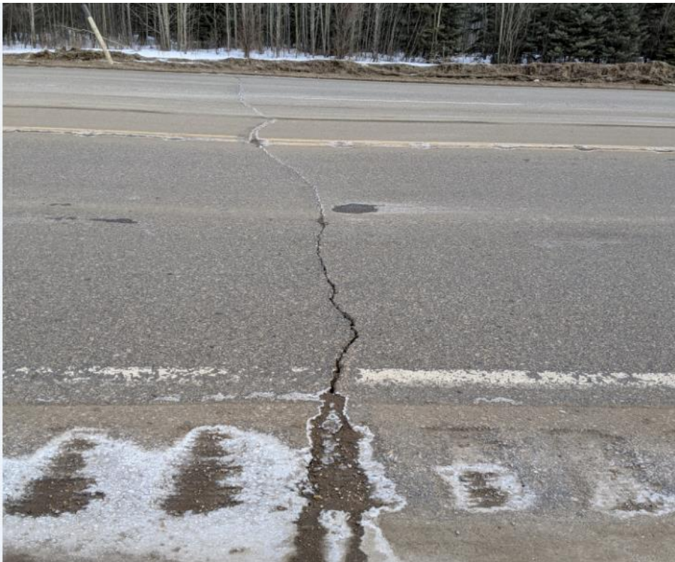
Photo # 6 Looking north at Crack E
