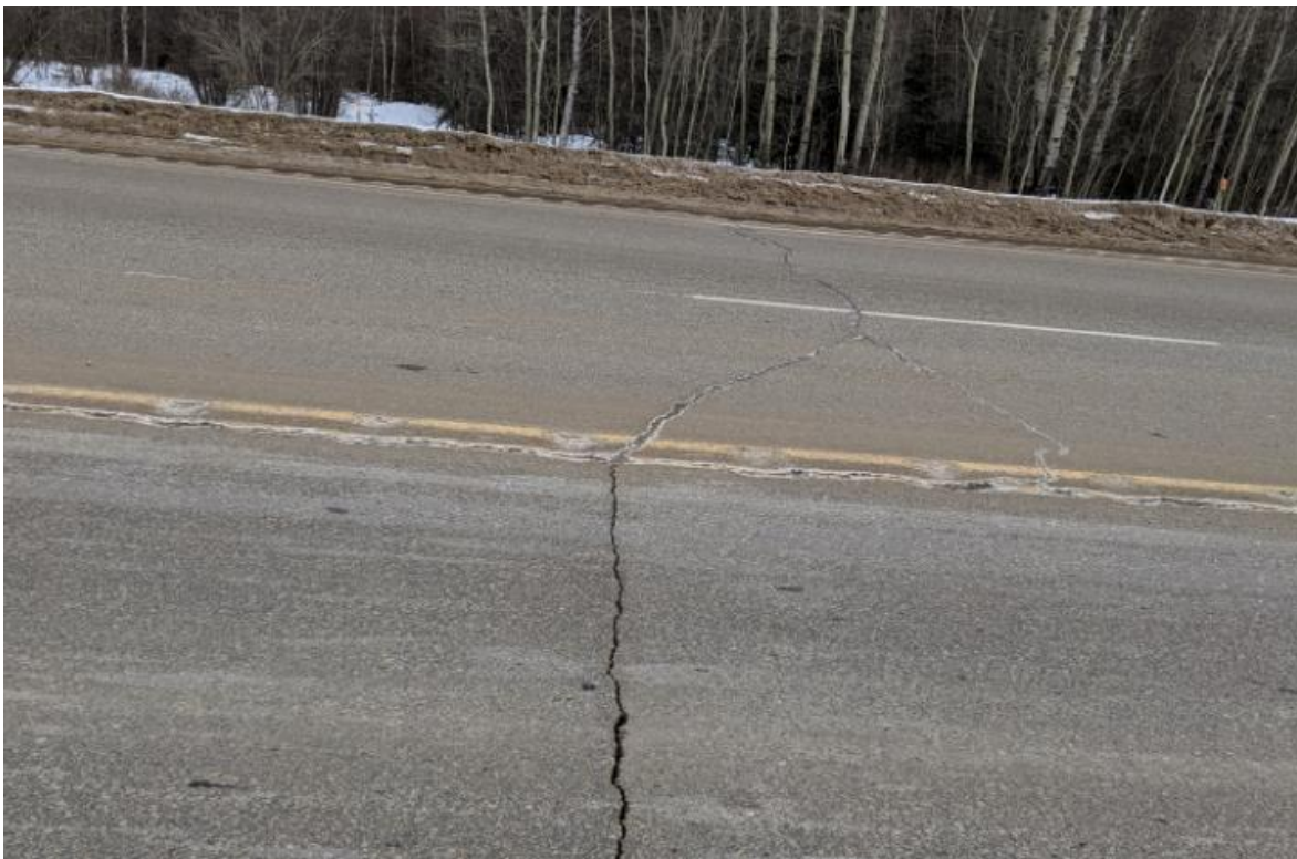
Photo # 2 Looking north at Crack B
