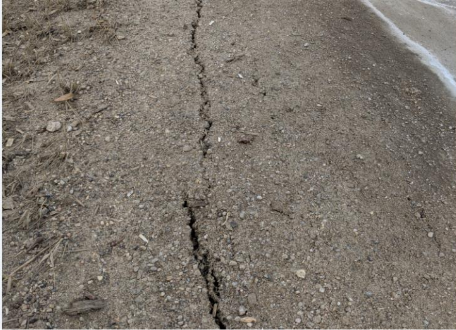
Photo # 5 Looking west at longitudinal crack along the shoulder
