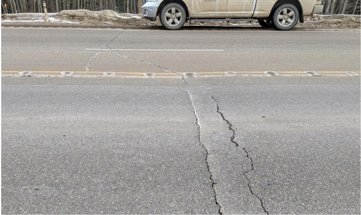
Photo # 3 Looking north at Crack C
