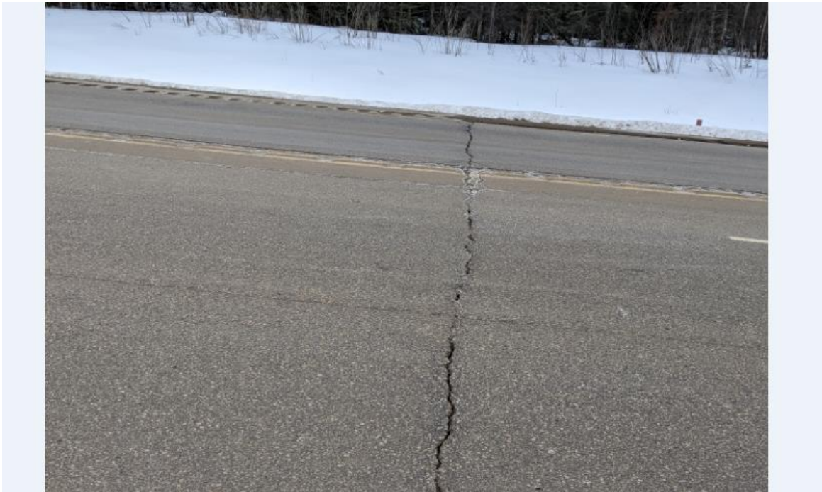
Photo # 4 Looking north at Crack D (East end of treated section)
