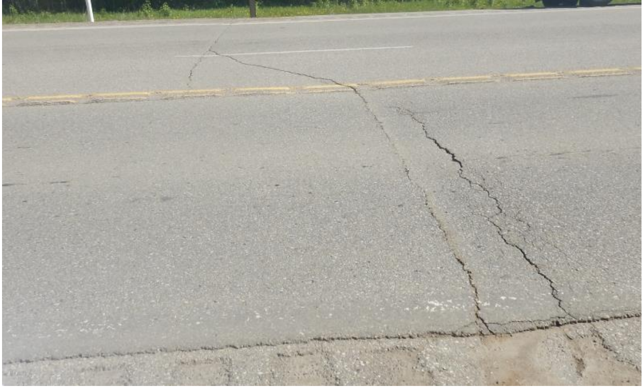
Photo # 3 Looking north at Crack C
