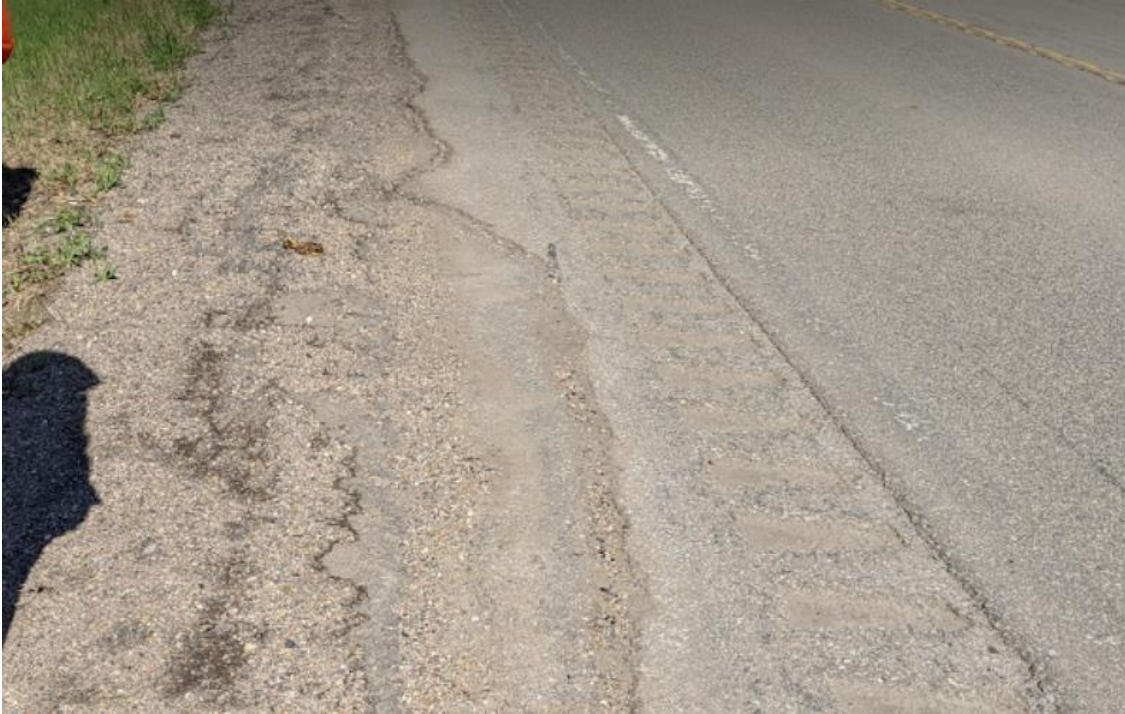
Photo # 5 Looking west at a longitudinal crack along the highway shoulder
