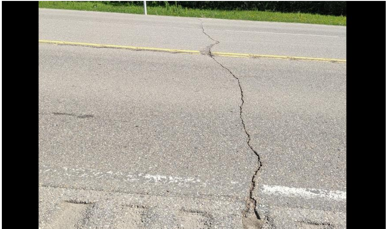
Photo # 6 Looking north at Crack E
