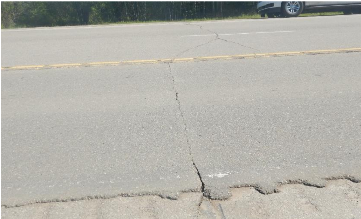
Photo # 2 Looking north at Crack B
