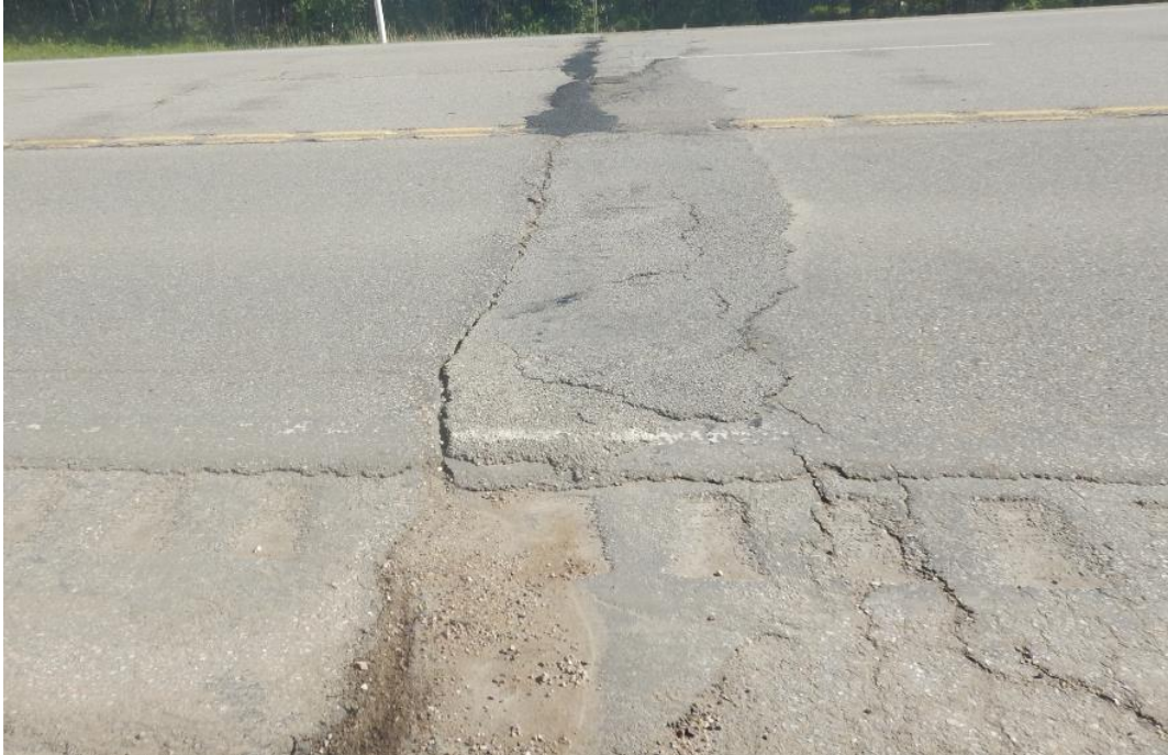
Photo # 1 Looking north at the bump crack (Crack A); there is about 50 mm drop at the crack location; drop is more noticeable within the EBL
