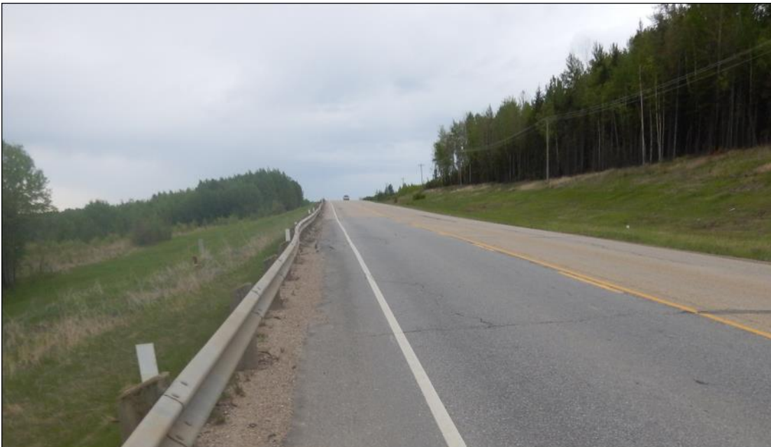
Photo No. 2 – Looking east at reflective cracks near the western limit of the landslide
