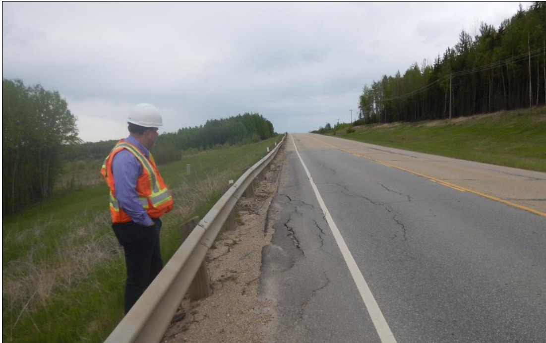
Photo No. 3 – Most active landslide block impacting the highway (middle section of landslide mass); note the presence of multiple retrogressive cracks impacting the highway WBL
