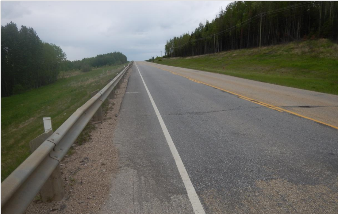
Photo No. 1 – Looking east towards the landslide and the extent of 2021 ACP patch
