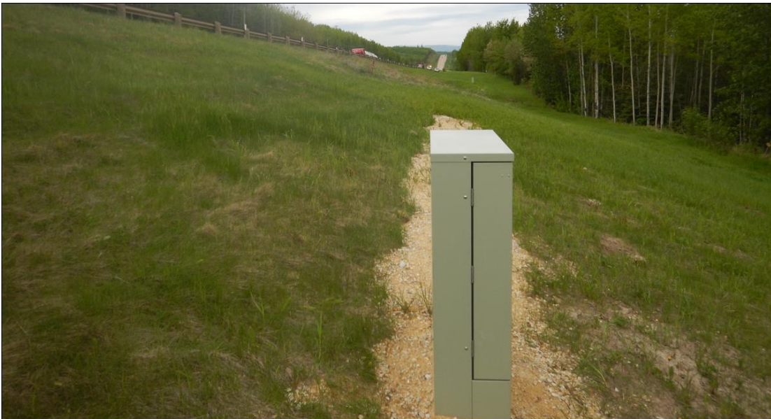
Photo No. 8 – Looking west at the TELUS box installed as part of the line relocation in 2024
