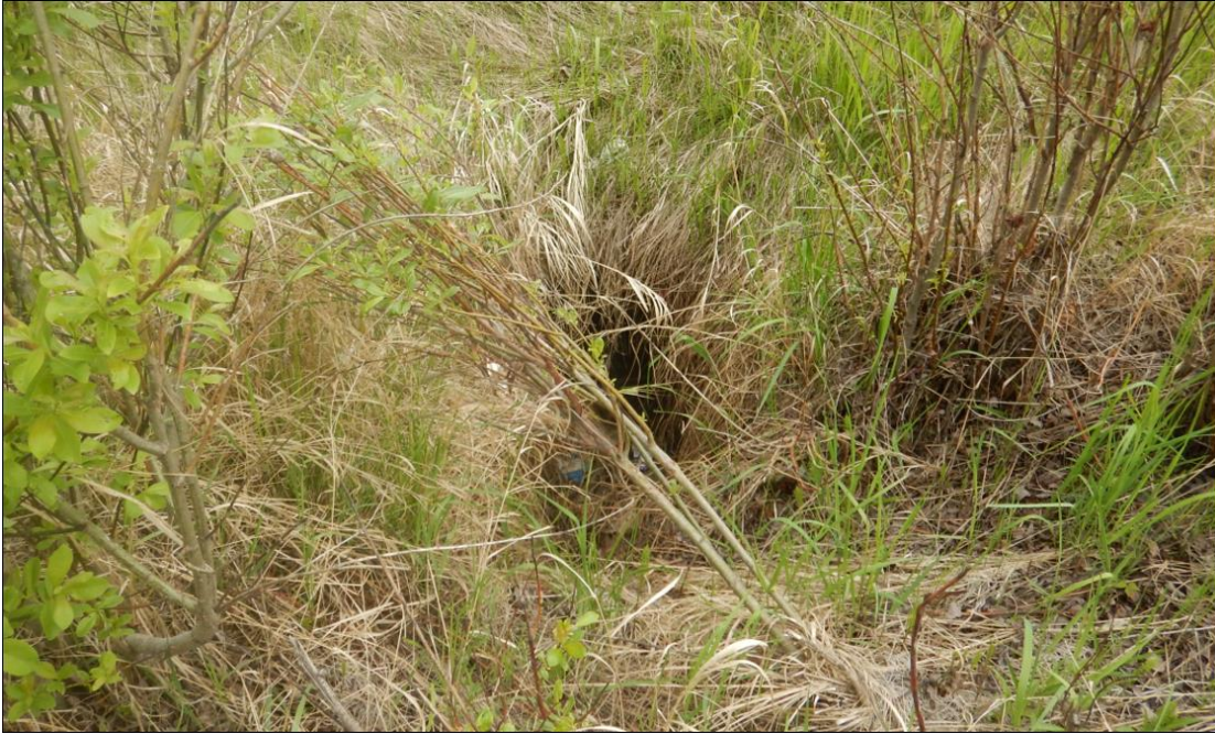
Photo No. 7 – 800 mm diameter culvert inlet. Culvert was rusty, partially blocked with vegetation and filled with garbage
