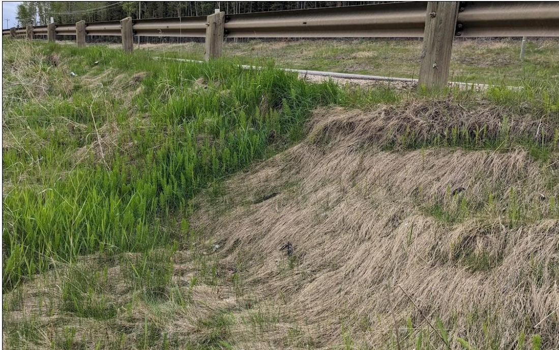
Photo No. 5 – Middle landslide block: Head scarp crack retrogressing into the highway; 600 to 1.2 m drop from original ground ( no change from 2023)
