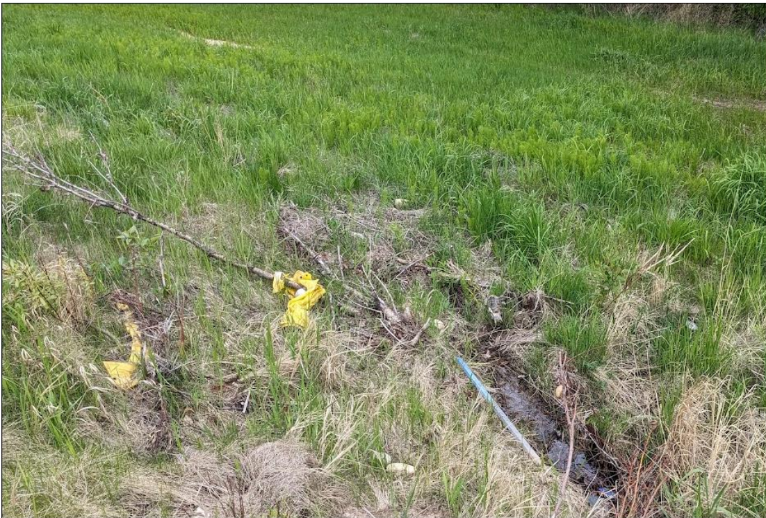
Photo No. 10 – Looking at Settlement Crack / Winter Benching. Note seepage at the bottom right of the photo
