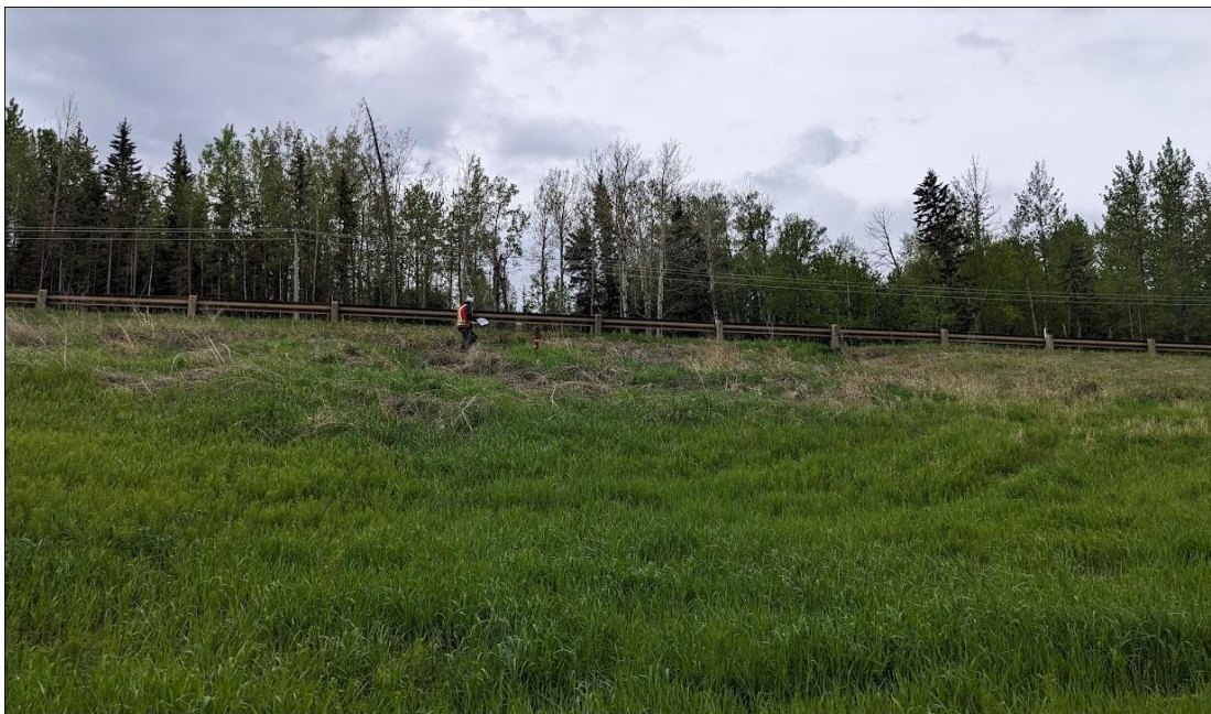
Photo No. 6 – Looking south at active landslide scarp cracks on the highway side slope
