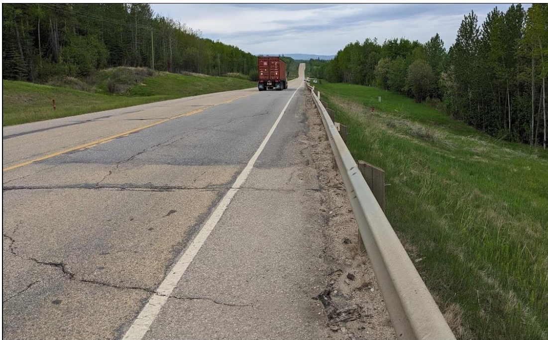
Photo No. 4 – Looking west at reflective cracks from the eastern limit of the landslide
