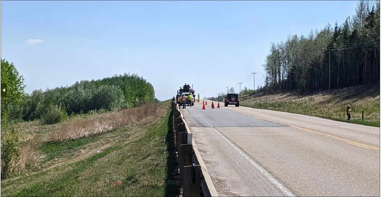
Photo No. 1 – Looking east toward the landslide and the 2021 ACP patch; more vegetation grew on the highway side slope within the landslide mass
