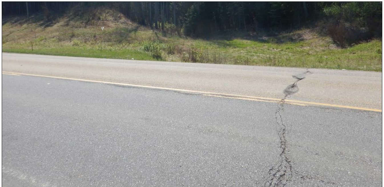
Photo No. 8 – Looking south at patched potholes on the east bound lane
