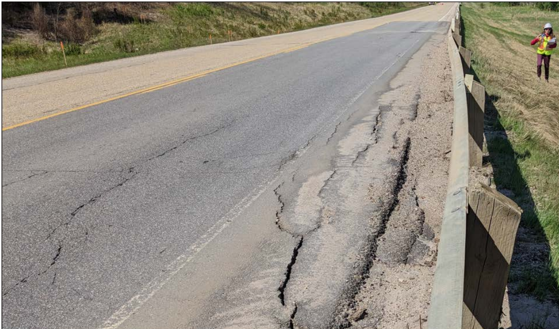
Photo No. 4 – Looking west at the most active area; note guardrail bowing out by 300 mm
