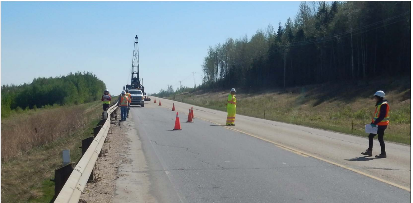
Photo No. 2 – Looking east at reflective cracks near the western limit of the landslide
