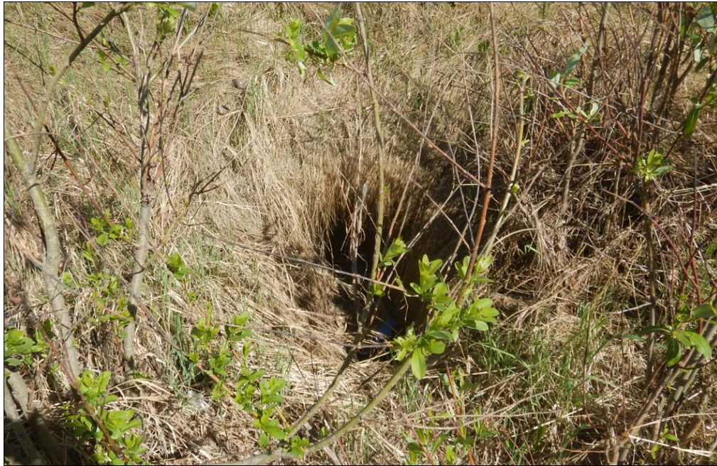
Photo No. 7 – 800 mm diameter culvert inlet. Culvert was rusty, partially blocked with vegetation and filled with garbage.
