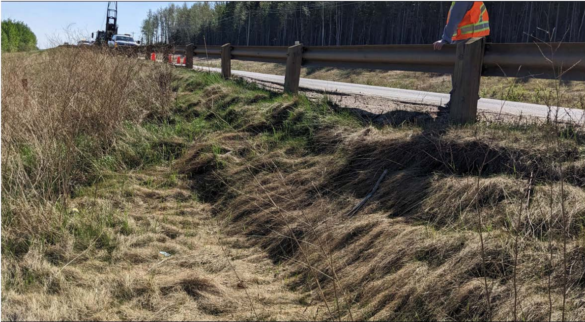
Photo No. 5 – Middle landslide block: Head scarp crack retrogressing into the highway; 600 to 1.2 m drop from original ground
