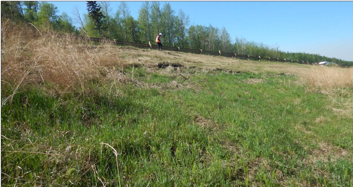
Photo No. 6 – Looking west at active landslide cracks on the highway side slope; these cracks may reflect the failure of the restored drill benches constructed in the winter of 2020 to install geotechnical instruments.
