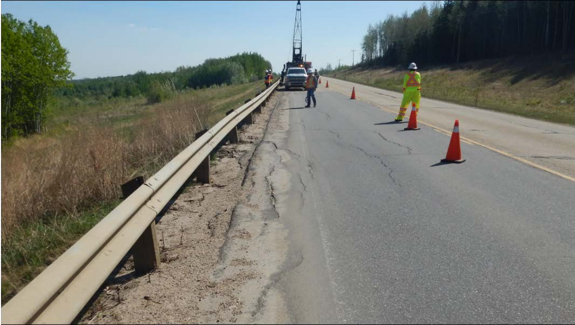
Photo No. 3 – Most active landslide block impacting the highway (middle section of landslide mass); note the presence of multiple retrogressive cracks impacting the highway WBL
