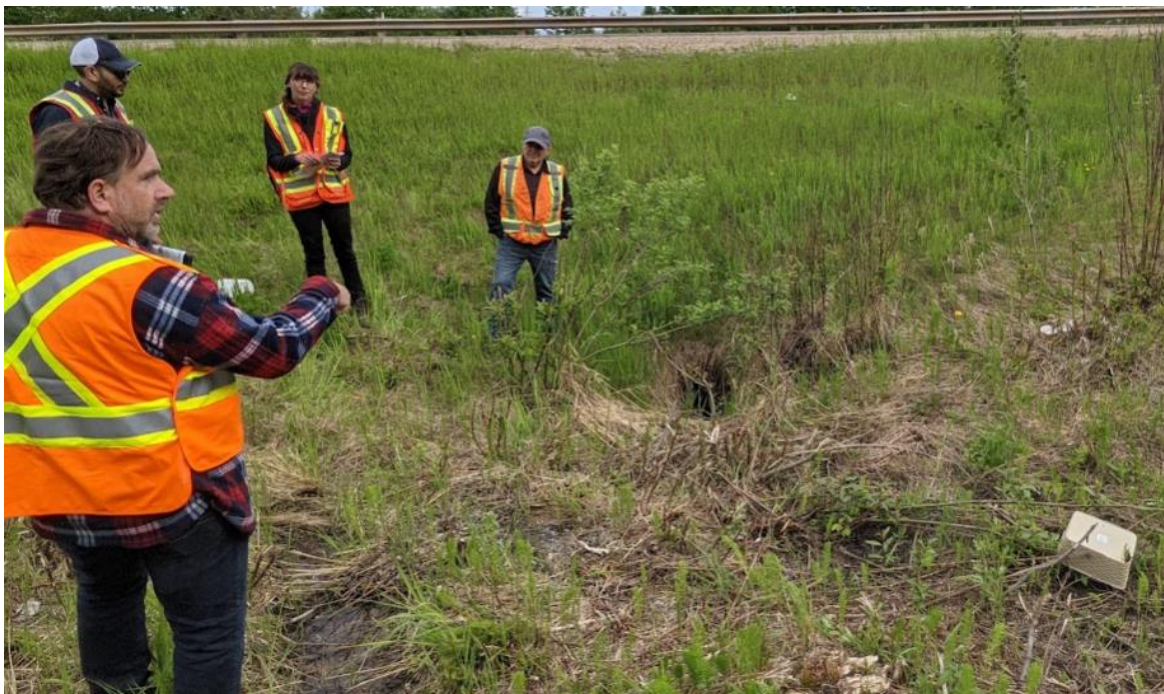
Photo No. 8 – 760 mm diameter culvert inlet. Culvert was rusty and filled with garbage
