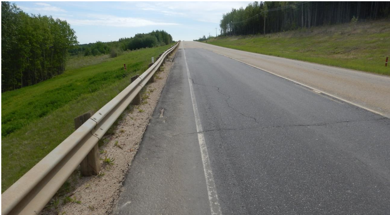
Photo No. 2 – Looking east at reflective cracks near the eastern limit of the landslide
