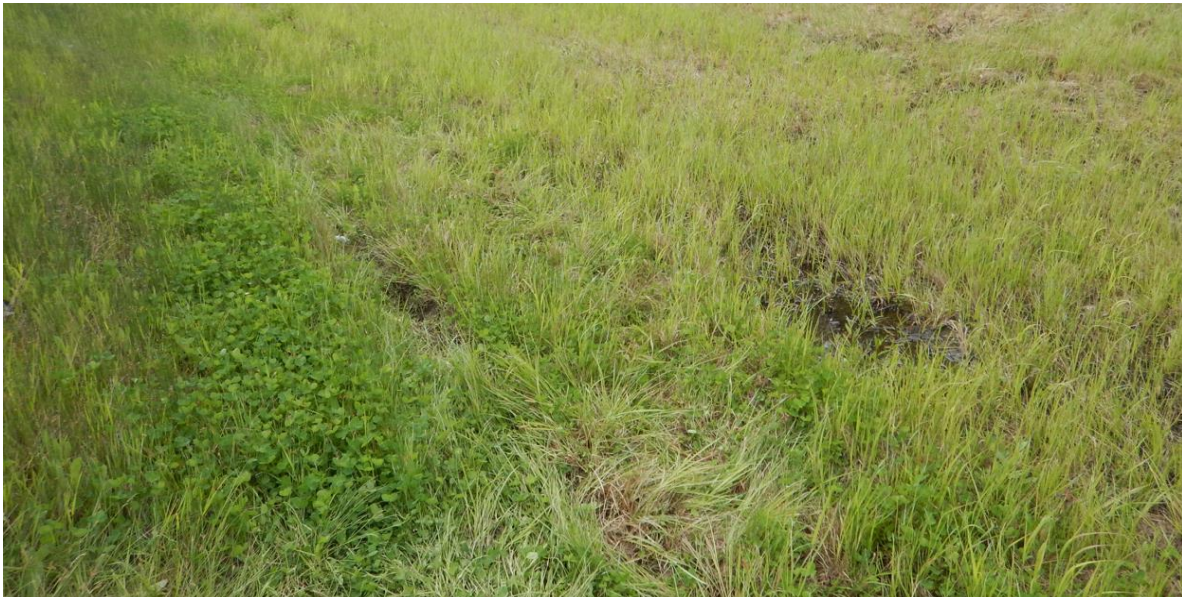
Photo No. 10 – Looking at wet area within the south ditch to the east of the 760 mm CSP culvert inlet location
