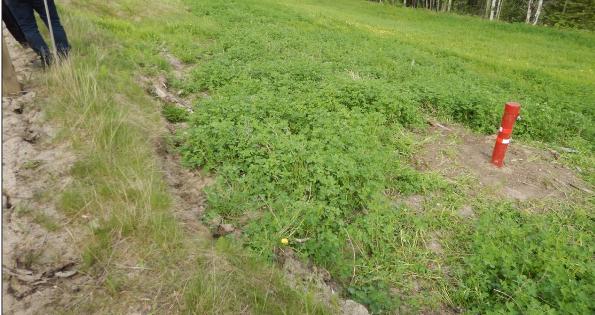
Photo No. 7 – Looking west at active landslide cracks on the highway side slope; these cracks may reflect the failure of the restored drill benches constructed in the winter of 2020. to install the instrumentation.
