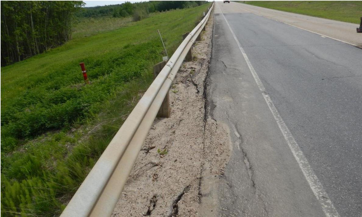
Photo No. 3 – Most active landslide block impacting the highway (middle section of landslide block); note the presence of multiple retrogressive cracks impacting the highway WBL
