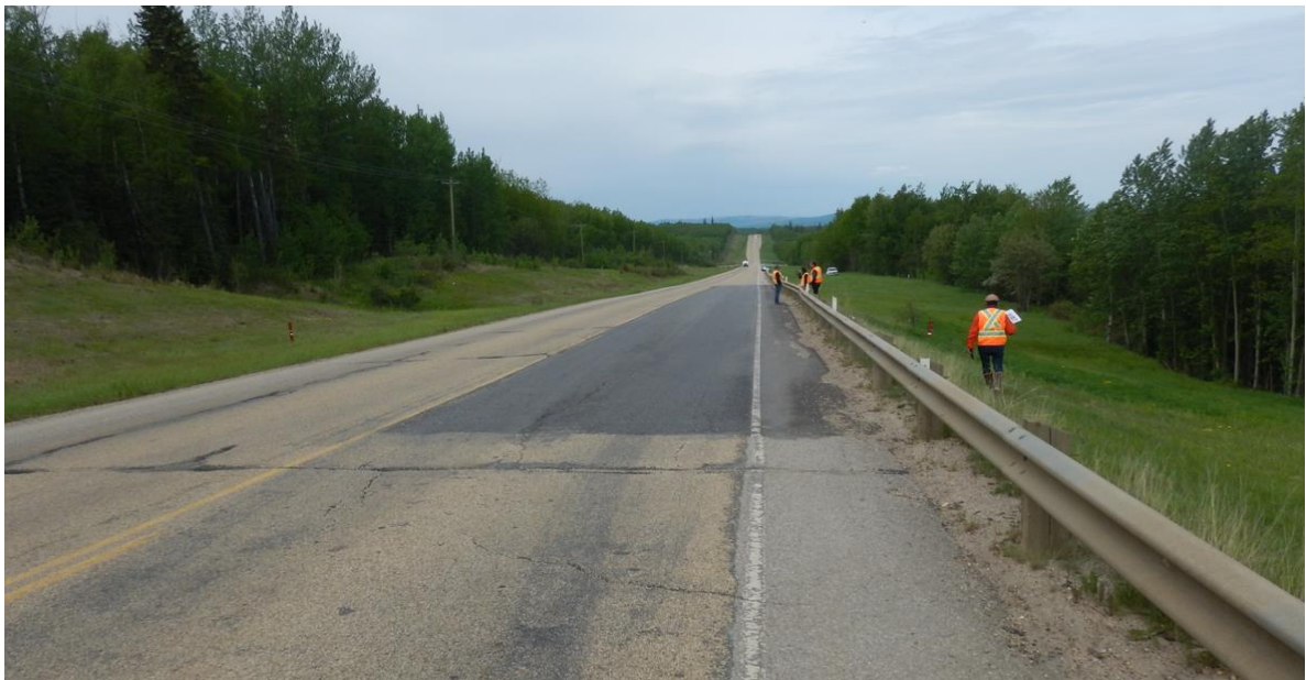
Photo No. 4 – Looking west toward the landslide and 2021 ACP patch; landslide cracks extend beyond the patched area
