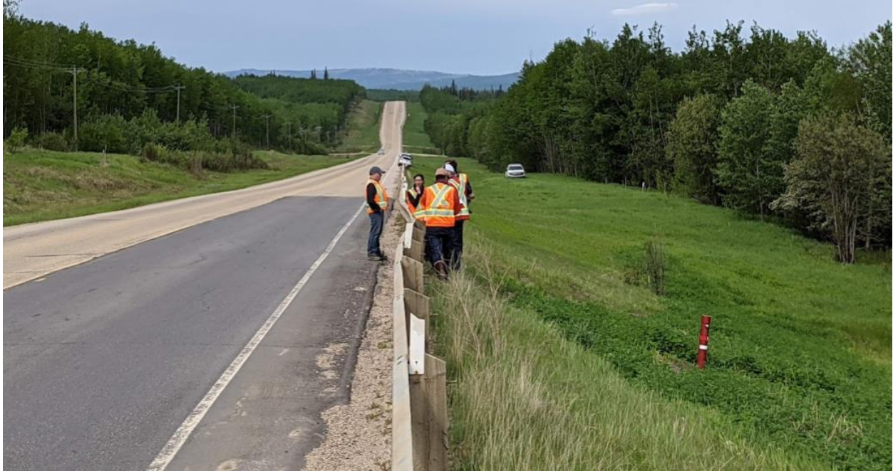
Photo No. 5 – Looking west at the most active area; note guardrail bowing out by 250 mm
