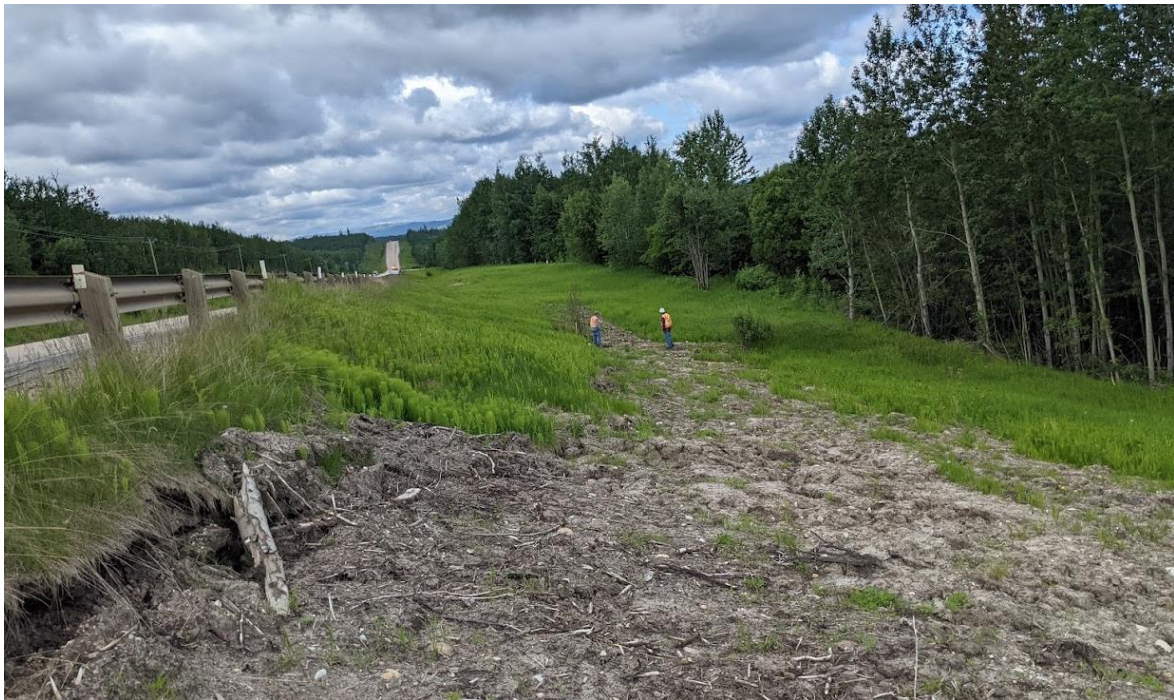
Photo No. 10 - Tension cracks on the side slope extending up to the guardrail
