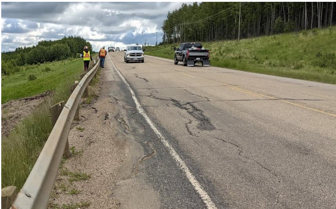
Photo No. 4 – Most active landslide block impacting the highway (middle section of landslide block). Note multiple retrogressive cracks impacting the highway WBL; cracks are 30 to 60 mm wide X 70 mm deep under the guardrail with up to 150 mm drop
