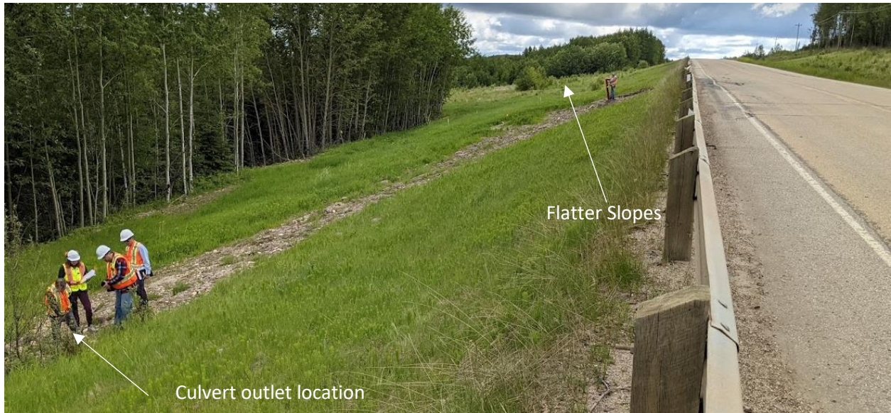
Photo No. 1 – Looking east toward the landslide and side slope distress between eastern edge of the tree line and the culvert outlet location. Note flatter side slopes constructed east of the tree line as part of the old landslide repair completed in 2007
