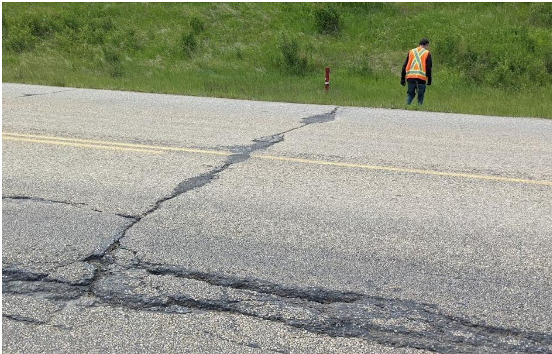
Photo No. 12 – Looking south at patched potholes on the east bound lane
