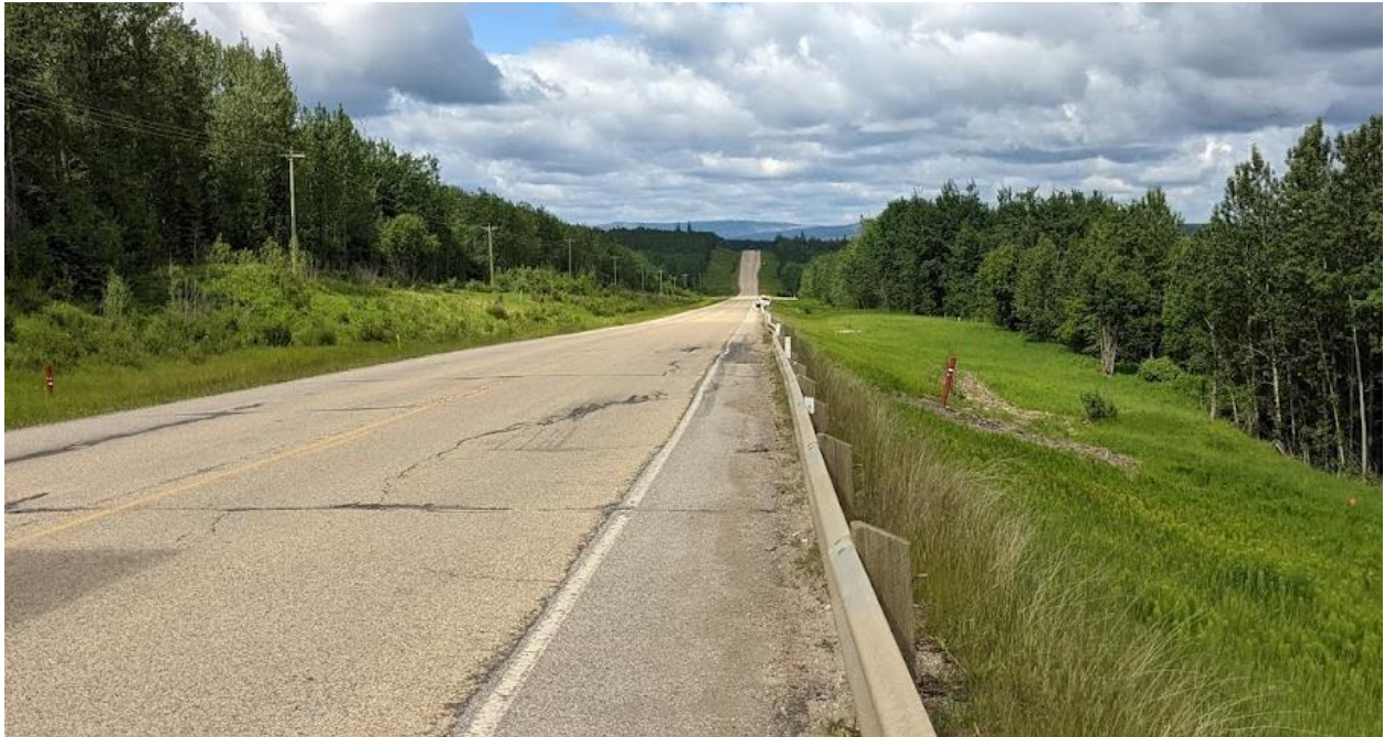
Photo No. 5 – Diagonal cracks to the east of the most active area (up to 200 mm wide with 80 mm drop)
