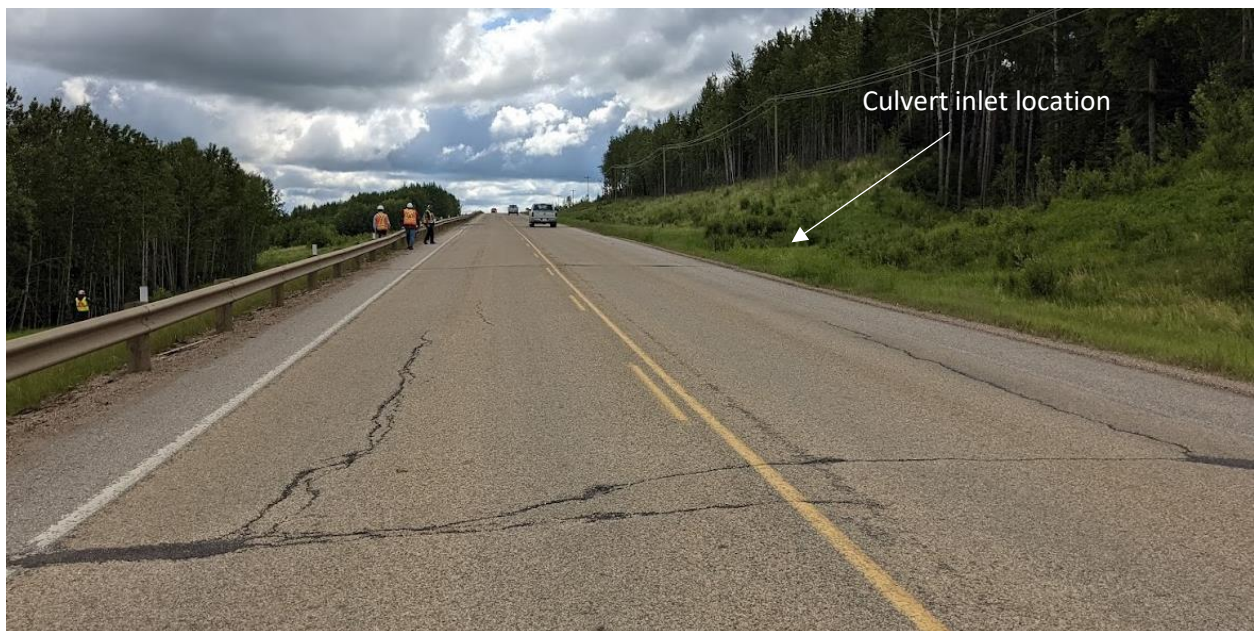
Photo No. 2 – Looking southeast at a transverse crack. Note the presence of a natural gully at the back slope as well as power lines
