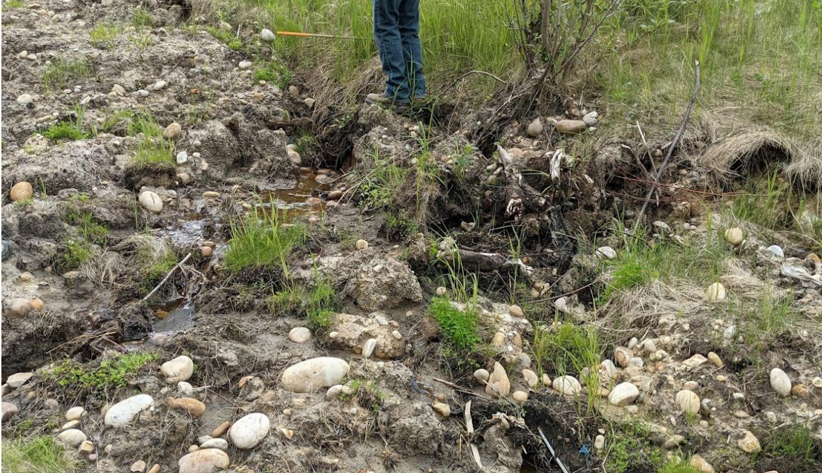
Photo No. 7 – Looking at damaged 900 mm culvert outlet. Water is still flowing from the culvert outlet
