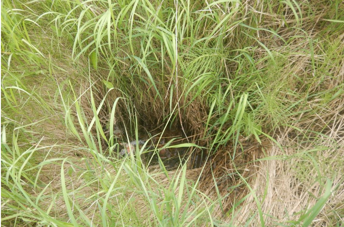
Photo No. 11 – 900 mm diameter culvert inlet. Culvert was rusty and filled with garbage
