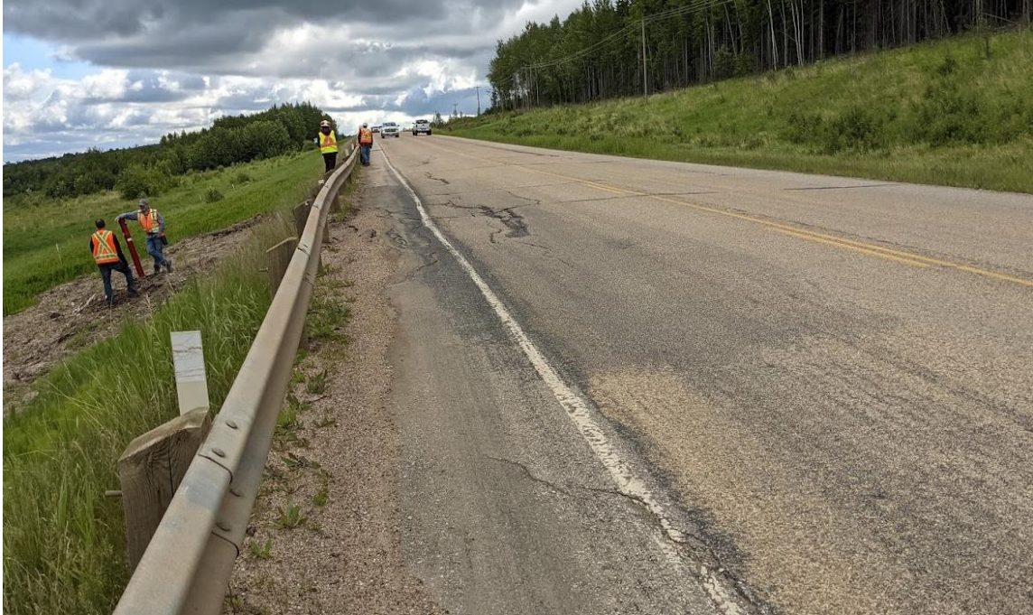
Photo No. 3 – Diagonal cracks on the highway surface near the western flank of the landslide (western section of landslide block)
