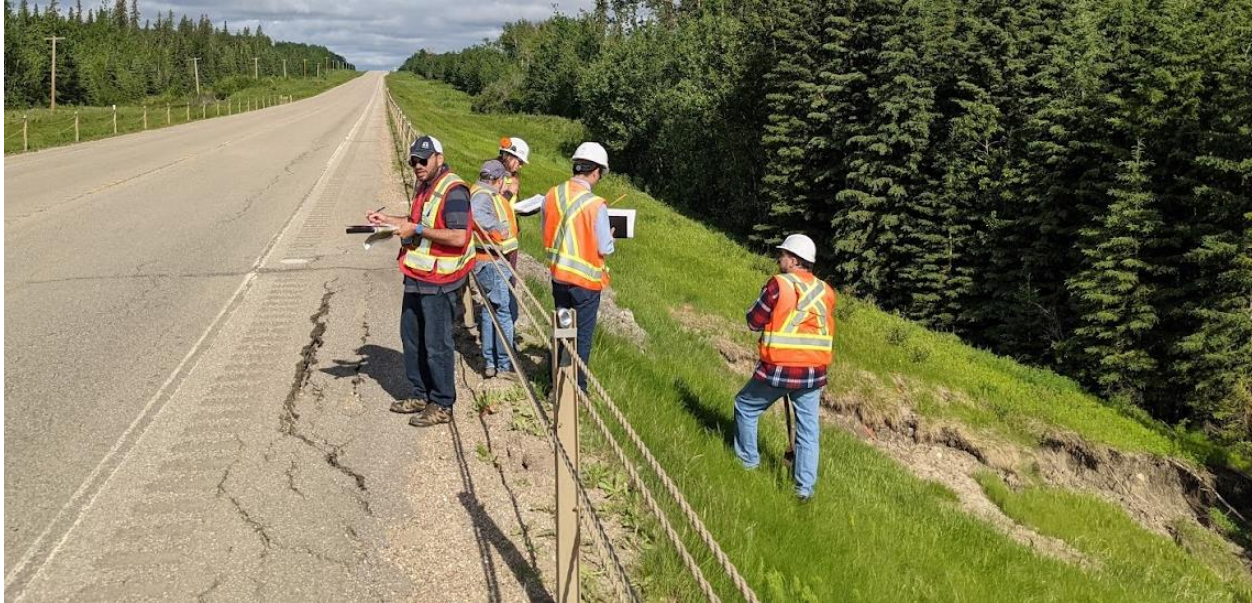
Photo No. 1 – Looking at WBL landslide; note the presence of open tension cracks on the highway shoulder; main head scarp crack of landslide is about 2.8 m from the HTC
