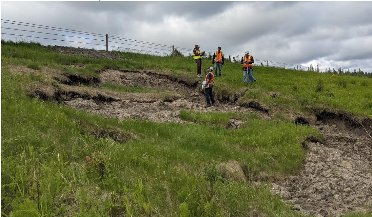
Photo No. 2 – Looking southwest at the north embankment landslide's head scarp crack and western flank; landslide mass was noted to be dry in 2022
