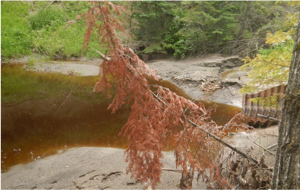
Photo No. 5 – Looking east; water ponding a bit around culvert outlet location
