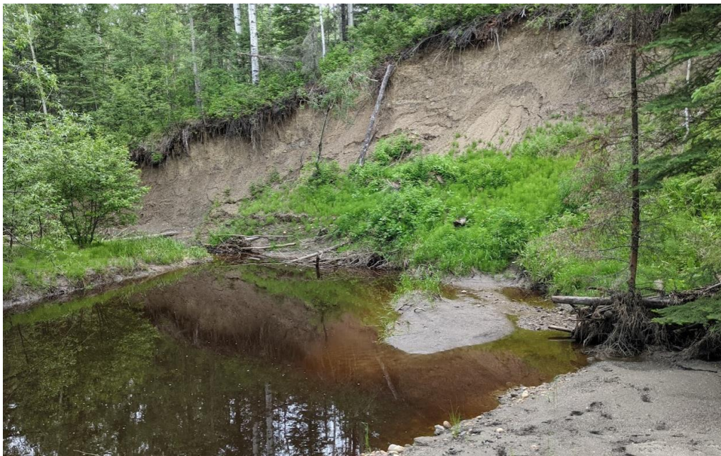
Photo No. 4. Looking northwest at the CSP culvert outlet; note water continues to pond in this area
