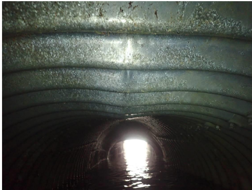
Photo No. 8 – Looking inside CSP Culvert outlet; note reverse curvature in the roof (Photograph was taken by AT during bridge culvert inspection completed on June 3,2020). This is approximately 27 to 30 m from the culvert outlet location.
