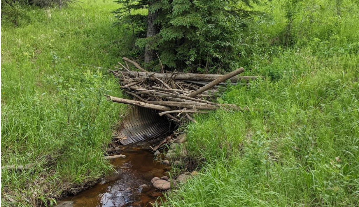
Photo No. 7 – Looking at CSP Culvert Inlet (1.9 m diameter); scattered riprap was noted at inlet location
