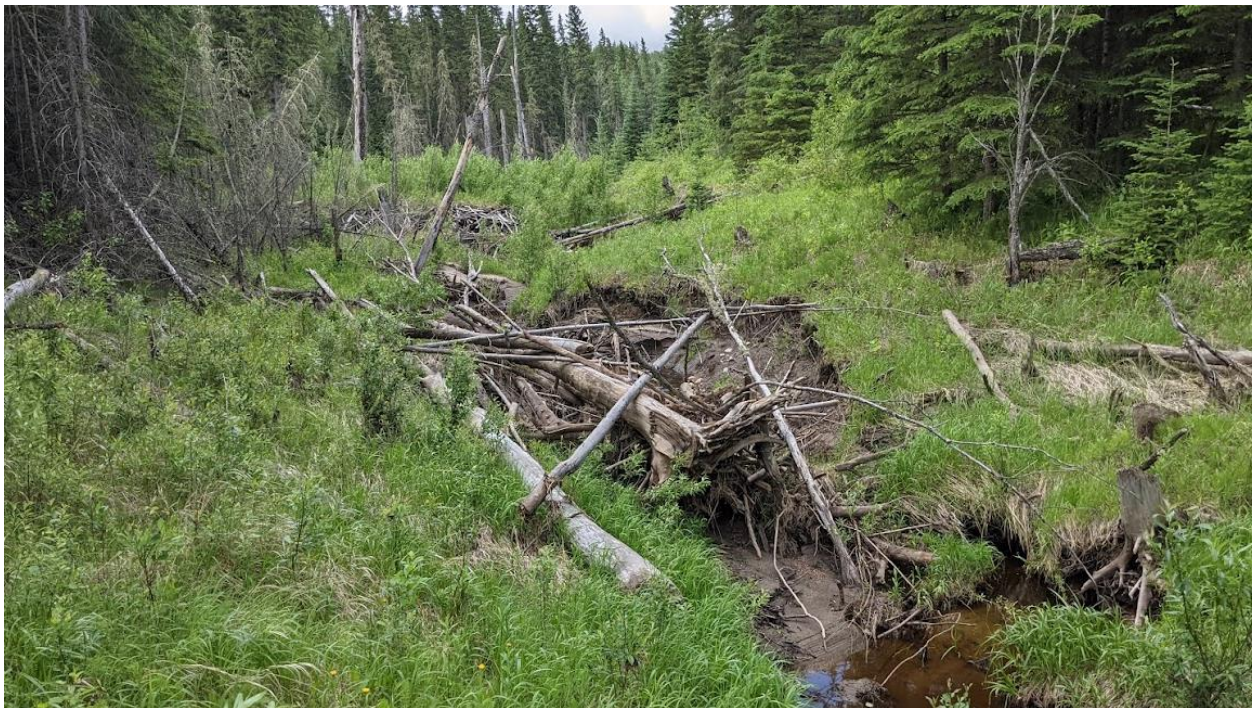
Photo No. 6 – Two beaver dams noted upstream of the culvert inlet
