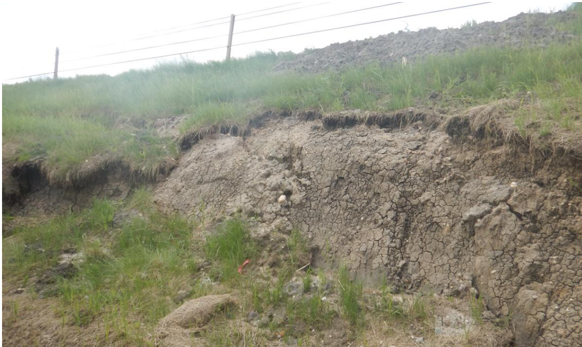
Photo No. 3 – Looking southeast at the landslide’s head scarp and eastern flank; multiple tension cracks noted between the head scarp and the guardrail during the previous inspection were buried under drill cuttings
