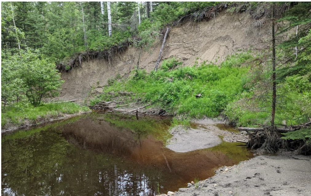
Photo No. 4. Looking northwest at the CSP culvert outlet; note water ponding near the culvert outlet
