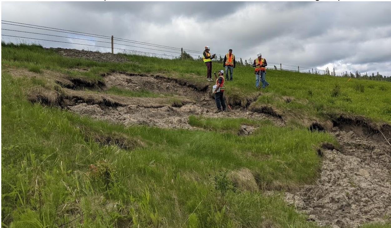
Photo No. 2 – Looking southwest at the north embankment landslide's head scarp and western flank; landslide mass was noted to drier than in 2020.
