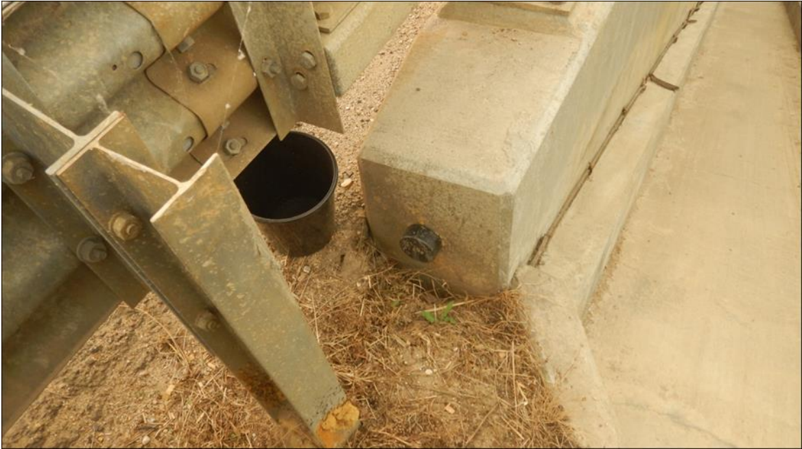
Photo 7. Looking at 100 mm wide x 200 mm deep void at the end of the wing wall
