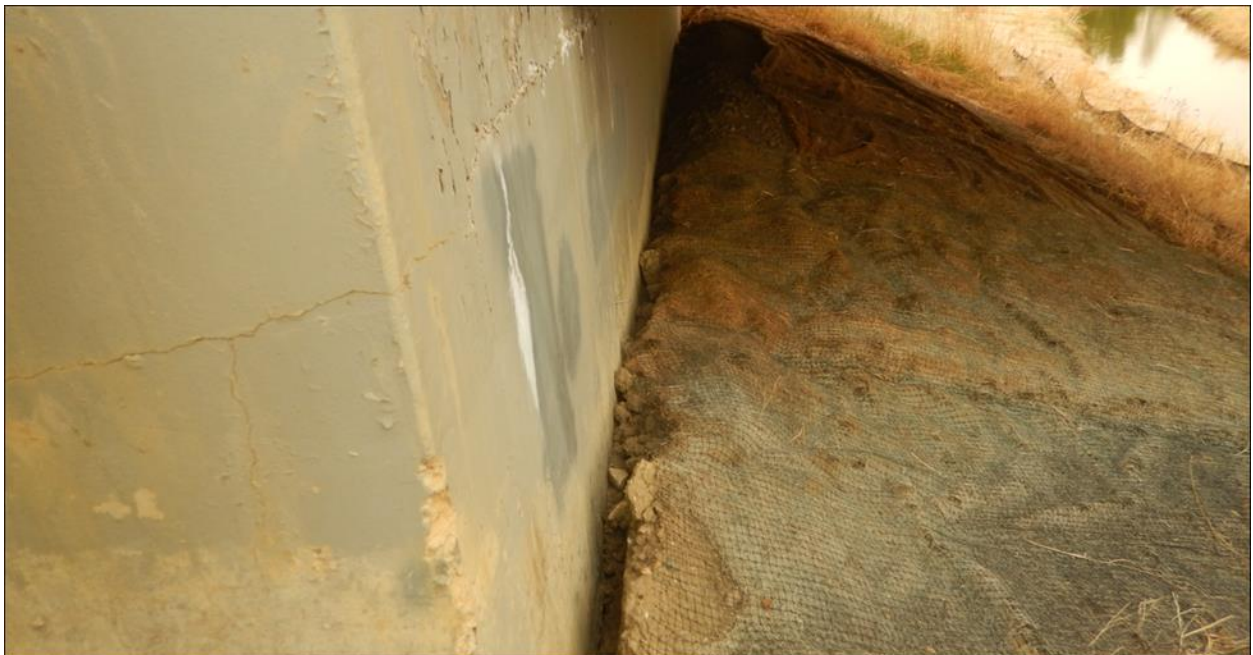
Photo 6. Shrinkage crack along the face of the abutment seat (200 mm wide, 450 mm deep, 2 m long)
