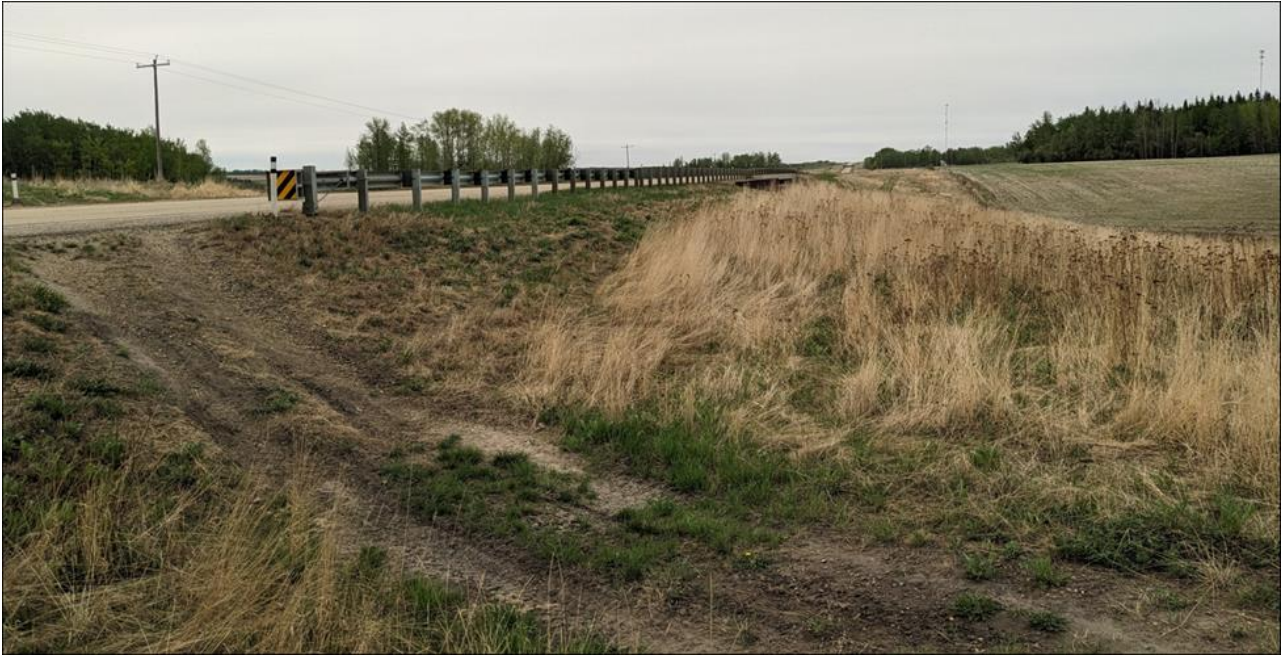
Photo 3. Looking south at the highway west ditch to the north of the repaired area.
