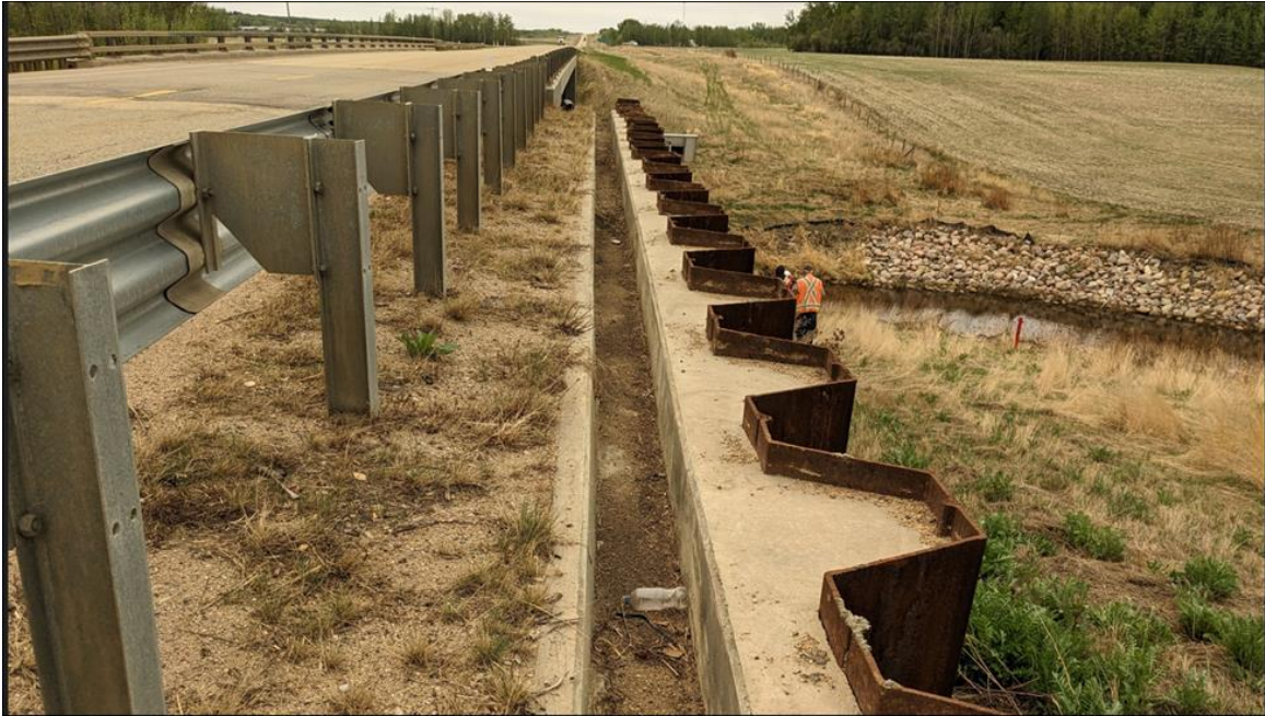
Photo 5. Looking south at guardrail and concrete drain trough behind Sheet Pile Wall B; accumulated debris from the road in the drain trough.
