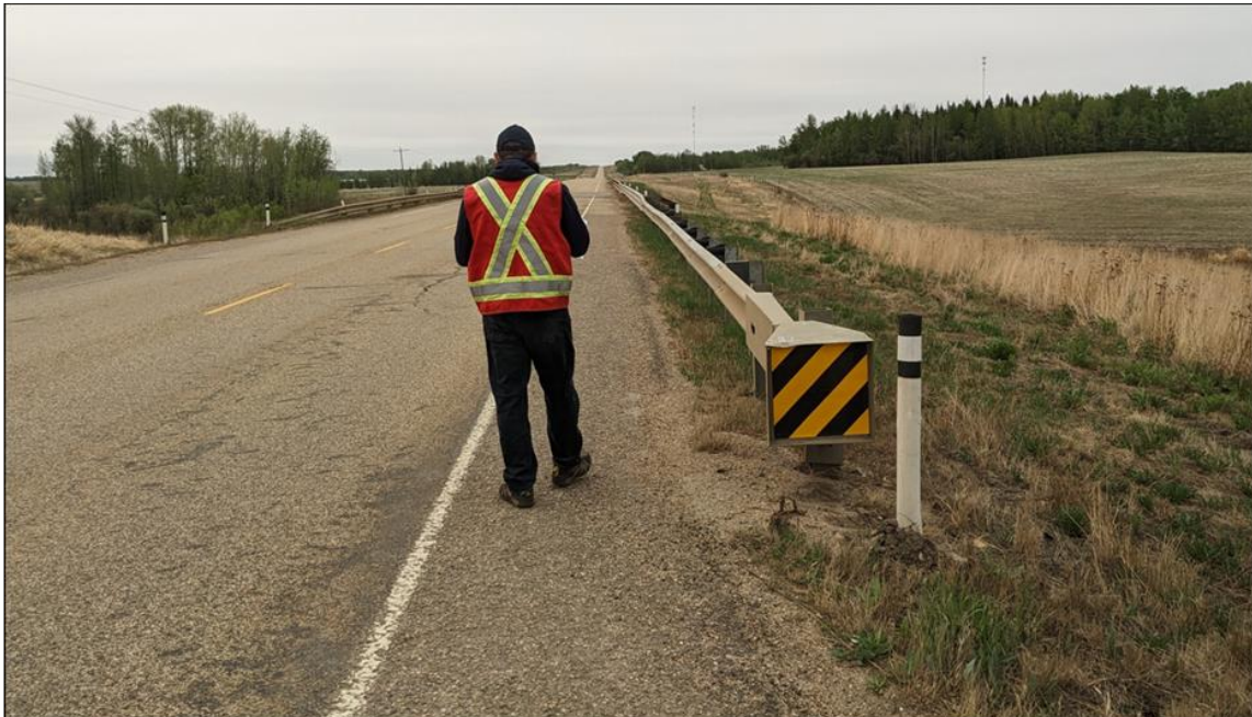
Photo 1. Looking south at guardrail and embankment west side slope; note growth of grass vegetation within the slope surface
