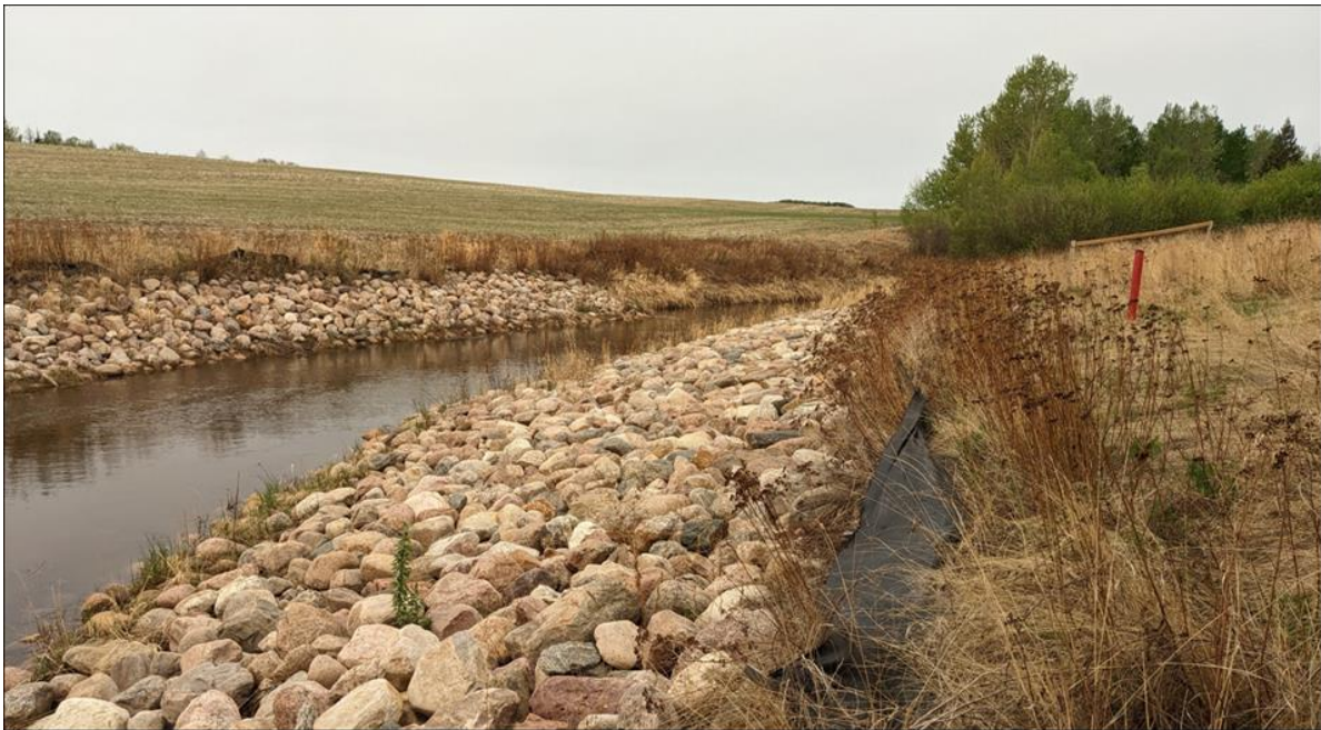
Photo 12. Looking west at the armored creek bank from the bottom of the slope (i.e.at Sheet Pile Wall A location); banks were armored using Class 1 Riprap
