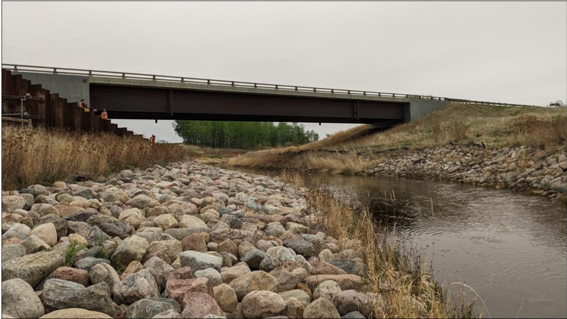
Photo 13. Looking east at the armored creek banks from the bottom of the slope |
