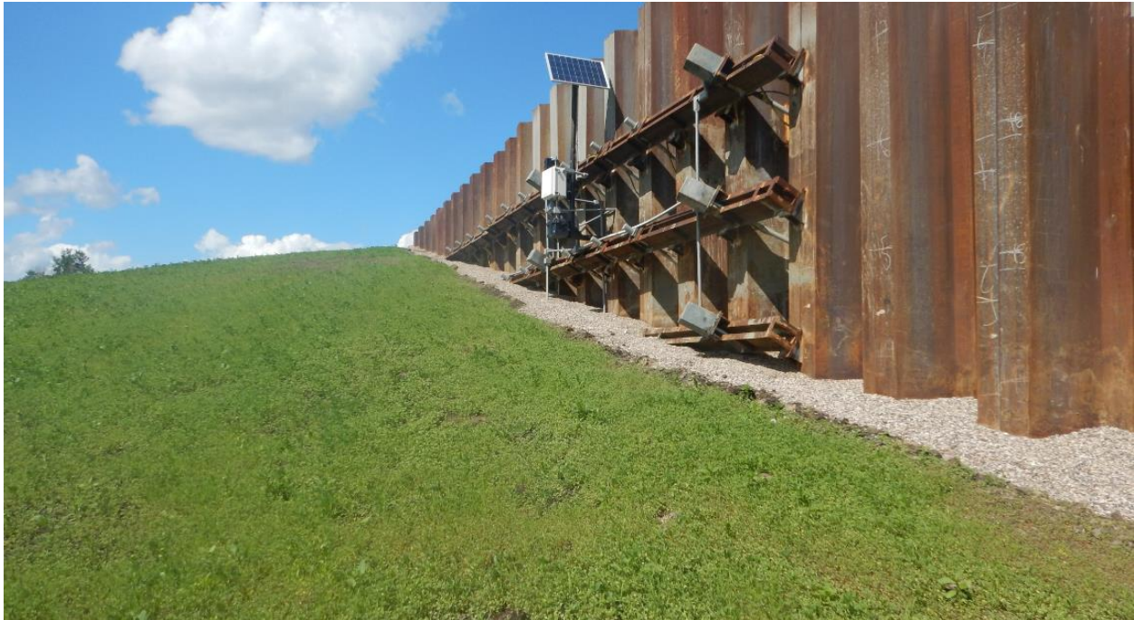
Photo No. 8 – Datalogger and solar panel installed on Sheet Pile Wall B
