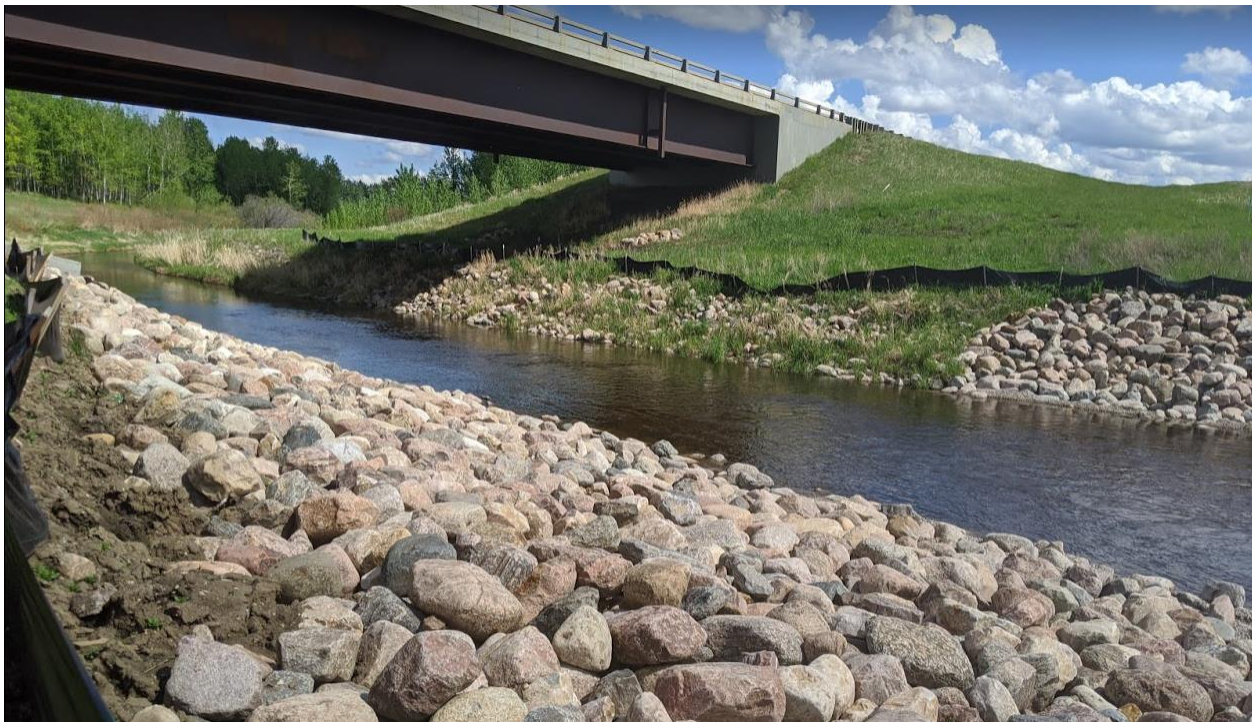
Photo No. 11 – Looking east at the armored creek banks from the bottom of the slope
