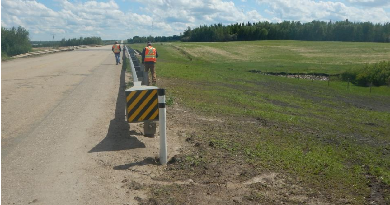
Photo No. 1 – Looking south at new guard rail and embankment west side slope; note growth of grass vegetation within the slope
