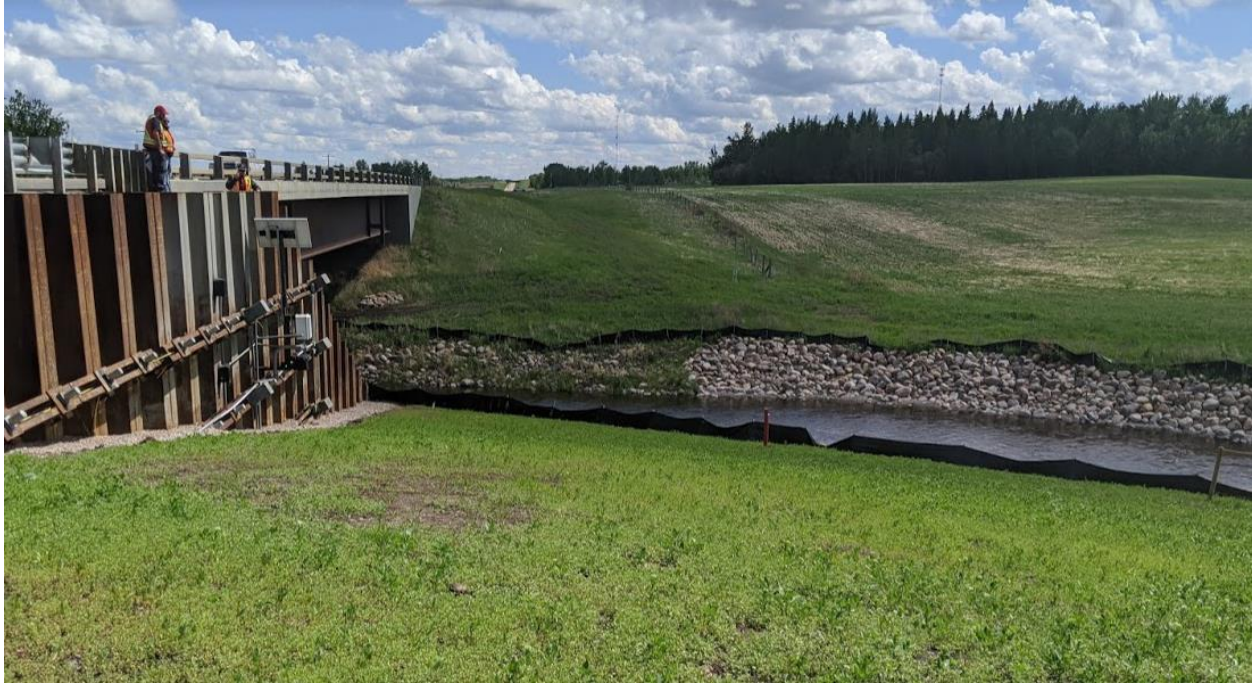
Photo No. 6 – Sheet Pile Wall B with three rows of anchors supporting the highway embankment; Sheet Pile Wall A is buried below ground and is parallel to the toe of the slope.
