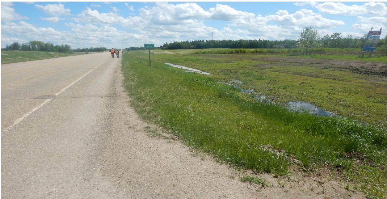
Photo No. 1a – Looking south at the highway east ditch to the south of the repair area; note ponding of surface water in the ditch
