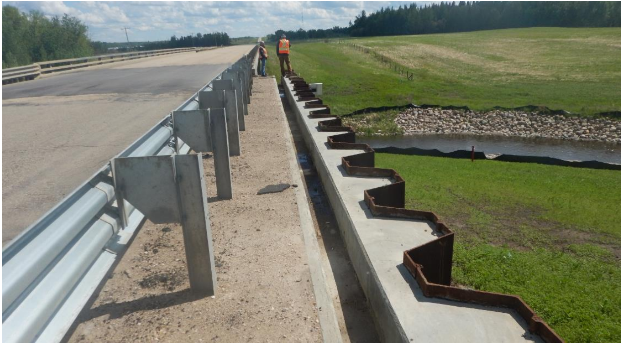
Photo No. 4 – Looking south at guardrail and concrete drain trough behind Sheet Pile Wall B
