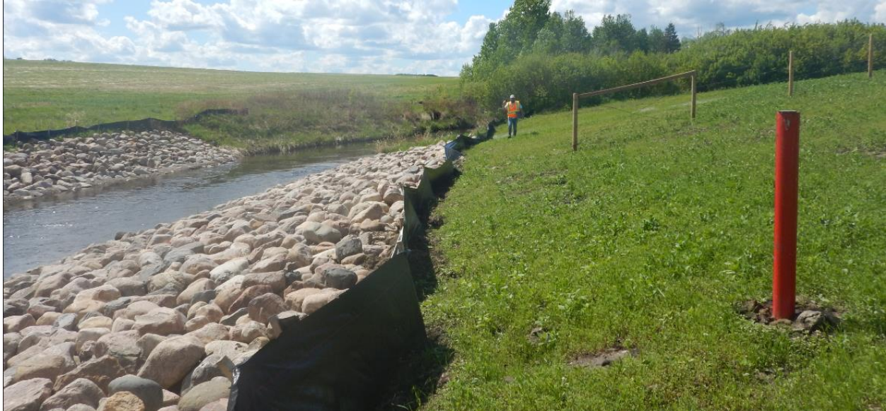
Photo No. 10 – Looking west at the armored creek bank from the bottom of the slope (i.e. at Sheet Pile Wall A location); banks were armored using Class 1 Riprap
