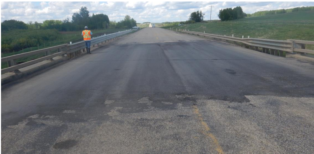
Photo No. 5 – Looking north at a 19 m long ACP patch placed along the highway behind the north abutment
