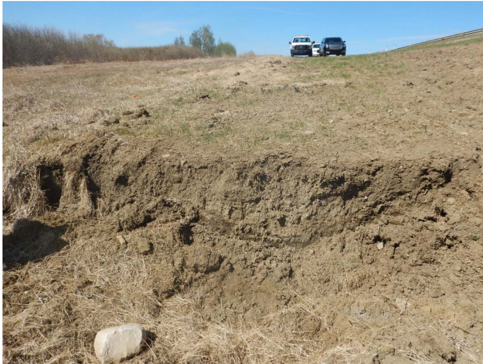
Photo No. 3. - A closer look at the observed seepage from the head scarp crack (Looking North)
