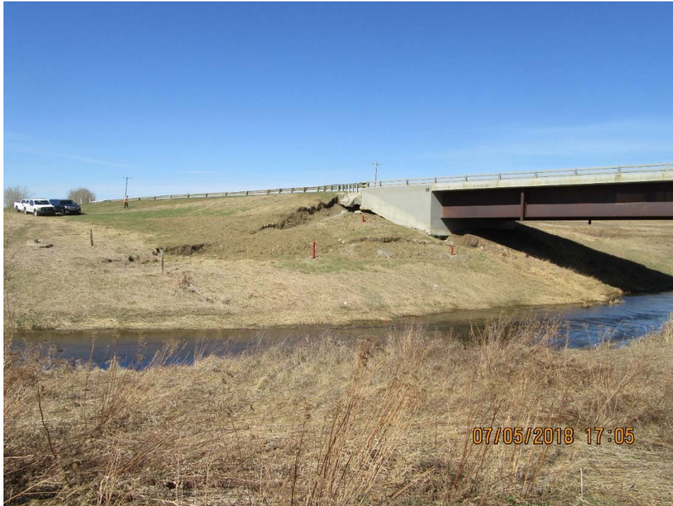
Photo No. 1. - Overall Landslide Area (Looking North)
