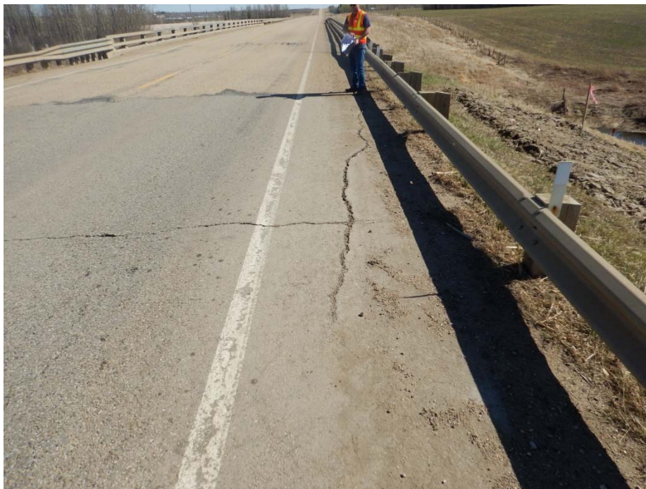
Photo No. 12. Dip in highway surface near the end of the bridge approach slab (Looking South)
