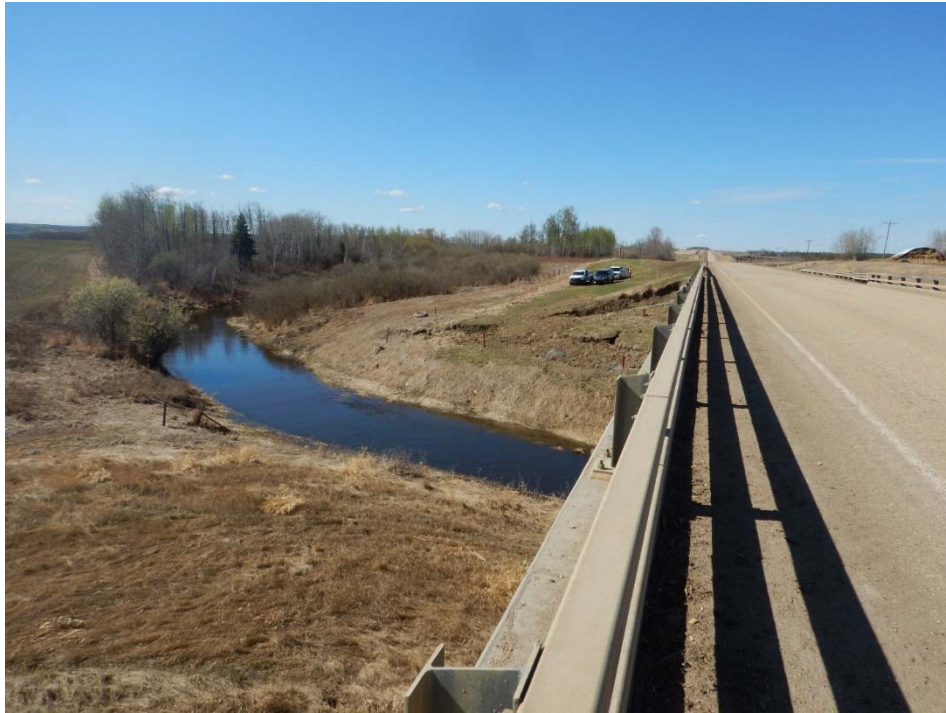
Photo No. 9. - Landslide Area (Looking North)
