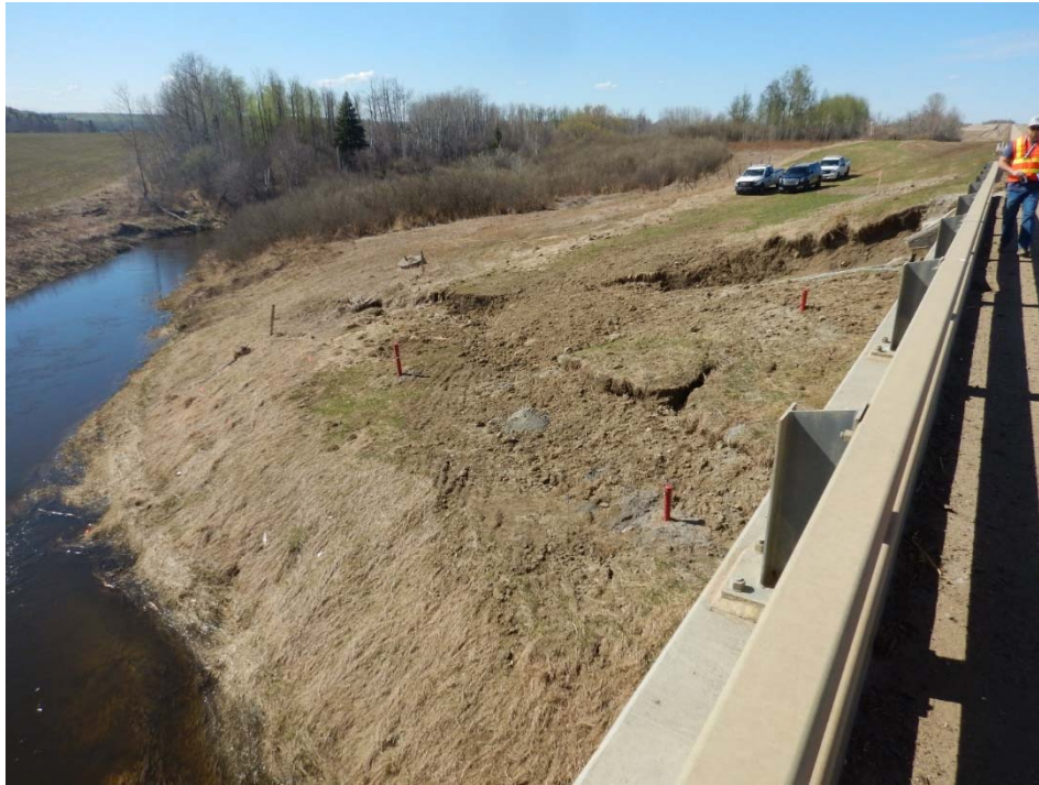
Photo No. 11. Backscarp, Lower Slump and Toe Roll in the Creek (Looking Northwest); the toe roll is reducing the capacity of the creek channel at the landslide location
