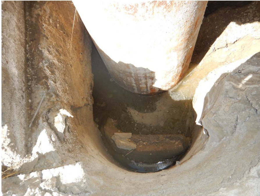
Photo No. 7. - Looking at the exposed casing of the most western abutment pile; the ground surface dropped by at least 1.6 m at this location and water ponded between the casing and the poured concrete slab by the abutment seat.
