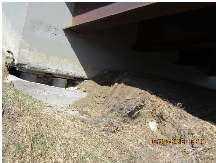
Photo No. 6. Looking north at the exposed abutment pile supports and the eastern flank of the landslide; note the gap developed between the top of the pile casing and the underside of the abutment seat. The gap is more distinguished in the casing adjacent to the eastern flank of the landslide
