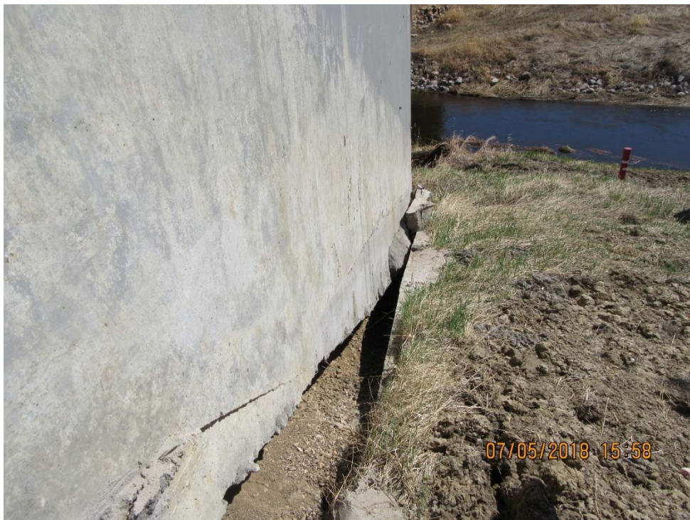
Photo No. 4. - Eastern flank of landslide created a void below the wingwall (Looking South)
