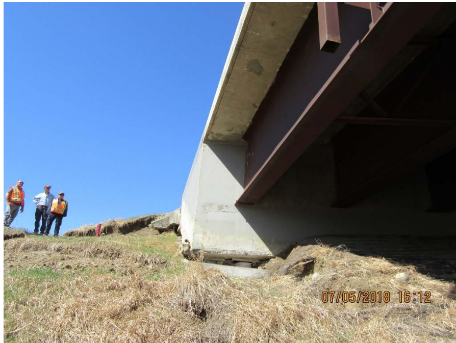
Photo No. 5. - Eastern flank of landslide created a void below the abutment seat (Looking North)
