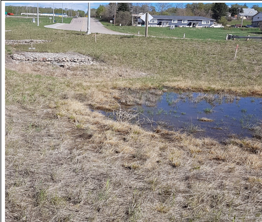
Photo #10. Highway 55 south ditch: Ponding water within a low area to the west of the 1200 mm diameter manhole.
