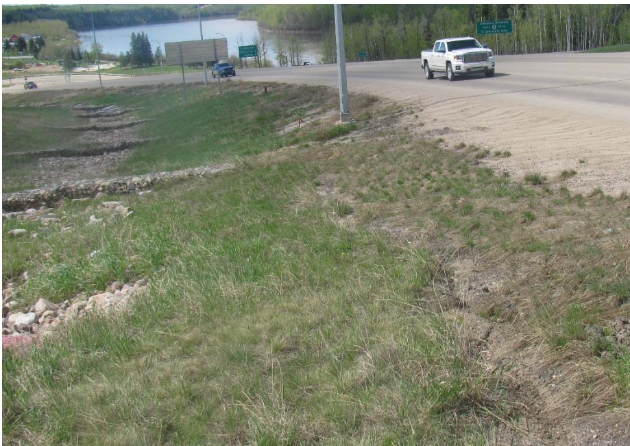
Photo #2. Hwy 55 South Ditch: Looking west at the east end of the existing riprap channel. Note the presence of bare side slopes and an erosion gully on the slope surface
