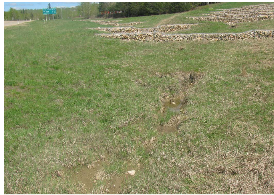
Photo #17. Hwy 55 North Ditch: Erosion gully between G4 and G5
