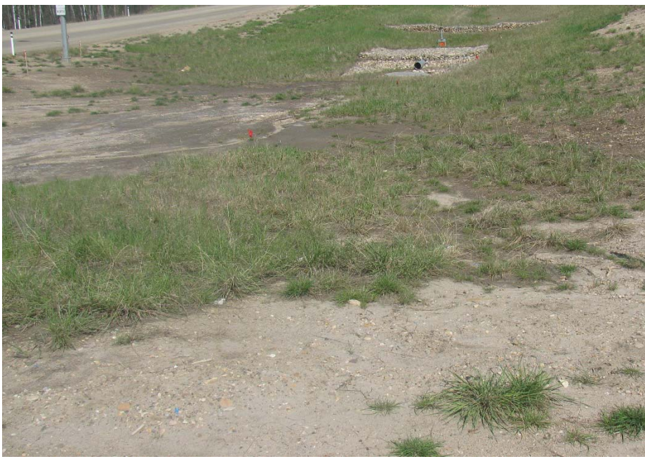
Photo #14. Highway 55 north ditch: Looking east at bare side slopes
