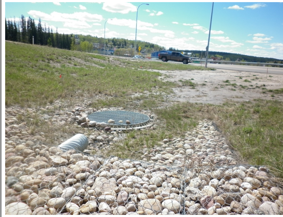
Photo #15. Hwy 55 North Ditch: Looking north from the manhole location at erosion rills and bare slopes
