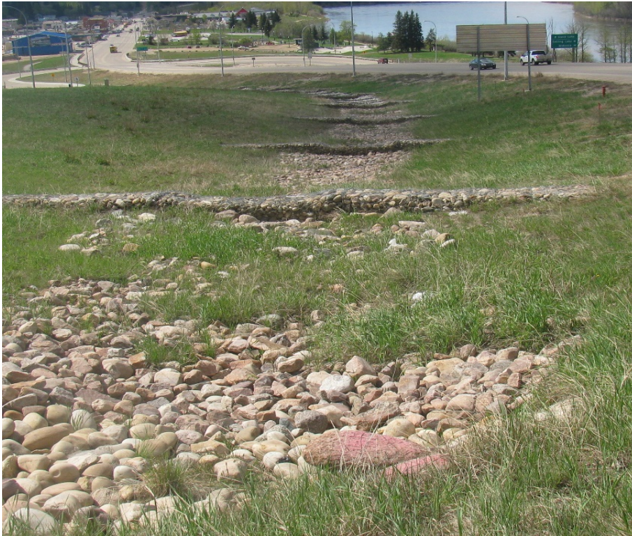
Photo #1. Hwy 55 South Ditch. Looking west at existing riprap channel from the east of G1.
