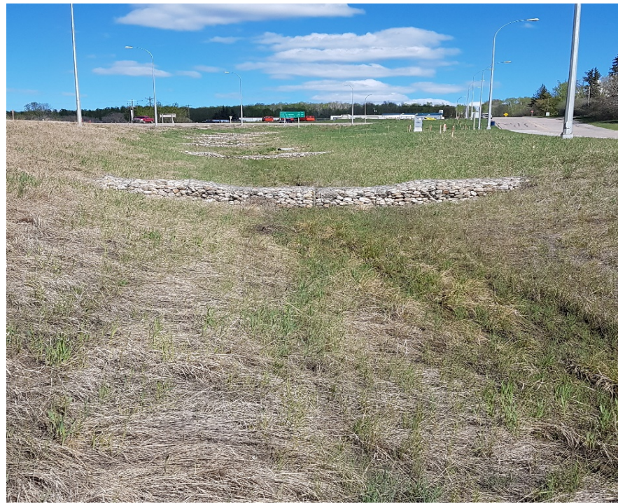
Photo #7. Hwy 55 south ditch: looking east at signs of erosion between G10 and G11
