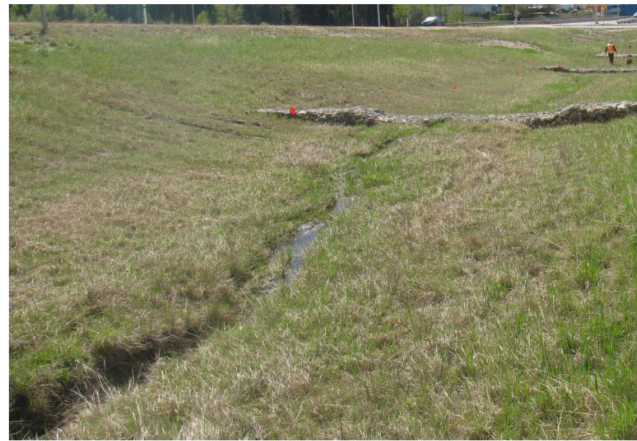
Photo #16. Hwy 55 North Ditch: Erosion gully between G2 and G3
