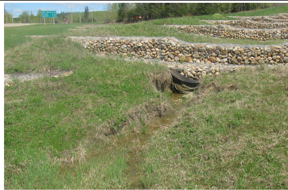
Photo #18. Hwy 55 North Ditch: Erosion gully between G5 and G6; note the gap developed below G6
