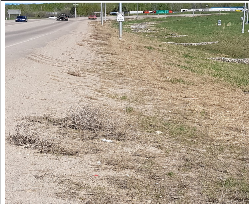
Photo #9. Looking southeast at a bare sandy slope on the south side slope of Hwy 55
