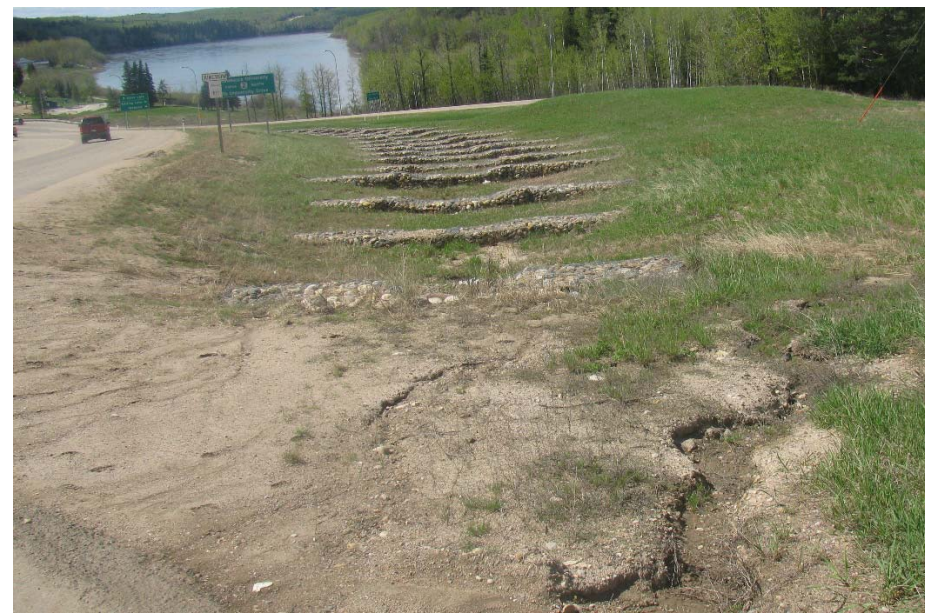
Photo #19. Hwy 55 North Ditch: looking west from the west side slope of 43 Street. Bare ground surface and erosion rills in the side slope
