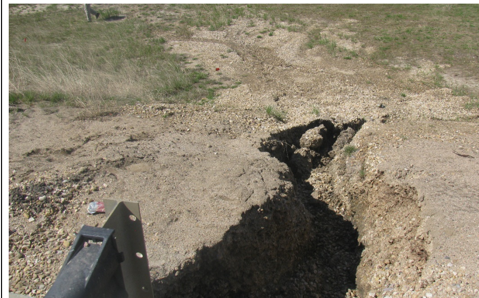
Photo #12. Looking north at deep erosion gullies developed within NE corner of the bridge; erosion gully was backfilled with gravel in 2016
