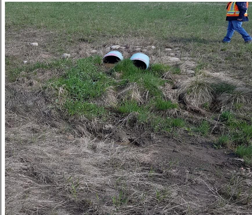
Photo #6. Looking southeast at the outlets of the storm water pipes; signs of erosion near the outlets of the pipes
