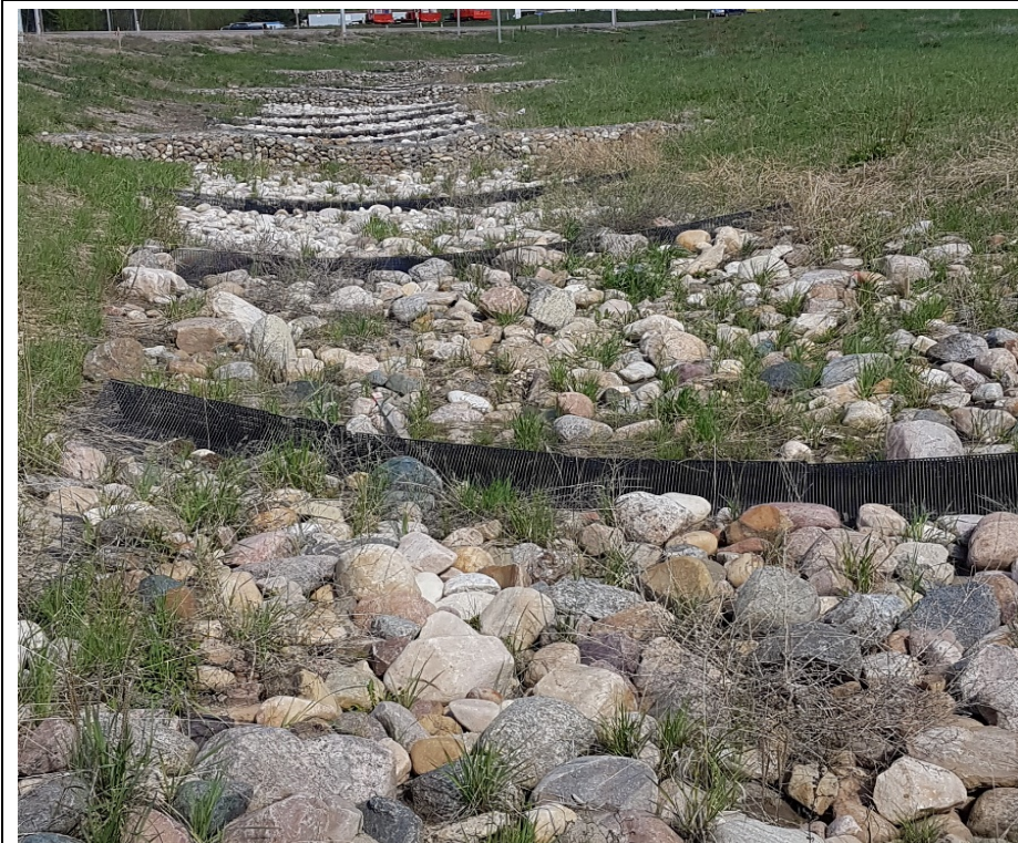
Photo #4. Hwy 55 South Ditch: Looking east at riprap between G9 and G8
