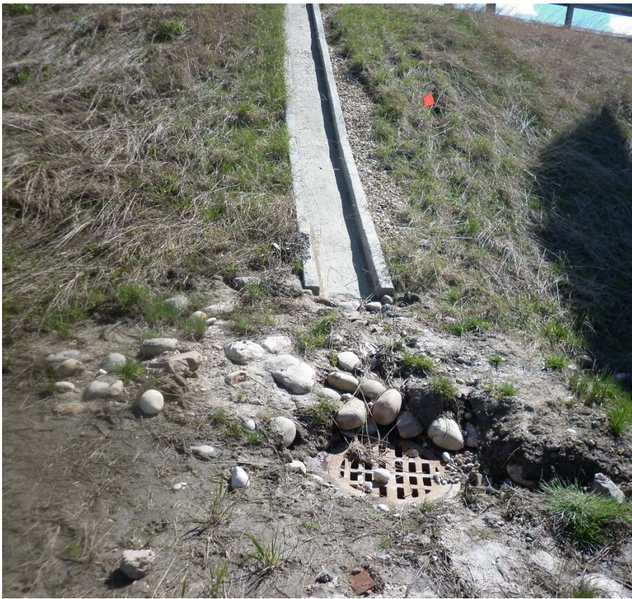
Photo #13. Drain trough on the northwest side of bridge crossing Tawatinaw River. Erosion developed below and on the west facing side the of the drain. Sediment accumulated around catch basin/ dissipation bowl.
