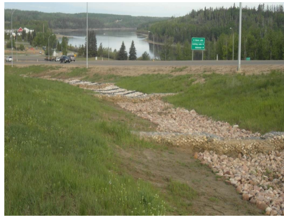
Photo 3. Hwy 55 South Ditch: Looking west at the west end of an existing riprap channel located between G2 and G3. Bare side slope to the south of the channel; the channel needs to be reshaped and riprap should be extended at least 2 m along the side slopes of the ditch
