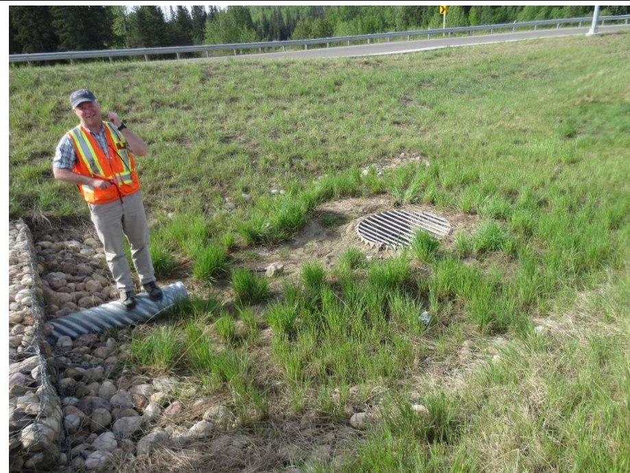
Photo 12. Highway 55 south ditch: Bare ground between the spill block and the Manhole; additional riprap is required at this location
