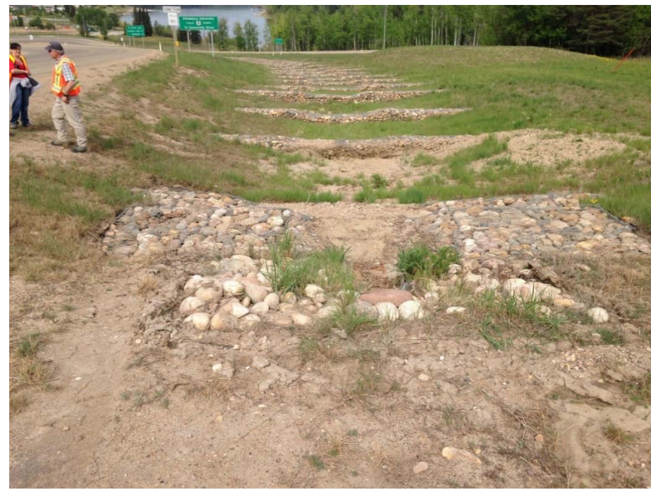
Photo 21. Hwy 55 North Ditch: looking west from the west side slope of 43 Street. Bare ground surface between west side slope of 43 St and G31 and between G30 and G31; sediment accumulated in the ditch behind the gabion baskets; ditch bottom should be cleaned of the built up sediment and riprap should be placed in these areas to reduce future erosion issues.
