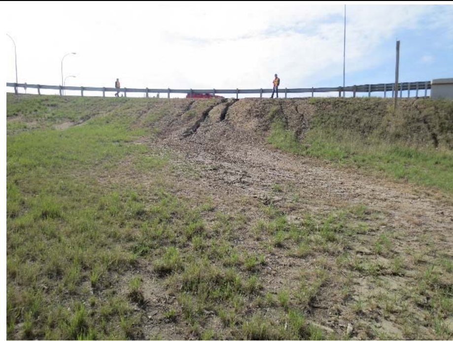
Photo 14. Looking south at deep erosion gullies developed within northwest side slopes of the bridge east approach fill
