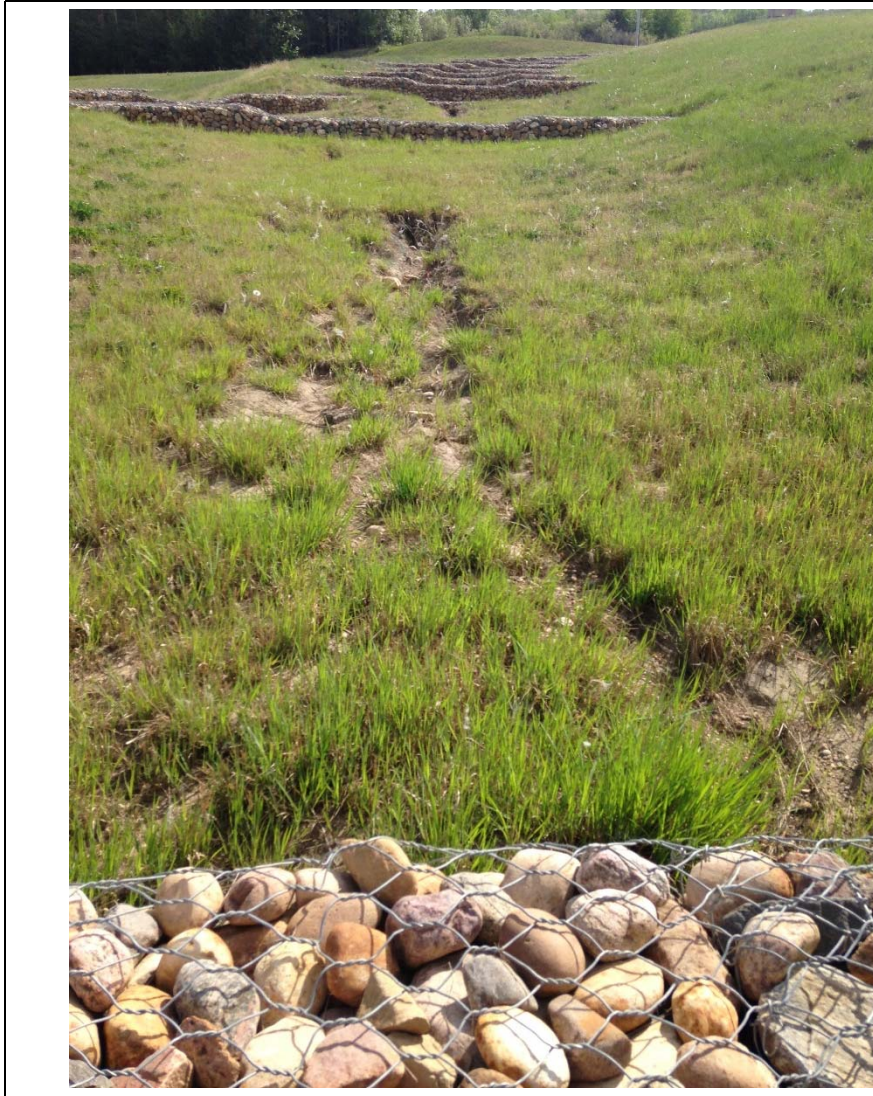
Photo 18. Hwy 55 North Ditch: Erosion gully between G3 and G4
