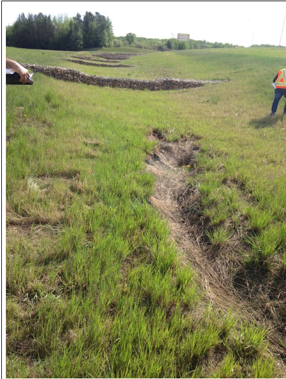
Photo 17. Hwy 55 North Ditch: Erosion gully between G2 and G3
