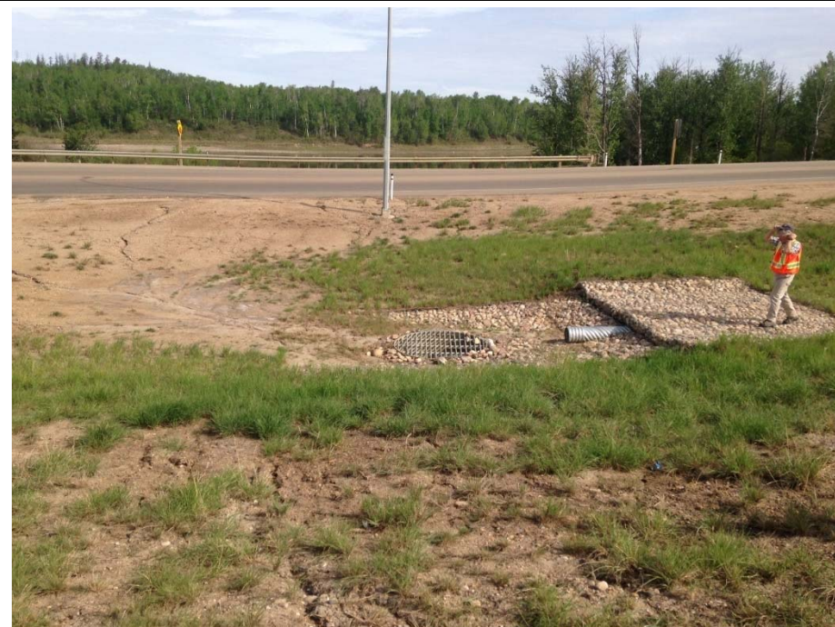
Photo 16. Hwy 55 North Ditch: Looking north at outlet of the Spill containment ditch block CSP pipe; note the presence of erosion rills and bare vegetation in the slopes; additional riprap should be placed between the CSP pipe and the manhole
