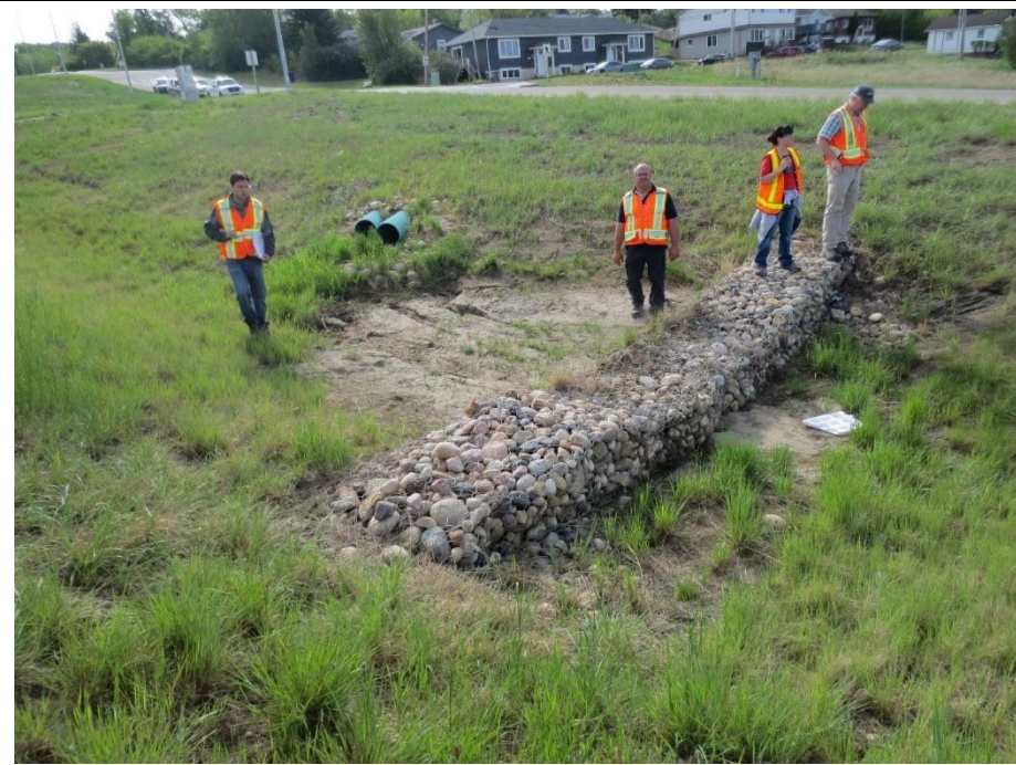
Photo 8. Looking southeast at G10 and the outlets of the storm water pipes; note the absence of vegetation in this area and signs of erosion at the outlets of the pipes
