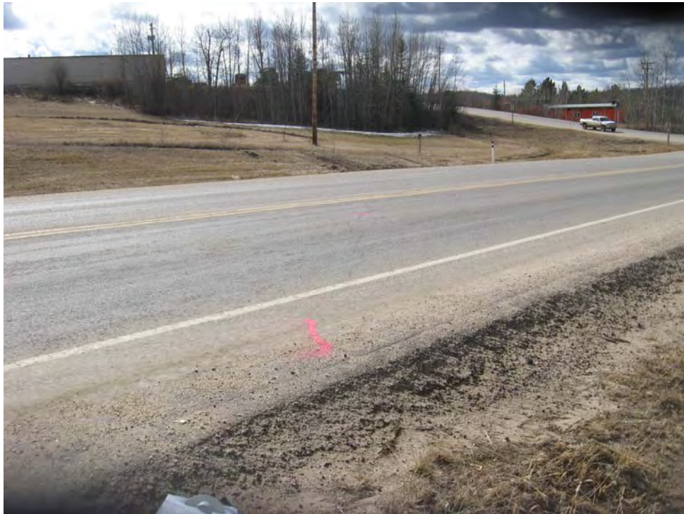
Photo 5 – Looking south at Crack A from the north ditch
