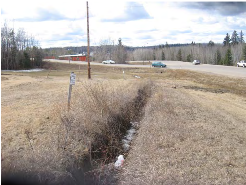
Photo 6 – Looking west at the catch water ditch at the top of the backslope
