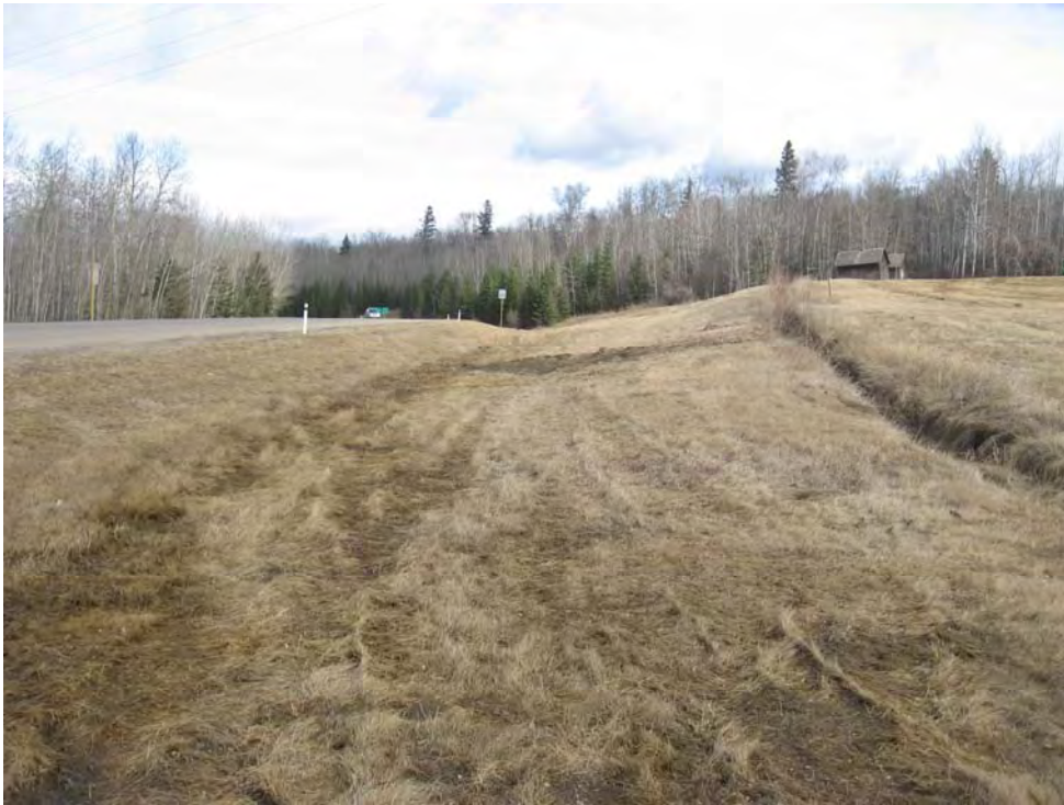
Photo 8 – Multiple wet spots in the south highway ditch- Looking east
