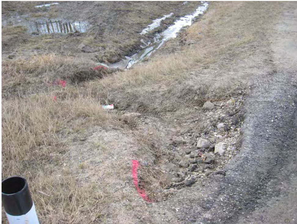
Photo 9 – Looking at ponded water at the outlet of the CSP culvert and erosion in the vicinity of the culvert
