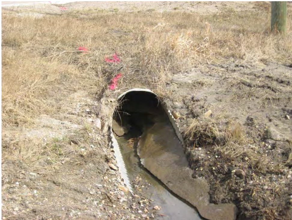
Photo 10 – Closer look at the culvert outlet. Note the cracks formed to the left of the culvert and formation of ice inside the culvert
