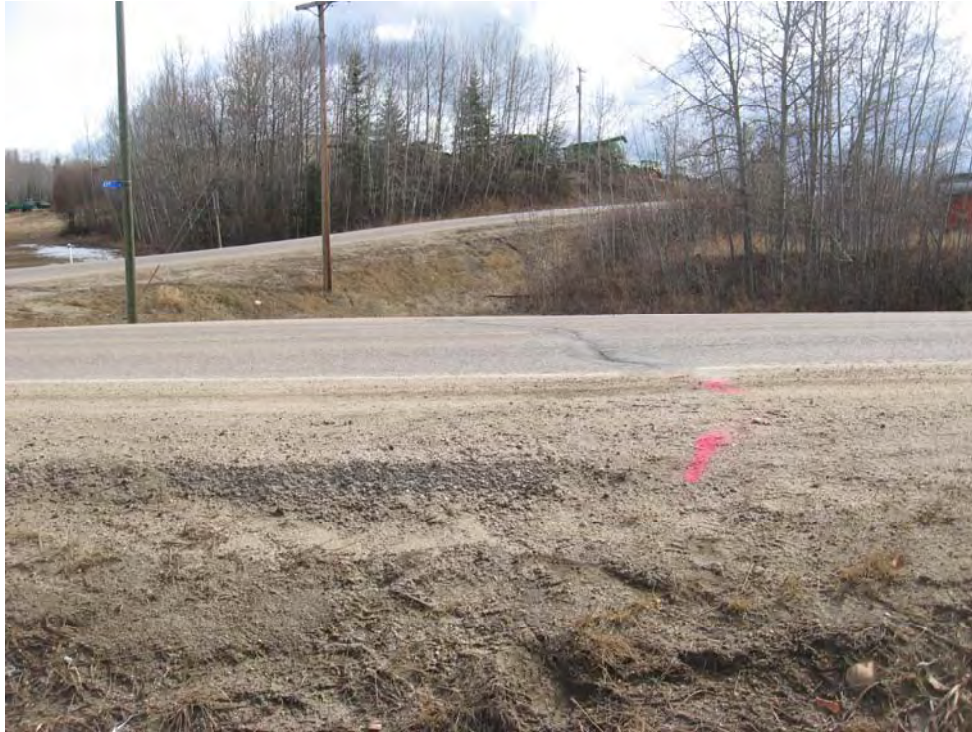
Photo 11 –Crack E at the west side of the site- Looking south from the north ditch
