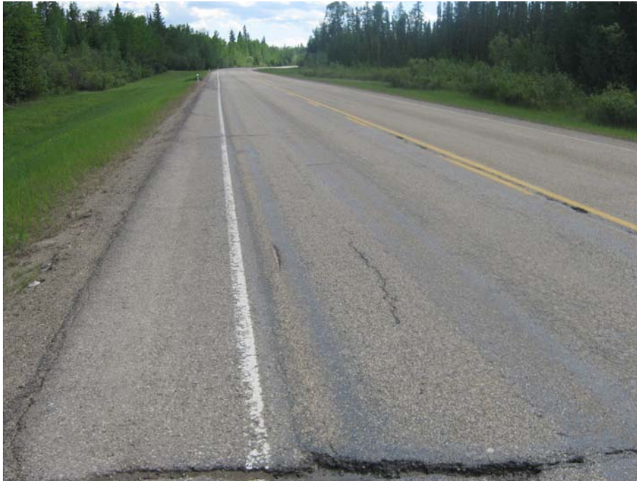
Photo#1 Looking south at a longitudinal crack in the highway NBL surface west of the landslide
