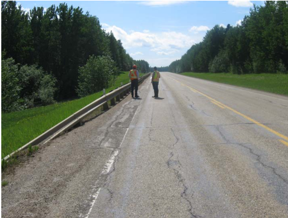
Photo#1 Looking southeast from the north side of the site at longitudinal cracks in the highway NBL
