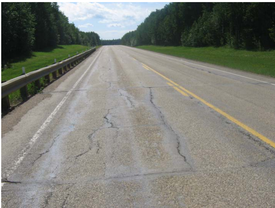
Photo#2 Looking southeast at an additional set of longitudinal cracks in the highway NBL
