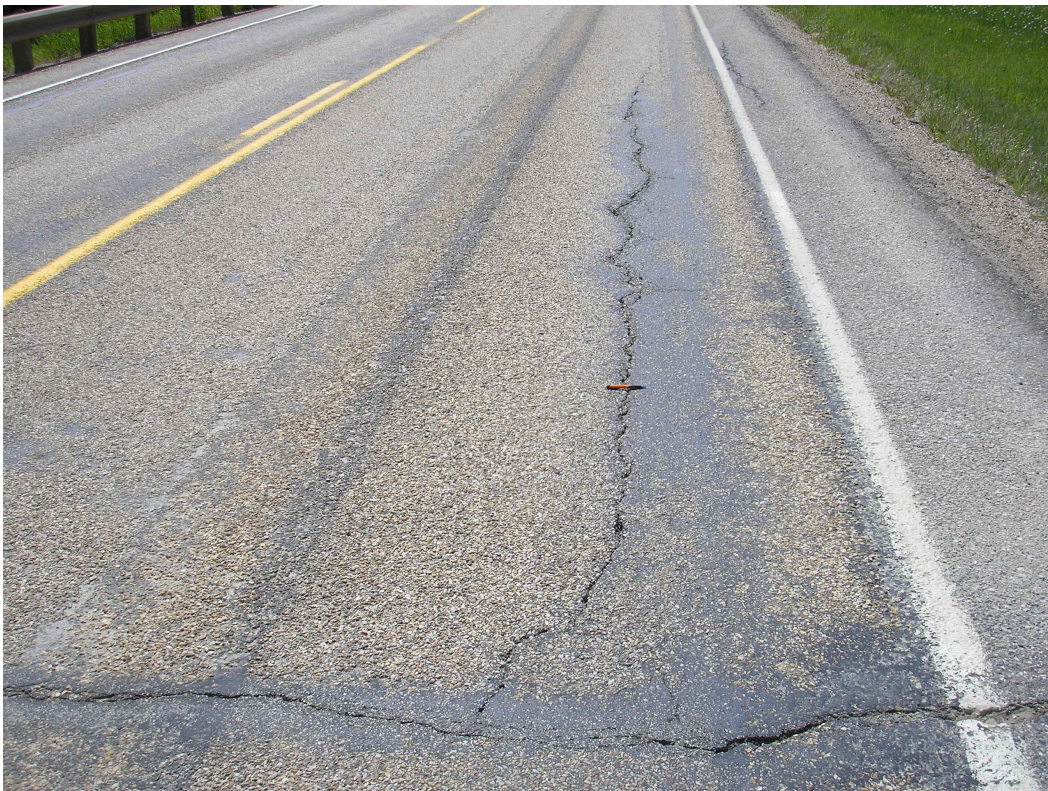
Photo #2 Looking south toward an open longitudinal crack on the highway SBL
