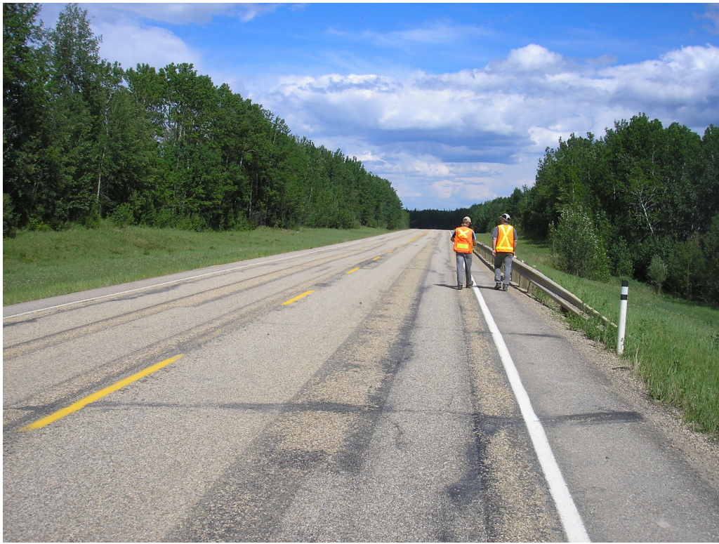
Photo #1 General view of highway surface at slide location, looking north
