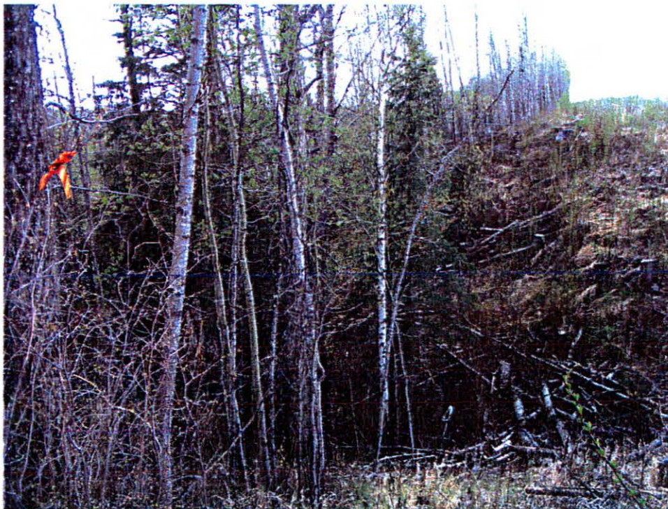
Photo 1 & 2 -Looking at the Gully at km 10.4, May 24, 2007.
