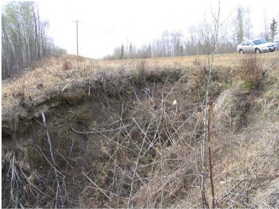
Photo 3 & 4 Looking at the Gully at km 10.2, May 2, 2006.
