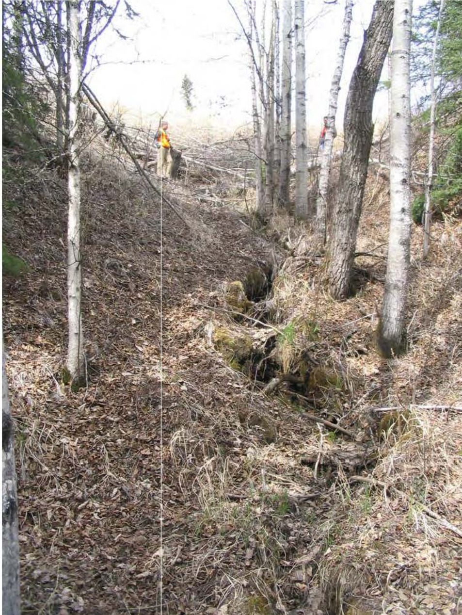
Photo 7 Looking at the Gully at km 10.45, May 2, 2006.
