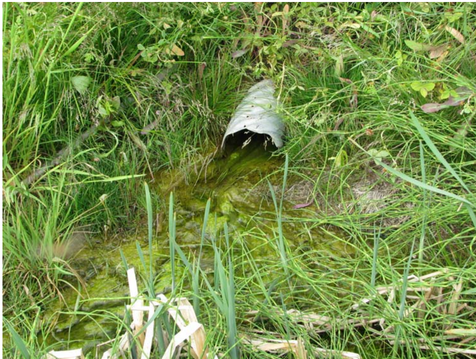
Photo 6 - Seepage from the subdrain of the South Slump repair (July 8, 2008).
