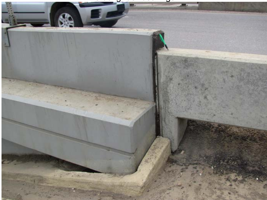
Photo #6 Looking southwest at the concrete barrier; the concrete barrier dropped by about 160 mm
