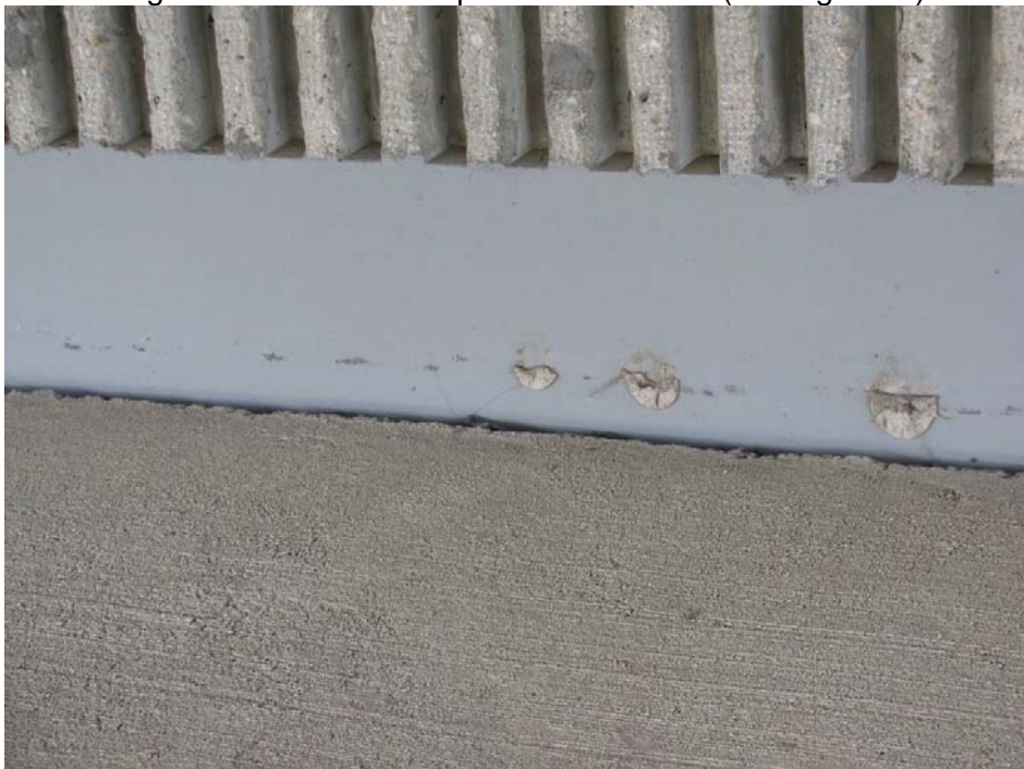
Photo #4 Settlement of west headslope concrete facing. Note the dents on abutment wall seat (looking west)
