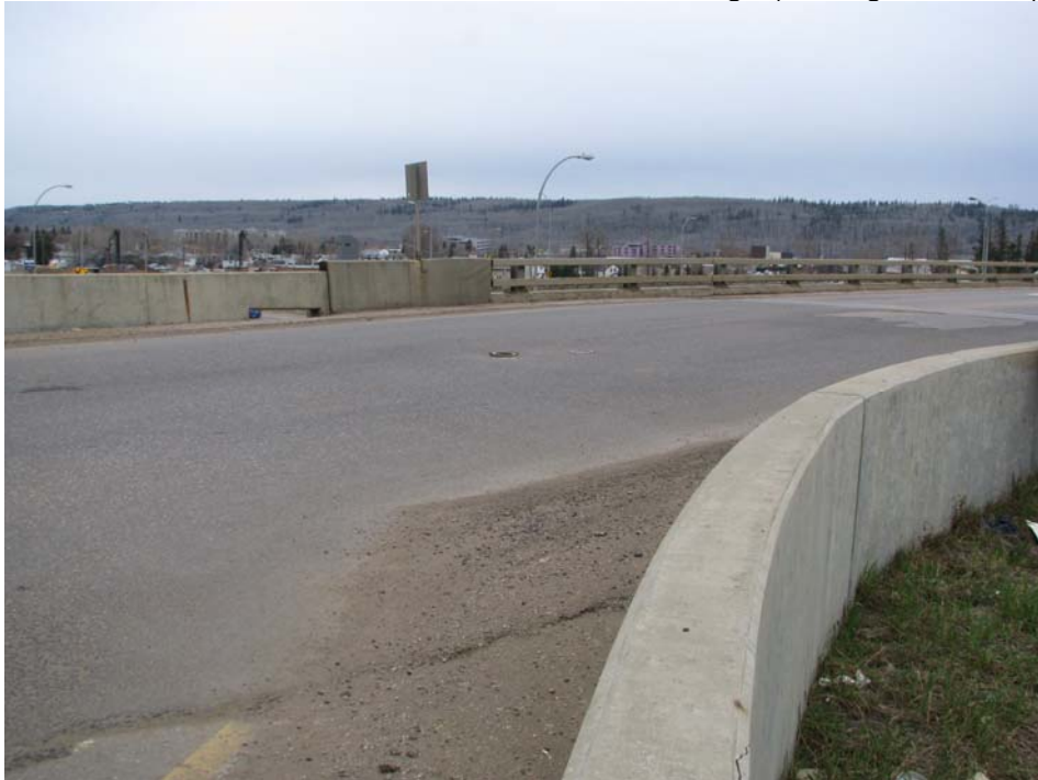
Photo #2 ACP overlay placed on the top of the bridge (looking north east from top of west head slope)
