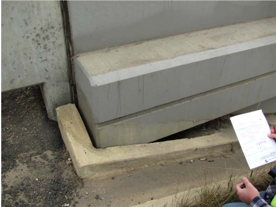
Photo #3 Settlement of bridge curb drain; the change in color of the side barrier signifies the original location of drain prior to settlement (looking north)
