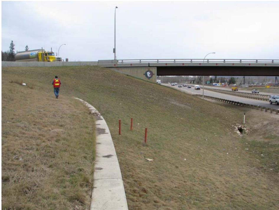
Photo #1 General view of the west side of the bridge (looking northwest)
