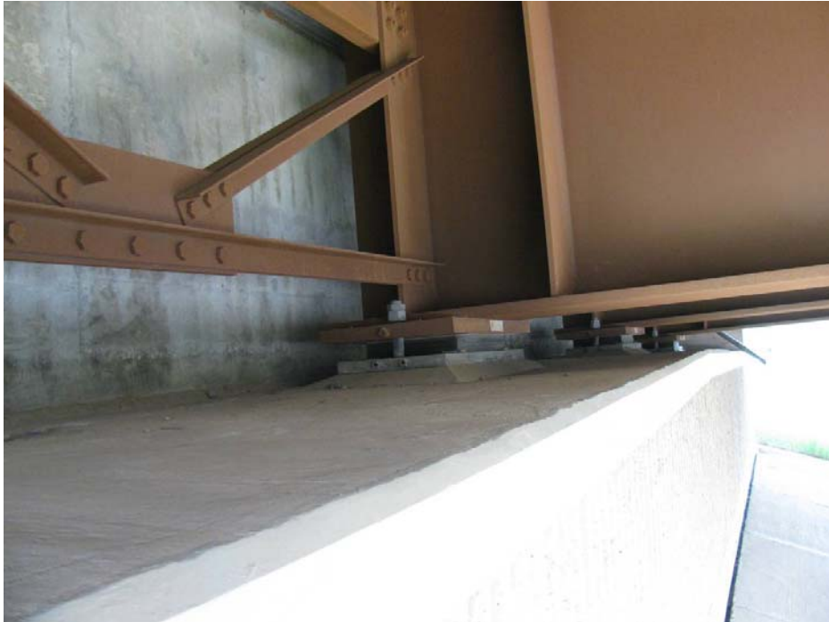
Photo #5 Looking northwest at the bridge girder bearings; no signs of distortion in the steel girder bearings
