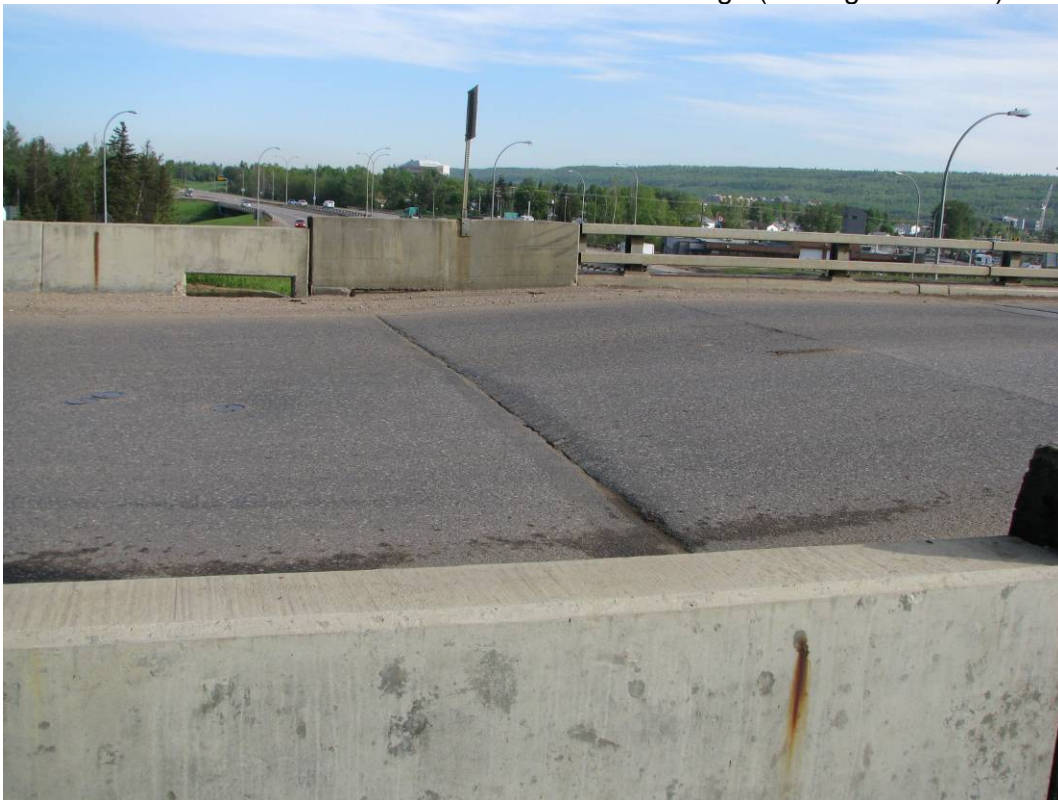
Photo #2 Dip along the bridge top surface over a distance of 4 m. (looking north from top of west head slope)
