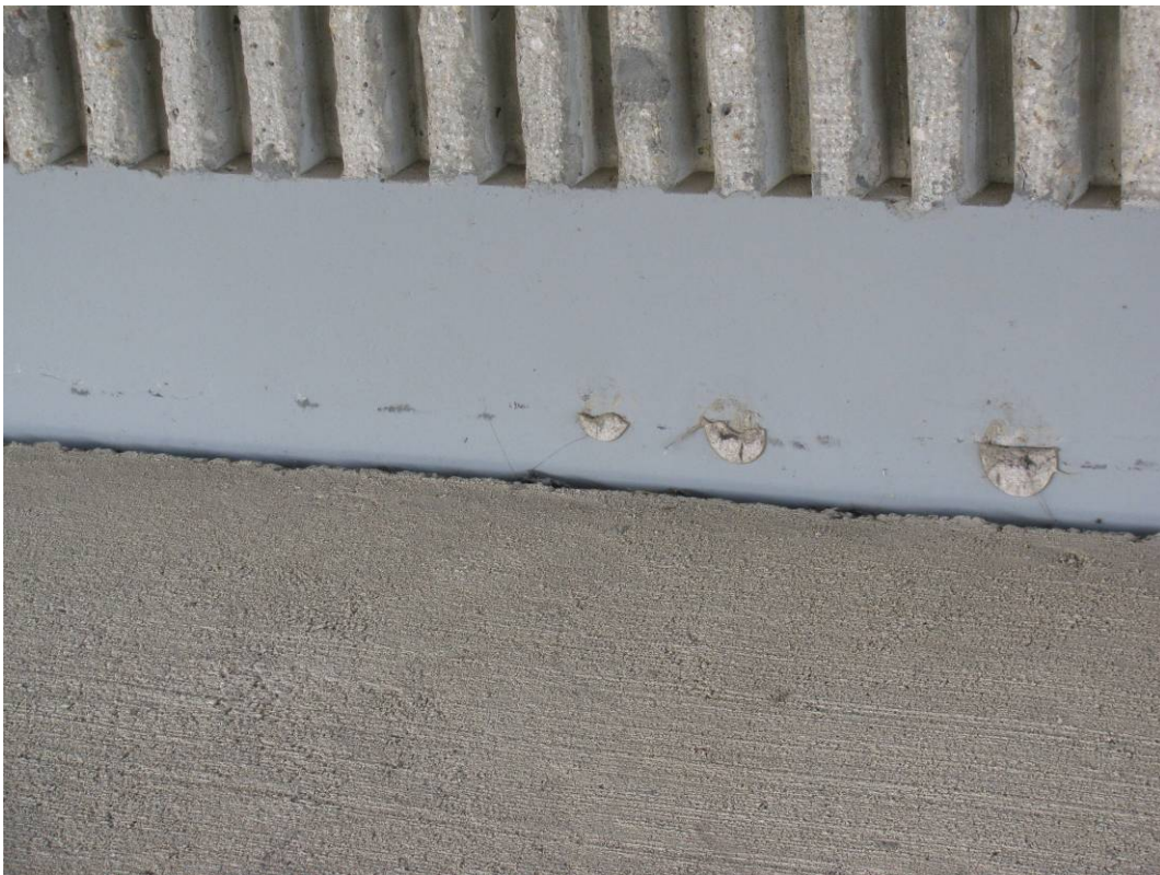
Photo #4 Settlement of west headslope concrete facing. Note the dents on abutment wall seat (looking west)
