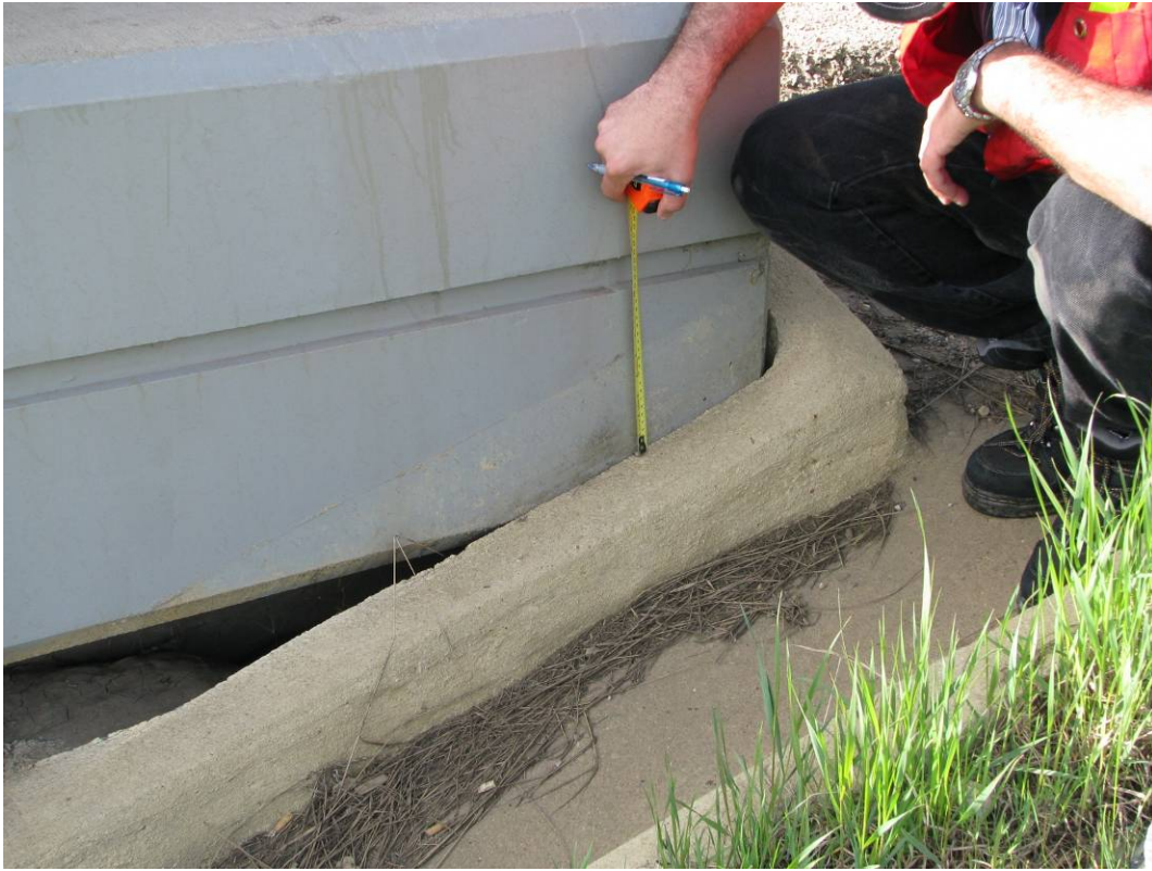
Photo #3 Settlement of bridge curb drain. Note that the dents in the side barrier are probably signifying original location of drain prior to settlement (looking south)
