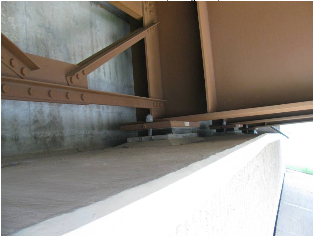
Photo #6 Looking northwest at the bridge girder bearings; no signs of distortion in the steel girder bearings
