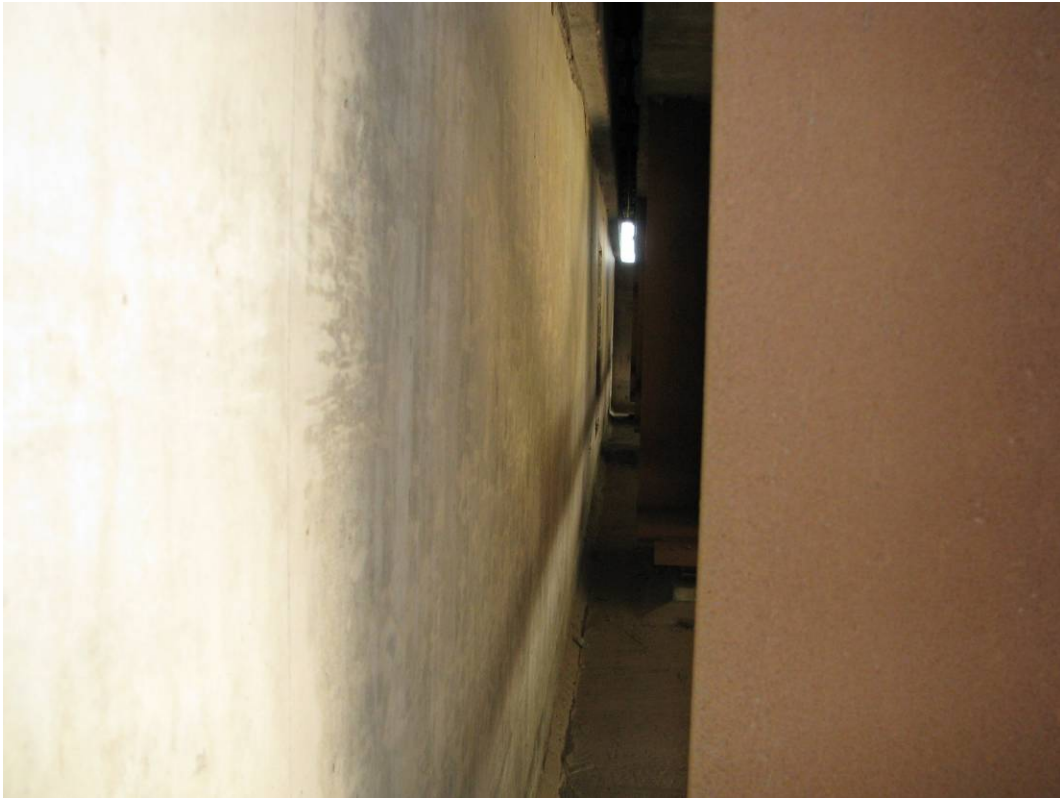
Photo #5 Looking along the west abutment wall face. No signs of abutment wall cracking/bulging. The clear space varied between the abutment wall face and girder ends from 180-200 mm (looking north)
