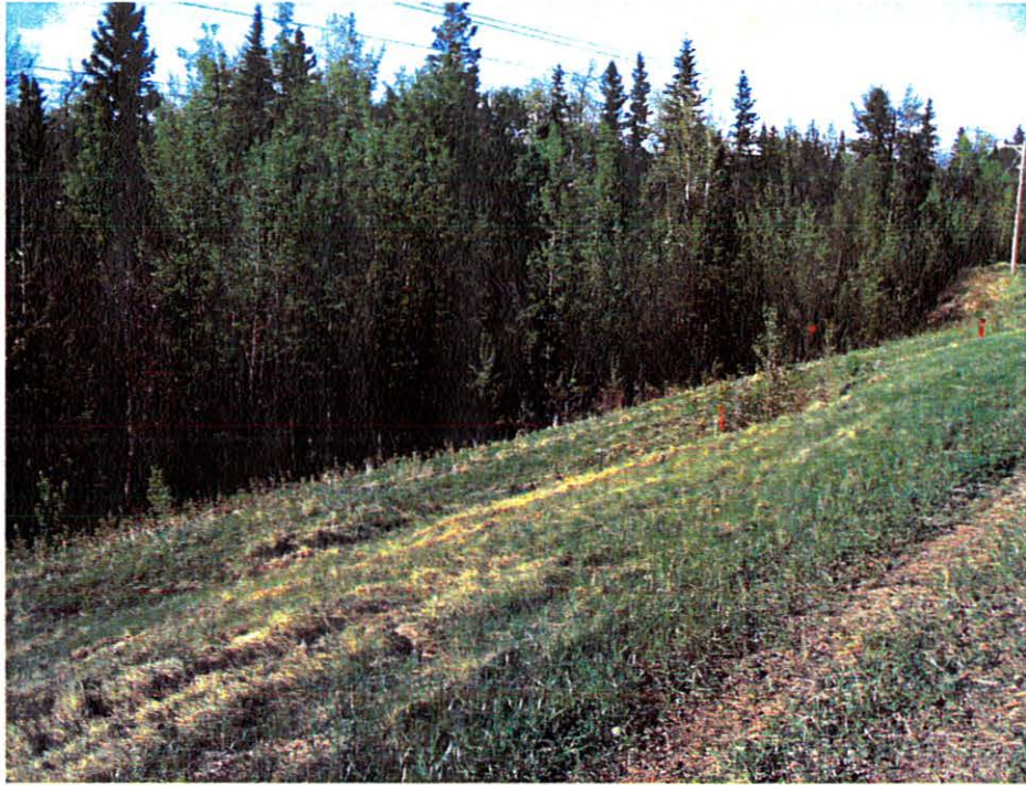
Photo 3 - Looking north at the distress area, May 24, 2007.
