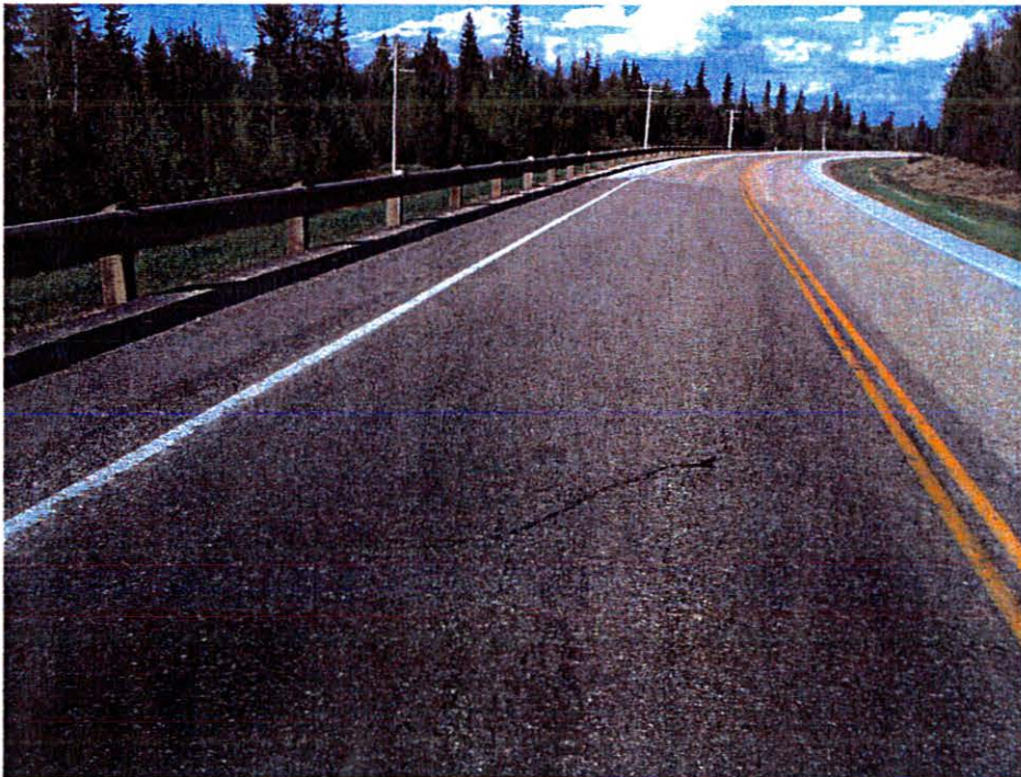
Photo 2 - Transverse crack through the patched area, May 24, 2007.
