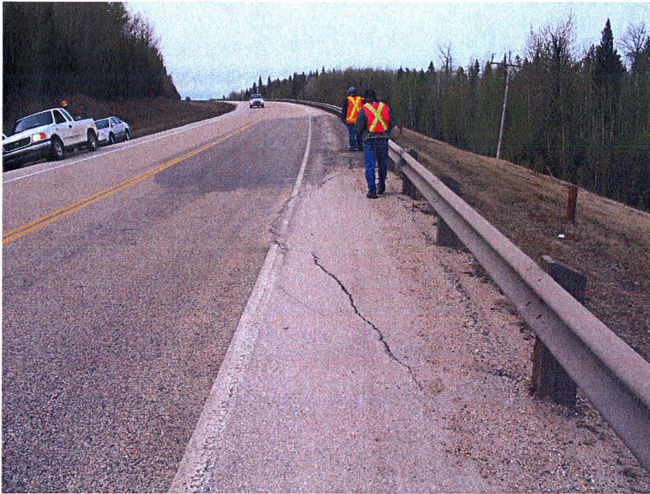
Photo 3 Looking West along Highway at cracks, May 2, 2006.
