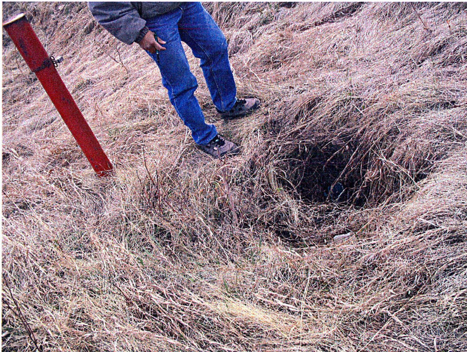
Photo 4 Hole around SI#5 location, May 2, 2006.
