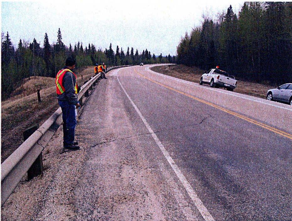
Photo 2 Transverse crack through the patched area, May 2, 2006.
