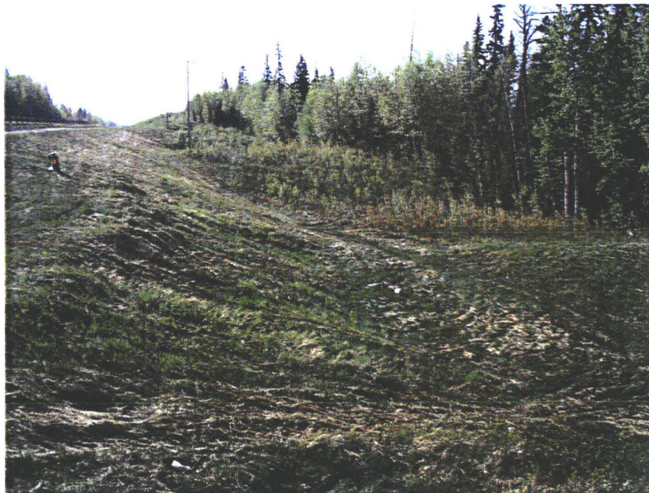
Photo 2 - Looking at the downslope toe area, May 24, 2007.
