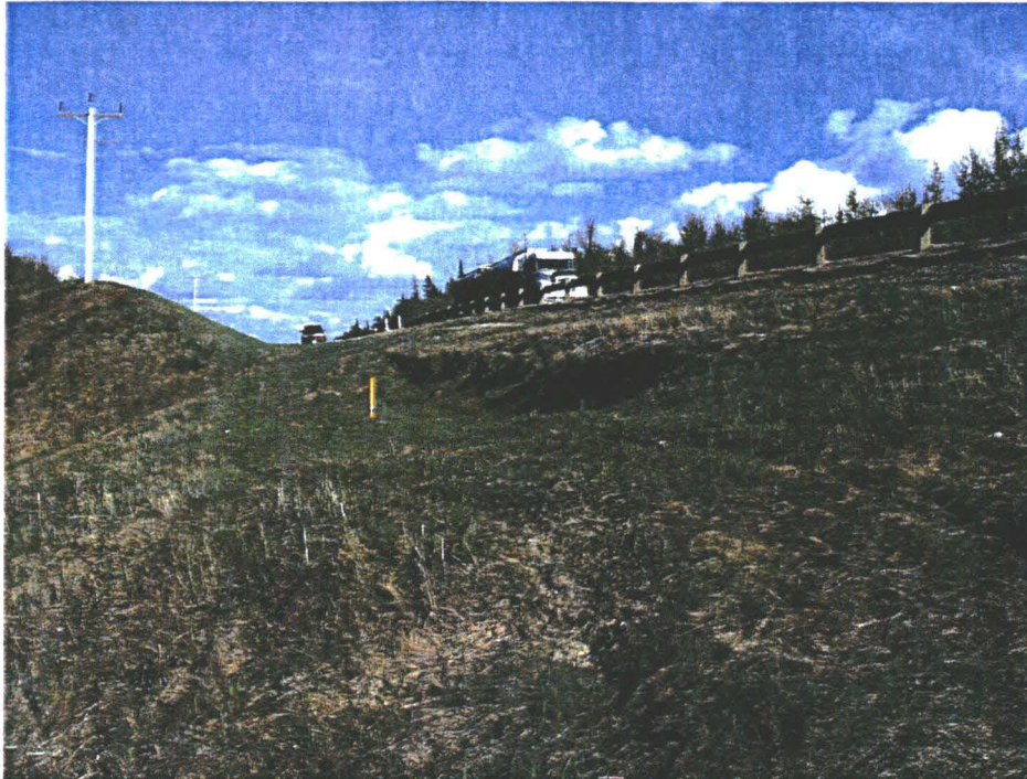
Photo 3 -Looking east at the distress area, May 24, 2007.
