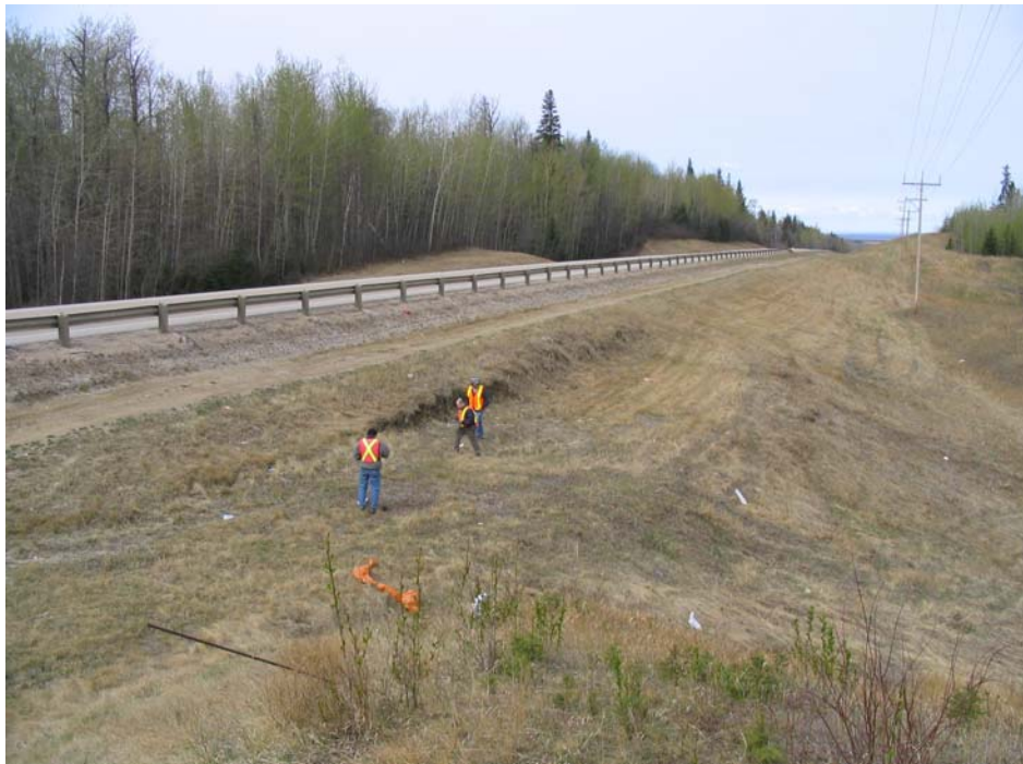
Photo 2 Looking from top at the distress area, May 2, 2006.
