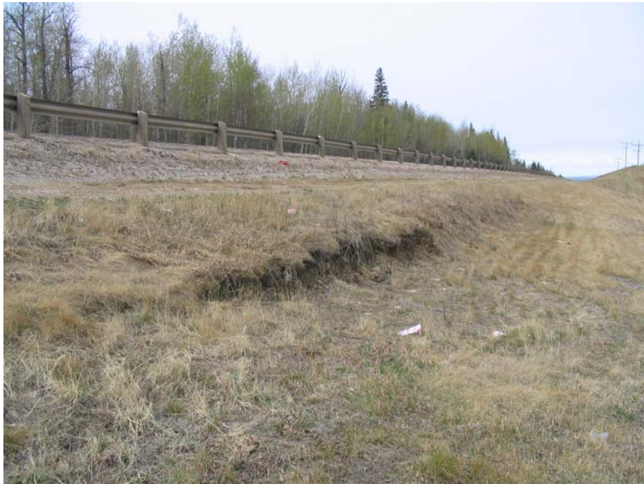
Photo 1 Looking northwest at the distress area, May 2, 2006.
