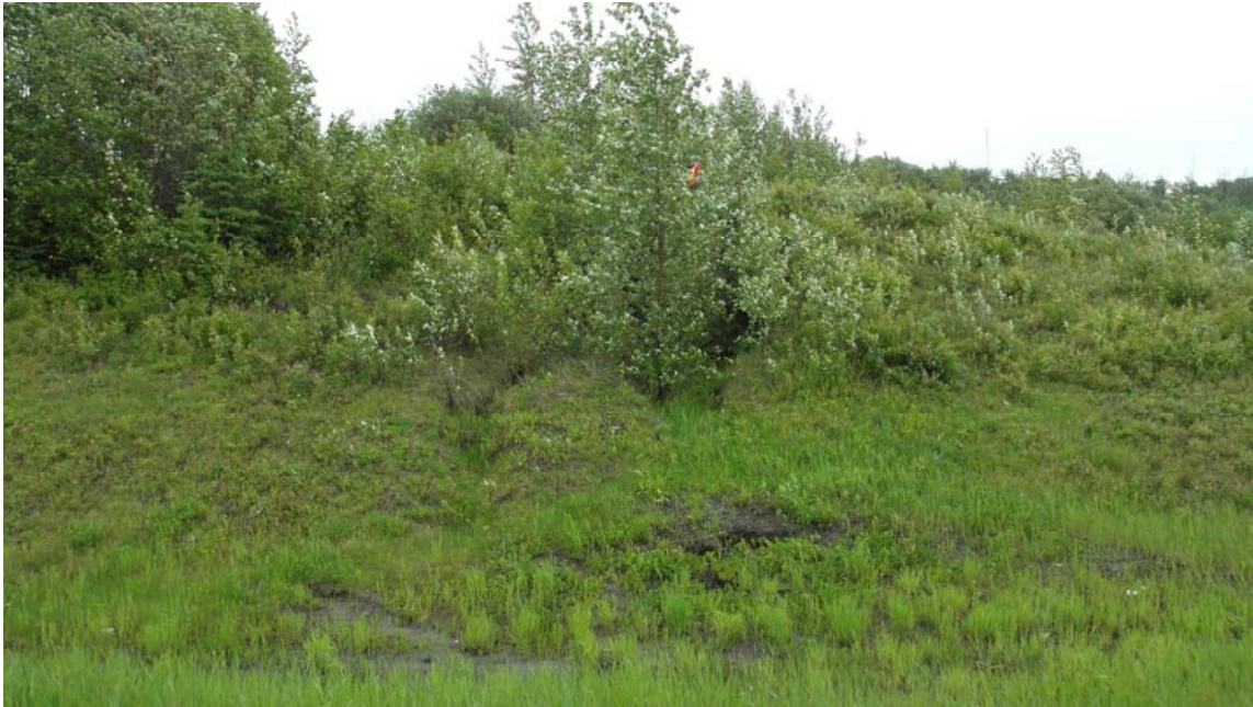
Photo# 1 General view of highway backslope slump; note that vegetation has grown within the slump mass (looking south)
