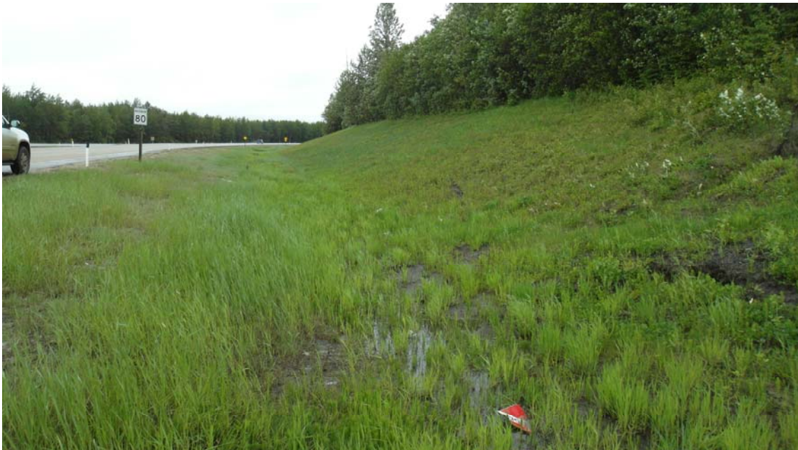
Photo# 2 Highway surface and side slope at the slump location, looking east; slight amount of water ponding in the ditch
