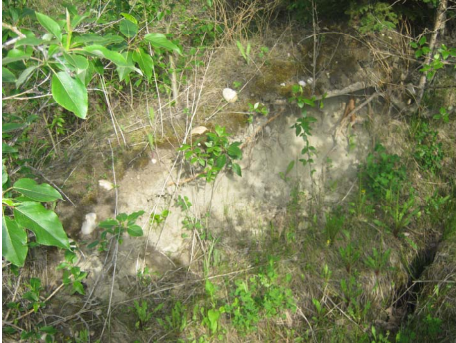
Photo# 3 Looking east at the west facing crack; the exposed face of the crack consists of fine silty sand
