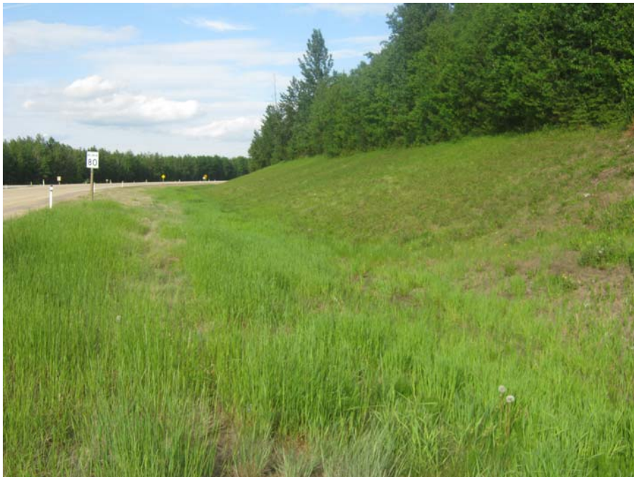
Photo# 2 Highway surface and side slope at the slump location, looking east
