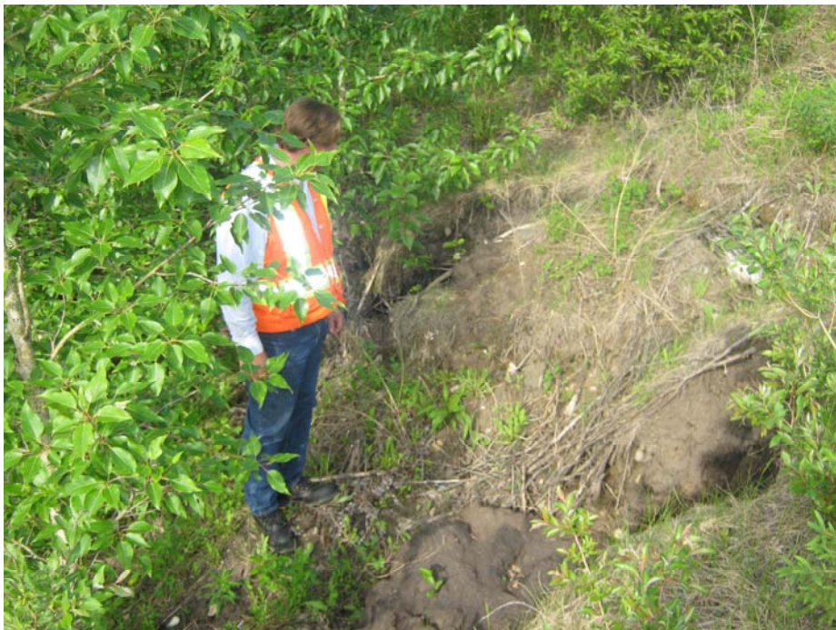
Photo# 4 Looking east at the slump cracks near the crest of the slope; note further movement of headscarp cracks
