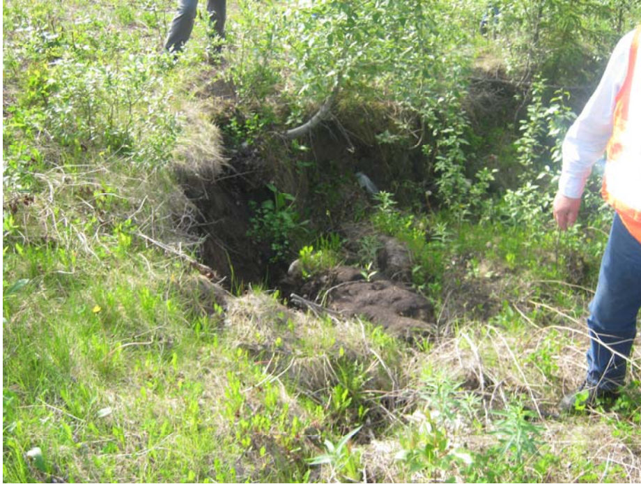
Photo# 5 Looking northwest at the slump cracks near the crest of the slope; note the retrogression of the scarp cracks
