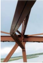
High Load Impact Damage
