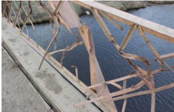
90% failure of diagonal - wide load impact damage
