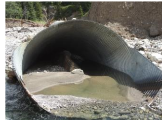
BF 77496 – Outlet and barrel floor folded and heaved nearly to roof
