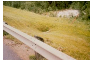
Hole in side slope of D/S side
