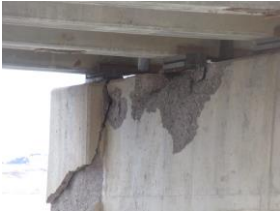
BF 1153 – Failed concrete at west end of P1 from frozen bearings under G1, G2. G2dbreck
