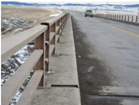
BF 1153 – 30mm drop in rail and curb over Sp.1-G1.
