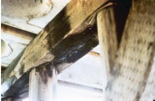
Bottom of cap with piling punching (North pier)
