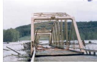
Bridge starting to move laterally
