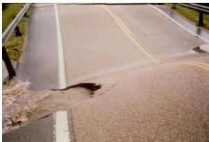
Water on U/S end up to shoulder of road
