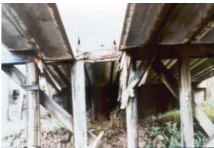
Failed pier cap
