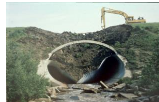
Total collapse of culvert. Only headwall intact
