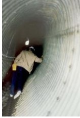
Inside collapsed culvert
