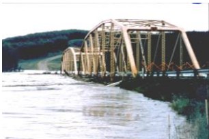
Truss partly under water
