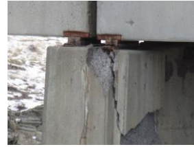
BF 1153 – Failed pier concrete and un-supported bearing under Sp. 1-G1.
