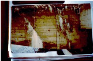
Shear crack in girder and efflorescence from cracks
