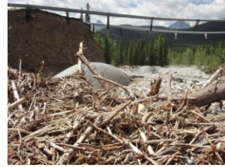
BF 77496 – Drift blockage across inlet and heaved barrel.
