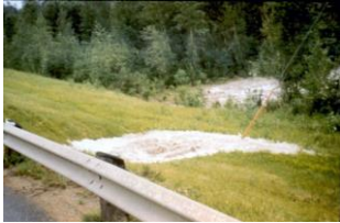
Water now coming out of D/S fill
