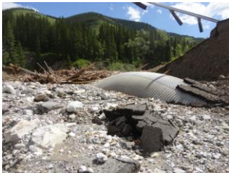
BF 77496 – Inlet blockage and barrel heave
