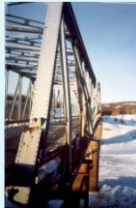
Broken hanger U7 - L7 and first diagonal U7 - L6
