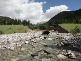
BF 77496 – Looking D/S at scale of washout (30m wide vs. 4.3M pipe).
