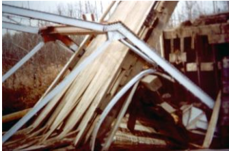
Abutment end of truss dropped and buckled the bottom chord
