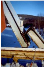
Severed batter post U7 - L8
