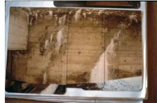
Shear crack at girder end
