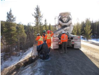
Grout / transit mix installed through holes cut into roof of original pipe.
