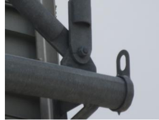
Crack in Vertical at Bolt Hole
