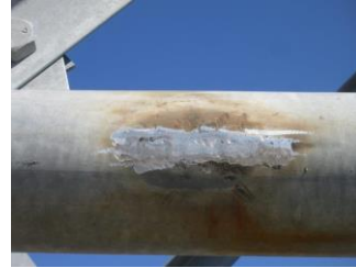
Crack in Bottom Chord – Weld Repair
