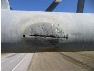
Crack in Bottom Chord – Stop Drilled
