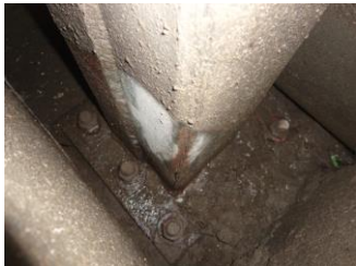
Crack in Column Plate Weld
