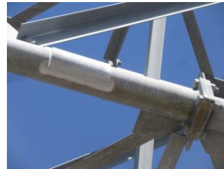
Crack in Bottom Chord – Steel Sleeve
