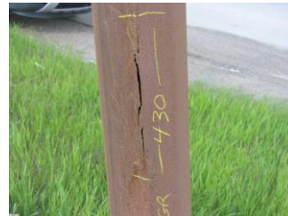
Crack in Column of COR10
