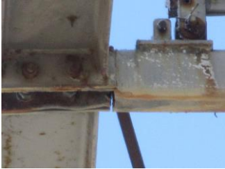
Crack in Access Platform Support
