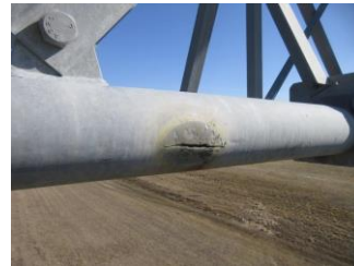
Crack in Bottom Chord
