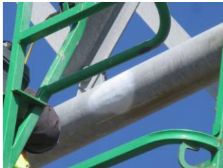
Crack in Bottom Chord – Metallized
