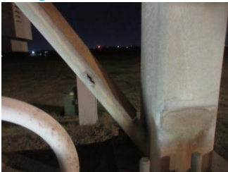
Crack in Diagonal
