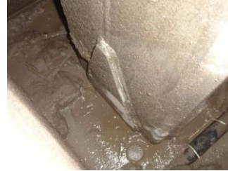
Crack in Column Plate Weld
