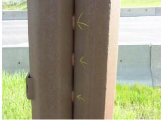
Cracks in Column Joint Welds of COR10
