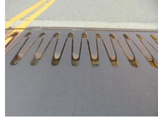
Finger Plate Joint with Broken/Lifted Fingers Welds
