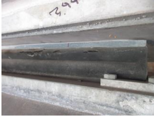
Torn Neoprene Pad Bearing
