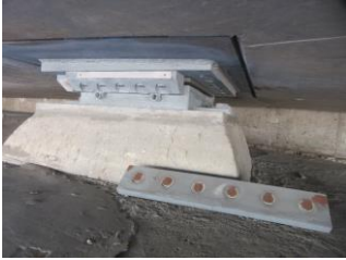
Pot Bearing – Failed Keeper Plate
