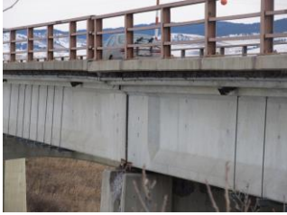
Failed Sliding Plate with Self-Lubricating Bronze Plate Bearing
