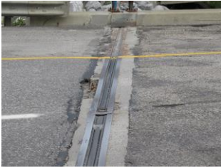
Missing Plow Guards and Spalled Paving Lip
