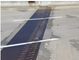
Finger Plate Joint with Broken/Missing Fingers
