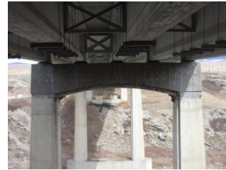
Failed Self-Lubricating Bearing Replaced with Neoprene Pad Bearings
