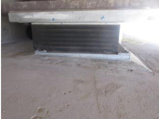
Displaced Neoprene Pad - Over Keepers
