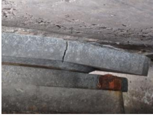
Pot Bearing – Cracked
