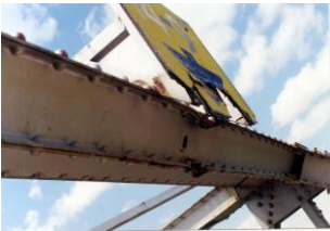
Portal U7EU7W is damaged with two 50 mm notches and broken clearance sign.
