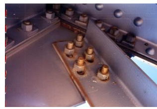
Span 2, top chord bracing U3N-U3S have slotted holes at U3N
