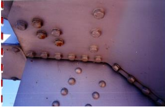
Span 2, at U9N, there are six loose bolts
