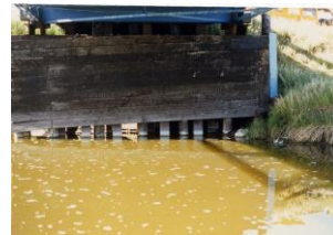
Timber planks missing at South pier
