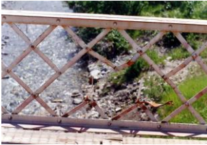
Lattice rail damaged at L1S
