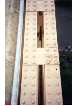
Outside top chord U4USN is missing 3 bolts
