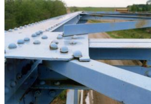
Top chord bracing U3S-U4N has broken gusset at U3S
