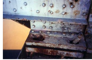
Sp. 1- Pier #2 bearing over expanded by 125 mm & bent anchor bolt
