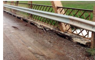
Damaged wheel guard at SE corner
