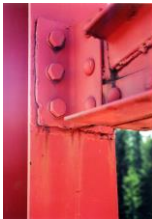
Modified sway brace connections were welded to the verticals, and then the welds were removed and bolt fasteners installed.
