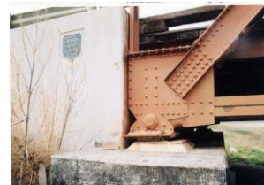
South abut. bearings are over expanded, neoprene pads are at the edges of masonry plates. Trusses are against the backwall.
