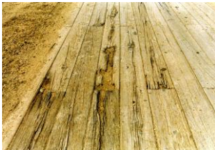
Dirty strip deck with broken & worn planks
