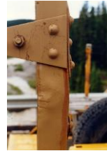
Vertical U4-L4N at m5 strut connection is buckled and has notches
