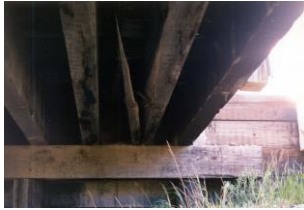
Broken stringer second from U/S East approach
