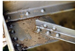
Bottom sway bracing L1S-L2N is cracked at L1/S. Note corrosion section loss.
