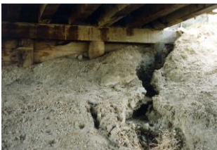
Erosion at West abutment
