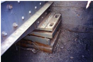
Abut. #1 bearing over expanded by 60 mm, twisted 25 mm and broken anchor bolt
