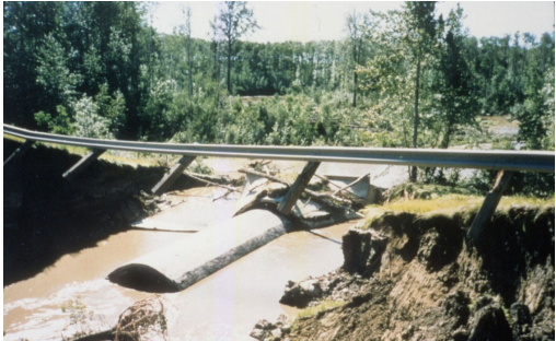
Arch culvert after high water in July.
