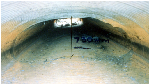
Arch shaped CSP with heaved floor and deflecting roof.
