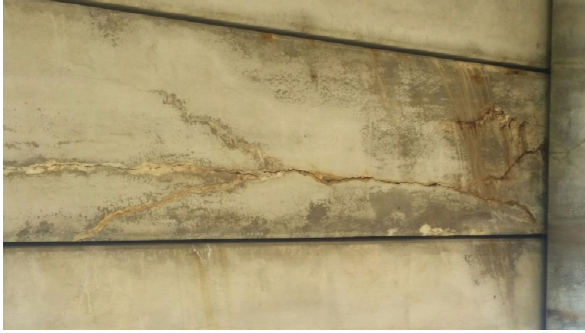
Corrosion cracking on pre-stressed girder underside
