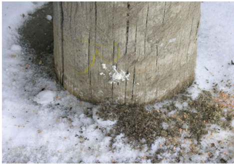
Timber Pile with Rot – Rated 3
