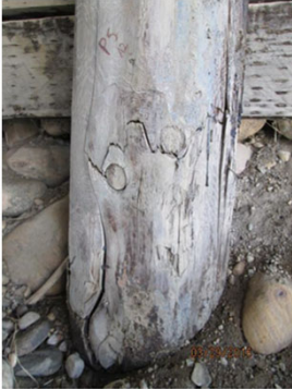
Timber Pile Horizontal Bending Crack – Rated 3
