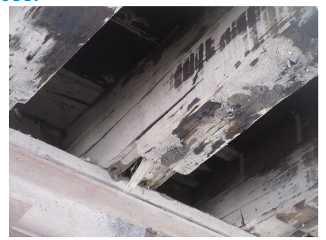
Rotted subdeck & rotted/cracked timber stringer. Both rated 3 or less.
