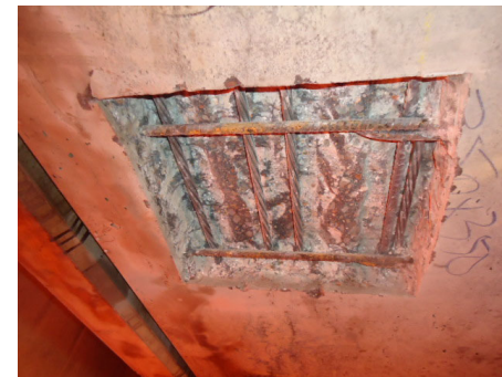
Partial depth repair of prestressed box girder. Note location of strand inside of rebar.
