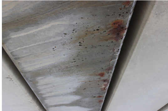
Wide longitudinal crack, with corrosion. Rated 2
