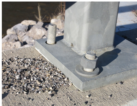
Missing anchor bolt nut – Rated 3
