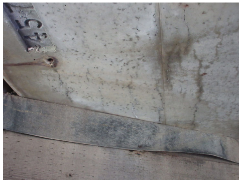
Narrow longitudinal crack with no corrosion. Rated 5
