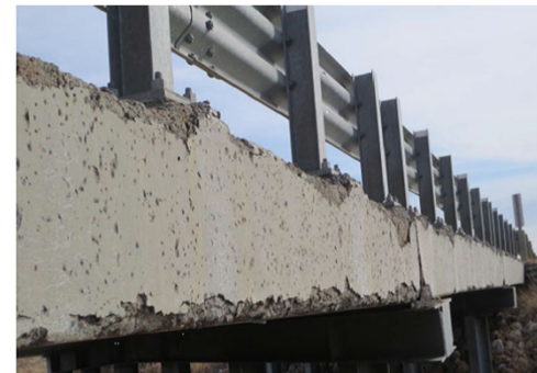
SC Girder Deterioration Affecting Post Anchorage – Post Rated 2.
