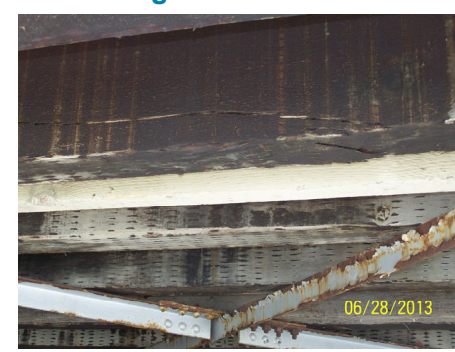
Cracked Timber Stringer – Rated 3
