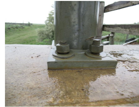
Loose anchor bolt nuts – Rated 4
