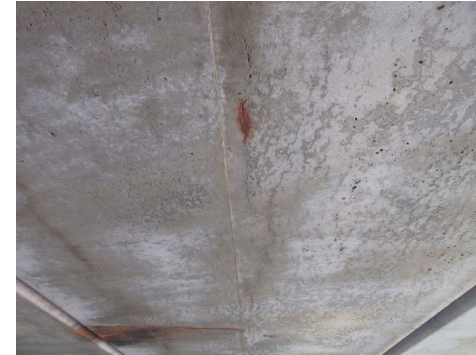
Narrow longitudinal crack with corrosion. Rated 4
