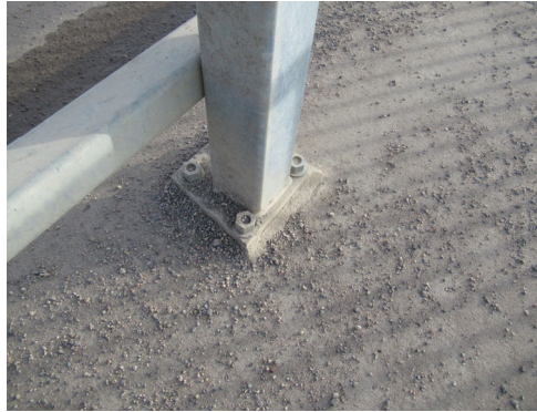
Anchor bolts - insufficient thread projection above nut – Rated 4
