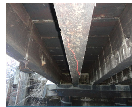
Cracked Timber Stringer –Rated 3
