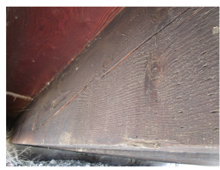
Cracked Timber Stringer – Rated 3
