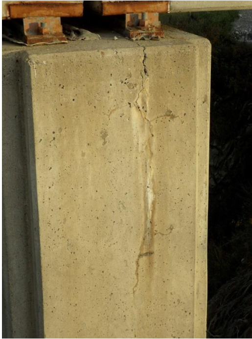
Figure 4: Wide crack in concrete cap at expansion bearing with staining.
