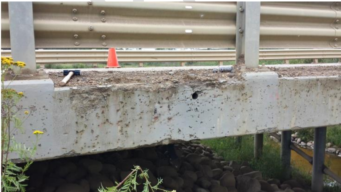
Example 2: Section loss along top and bottom corners of exterior girder. Girder rated 3. Bridgerail posts rated 3.
