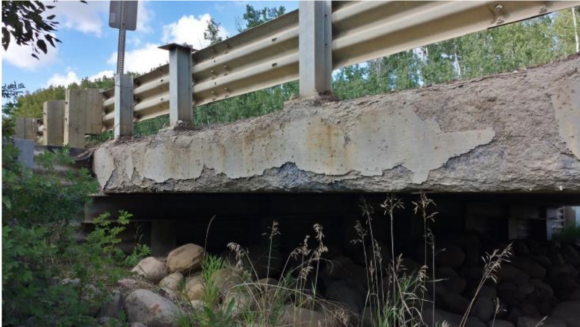
Example 1: Extensive scaling of exterior girder surfaces with section loss along top and bottom corners, but not extending up to the edge of the bridgerail post base plate. No exposed steel stirrups or prestressing strand. Concrete section loss of bridgerail post plinth. Girder rated 3. Bridgerail posts rated 3.
