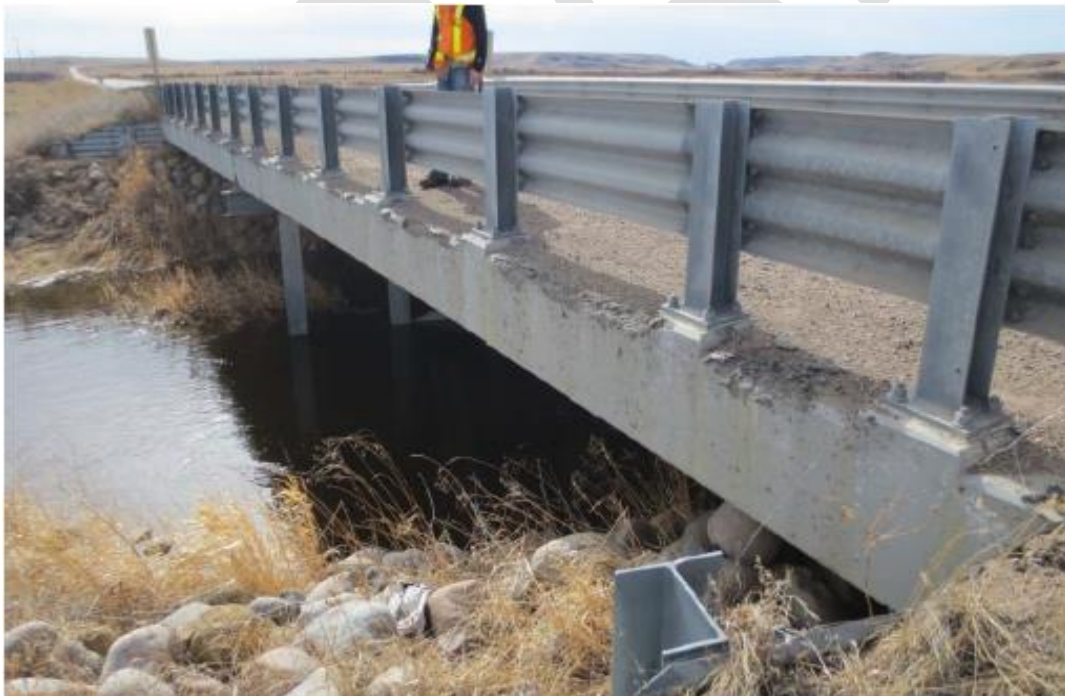
Example 6: Section loss at the top corner of exterior girder that does not extend to the edge of the bridge rail post base plate. Aggregate popouts on exterior face of girder. Concrete section loss of bridge rail post plinth. Girder rated 3. Bridge rail post rated 3.
