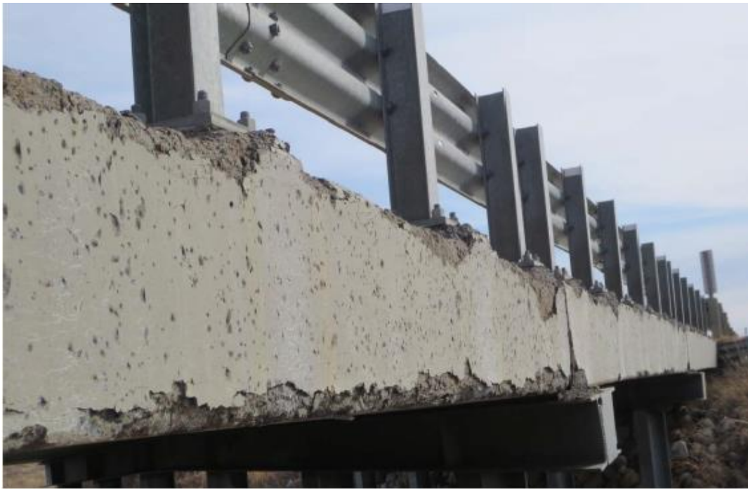
Example 5: Scaling of exterior girder face with section loss on top and bottom corners extending beneath the bridge rail post base plates. No exposed steel strands or stirrups. Exterior girder rated 3. Bridge rail posts rated 2.
