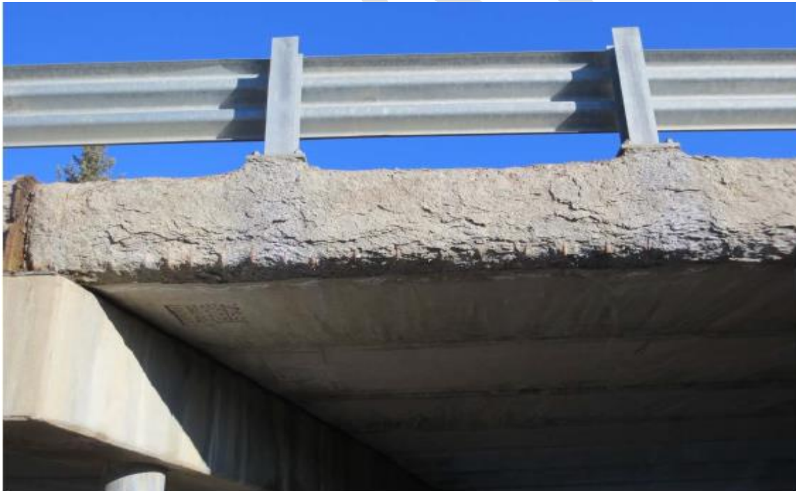
Example 4: Significant section loss on all surfaces extending beneath bridge rail post baseplate. Exposed steel stirrups. Exterior girder rated 2. Bridge rail post rated 2.
