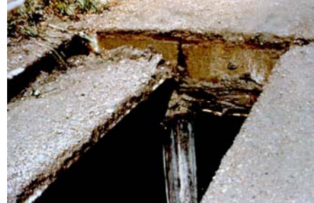
Sheared timber cap. One girder hung up on pile.
