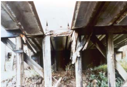
Failed pier cap
