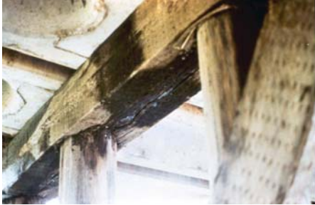
Bottom of cap with piles punching (North pier)
