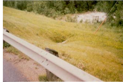
Hole in side slope on d/s side
